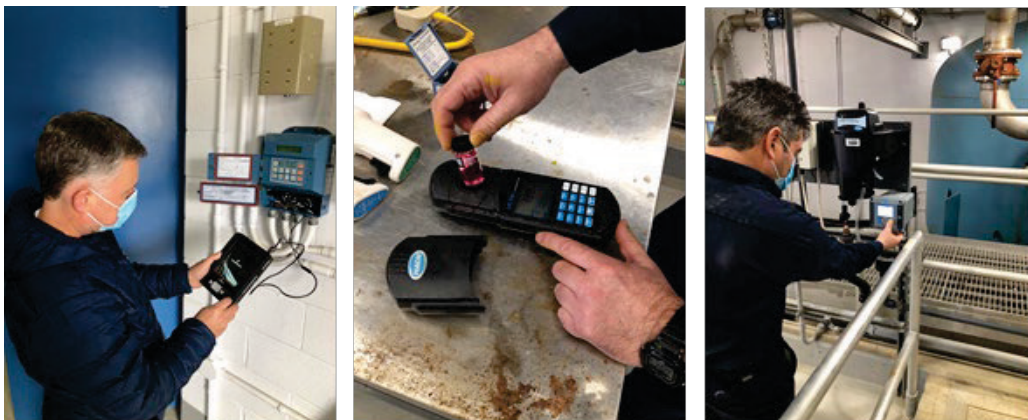
Figure 13. Staff calibrating level transmitter and verifying handheld chlorine analyzer and online turbidity analyzer
