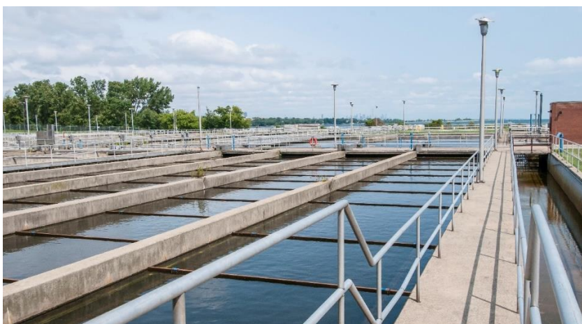
Figure 10. Row of outdoor wastewater secondary clarifier tanks at a Peel Region water resource recovery facility
