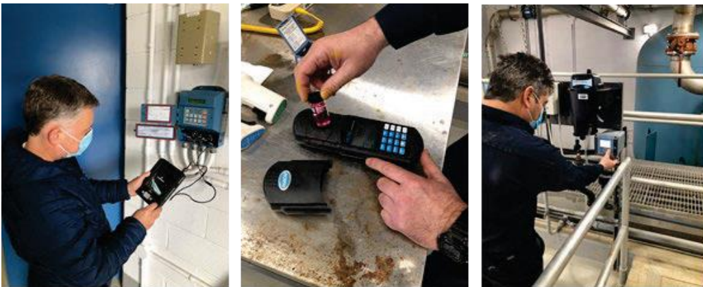
Figure 15. Staff calibrating level transmitter and verifying handheld chlorine analyzer and online turbidity analyzer
