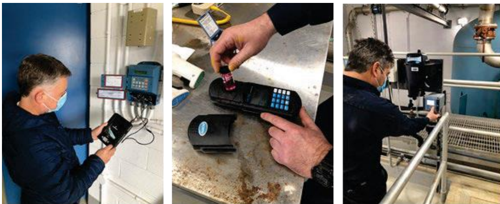
Figure 13. Staff calibrating level transmitter and verifying handheld chlorine analyzer and online turbidity analyzer
