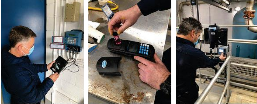
Figure 11. Staff calibrating level transmitter and verifying handheld chlorine analyzer and online turbidity analyzer
