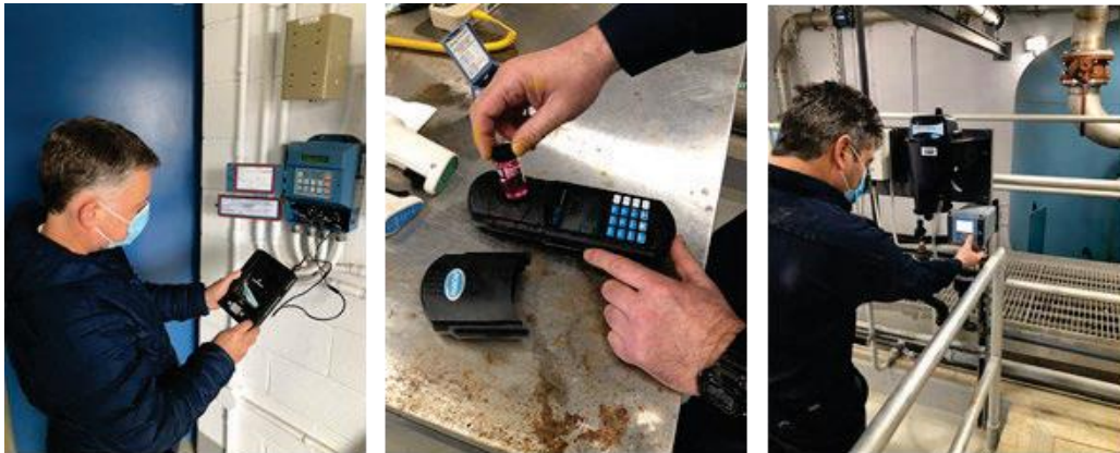
Figure 12. Staff calibrating level transmitter and verifying handheld chlorine analyzer and online turbidity analyzer
