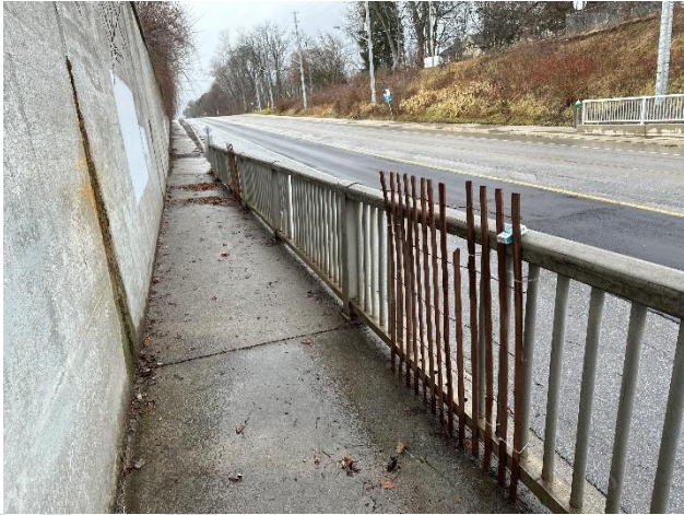
Pedestrian Facilities: Sections of railings are missing on the west side, north of the underpass.
