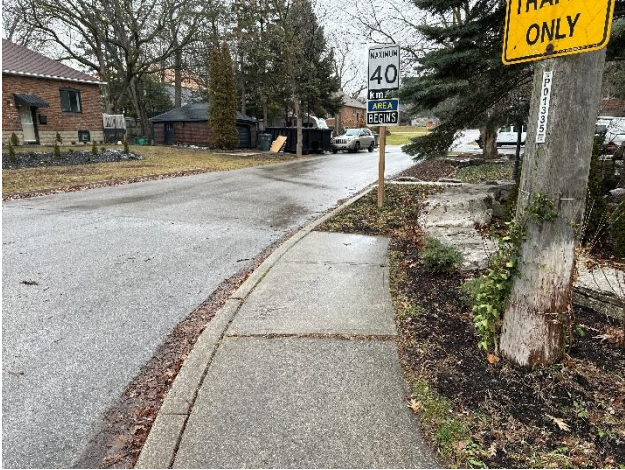
Pedestrian Facilities: Southeast sidewalk ends after the curb return. Photo Location: Southeast corner, looking east
