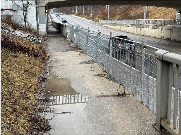
Pedestrian Facilities: West side railing section near the underpass is missing, with some pooling.
