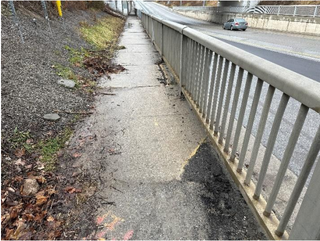
Pedestrian Facilities: Recently patched sidewalk near the railing on the west side.
