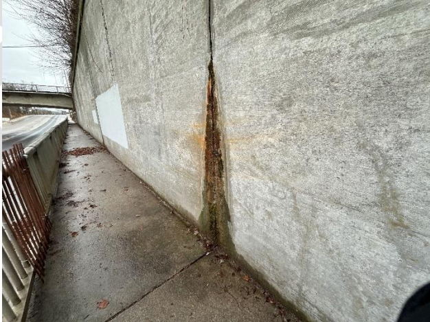
Pedestrian Facilities: Potential water seepage is present in west side retaining wall.
