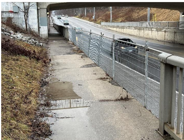
Missing railing sections on the west side of Dixie Road, with multiple instances of pooling
