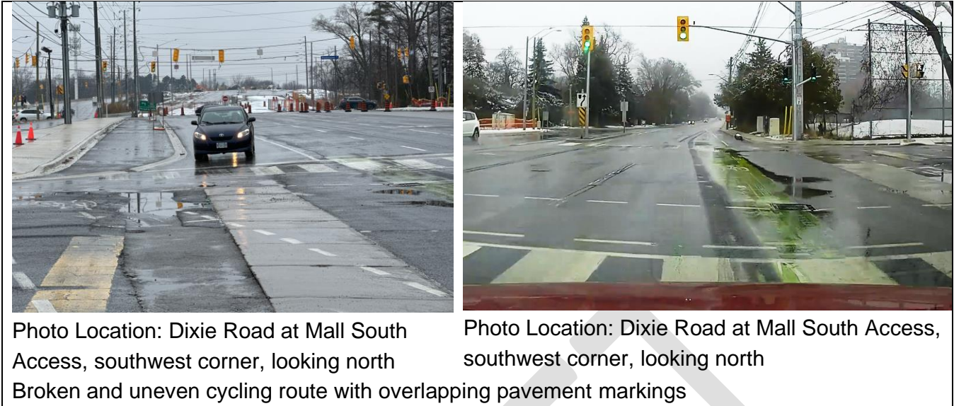
Exhibit 26: Issues with Cyclist Facilities at Dixie Road at Mall South Access
