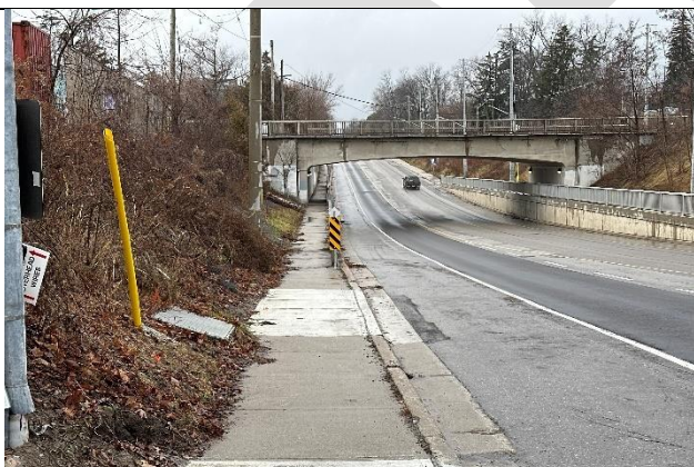
Bicycle lane buffer is missing on both sides between Orchard Hill Road and Lakeview Golf Course Access Photo Location: West side of Dixie Road, approximately 50m from the underpass, looking north
