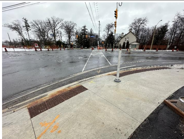
Exhibit 19: Misaligned Tactile Walking Surface Indicators at Rometown Drive
