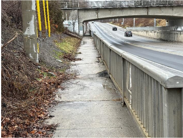
Uneven and damaged sidewalk near the railing on the west side of Dixie Road
