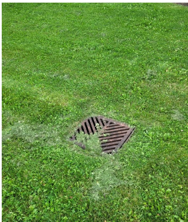
Photo 9. Example of existing property storm sewer disturbance at bottom of built swale.
