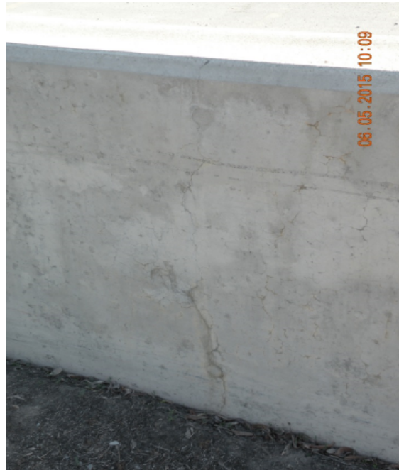
Narrow Crack on Interior Parapet Wall
