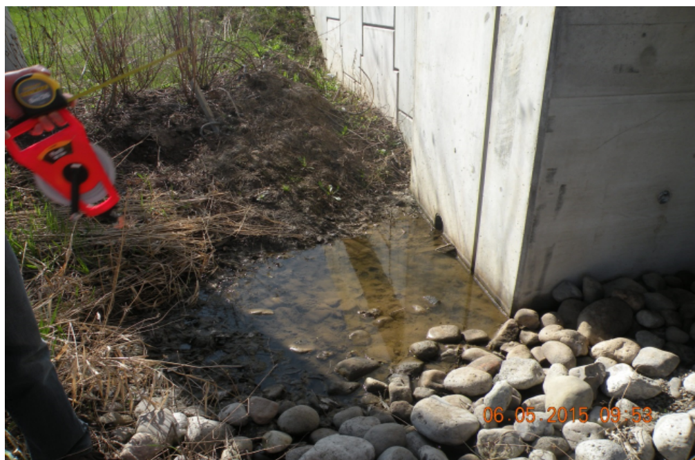
Typical Ponding at Abutment Corners
