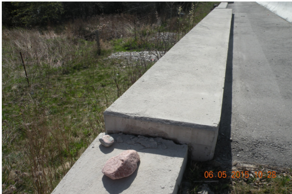
Disintegrated Concrete at RSS Connection
