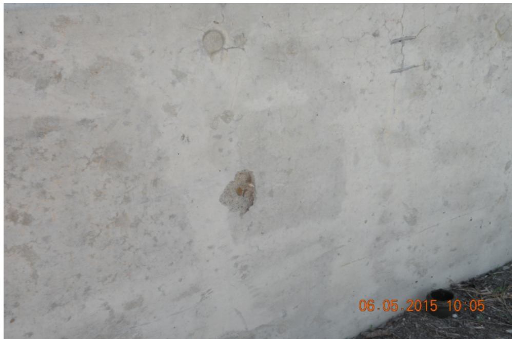
Spall on Interior Parapet Wall
