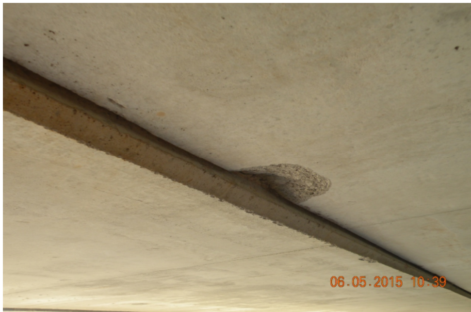
Spall at Second Joint from East End
