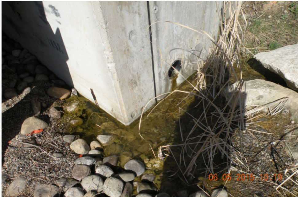
Pounding (Typical on East Side)
