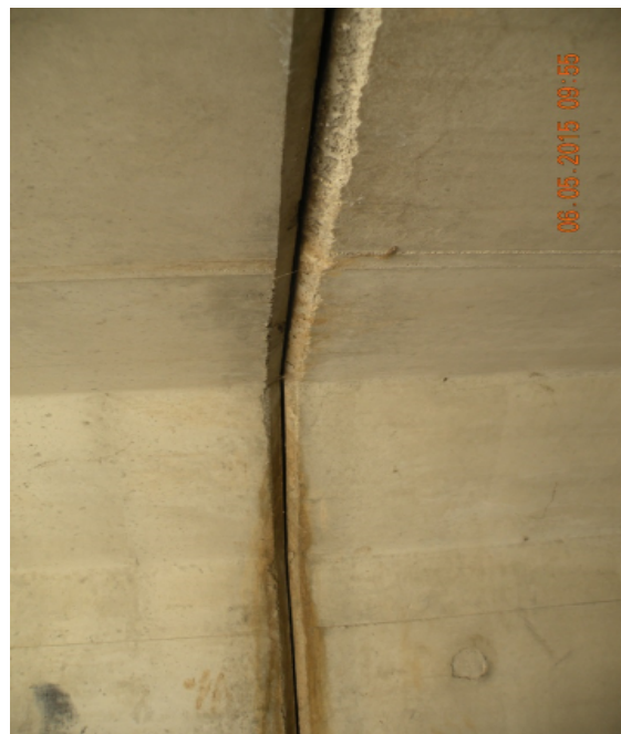
Joint with Staining and Scaling
