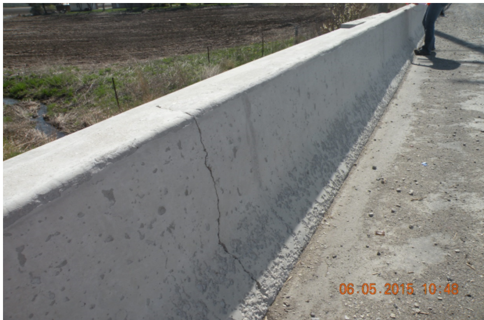
Wide Crack and Scaling on Barrier Wall (typical both sides)
