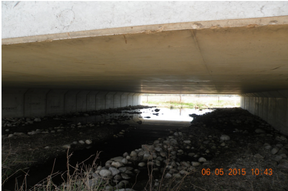
Looking East (Note Scaling on Exterior Soffit)
