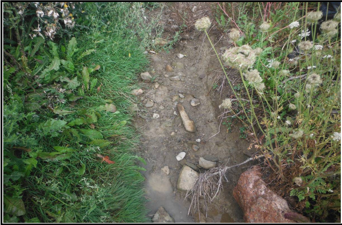
PHOTOGRAPH NO.: 18 - Culvert 10 FROM: In channel on upstream side LOOKING: Channel COMMENT:
