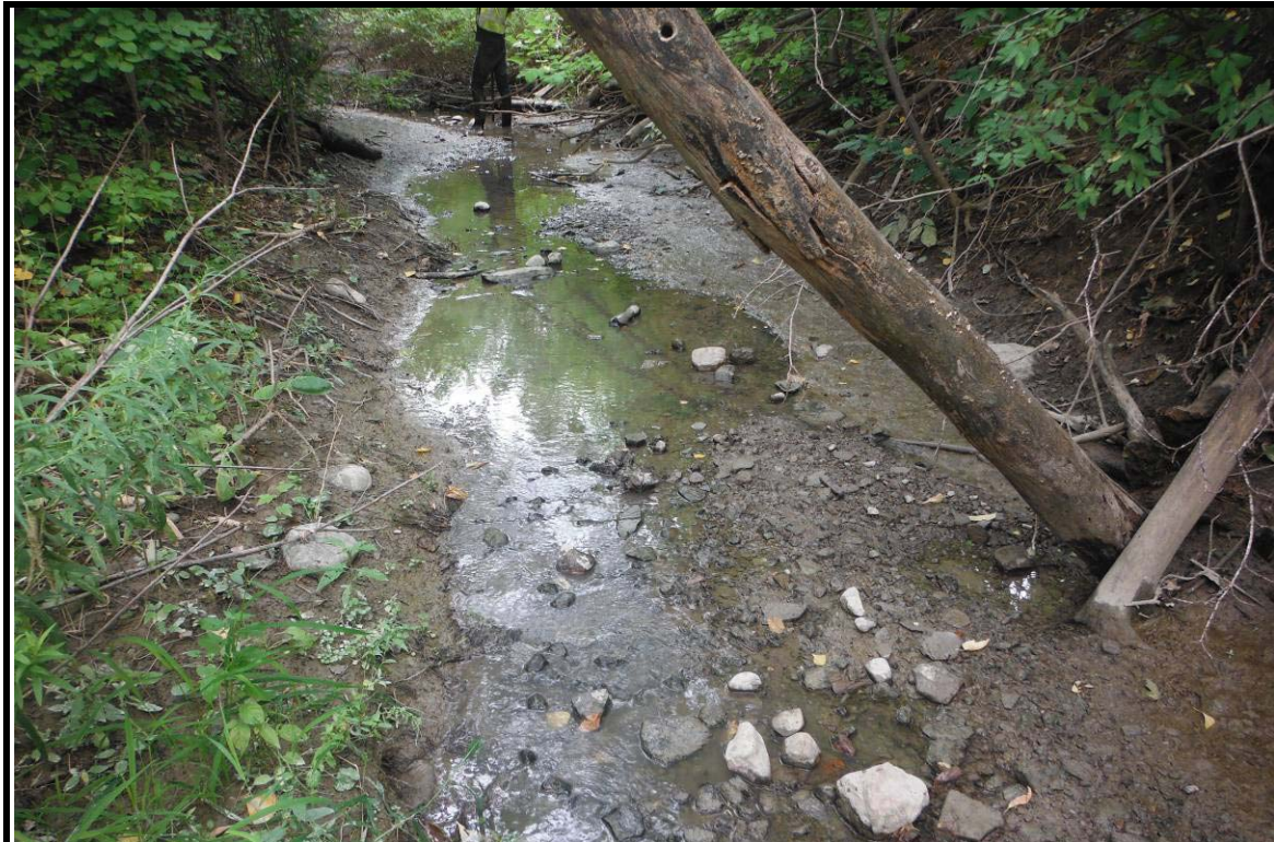
PHOTOGRAPH NO.: 16 - Culvert 10 FROM: In channel on downstream side LOOKING: Upstream COMMENT:
