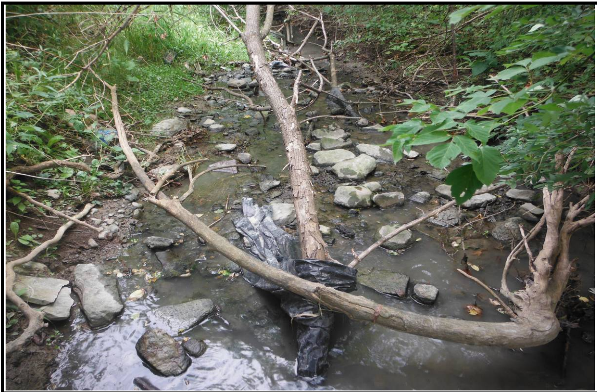
PHOTOGRAPH NO.: 13 - Culvert 10 FROM: In channel on downstream side LOOKING: Downstream COMMENT:
