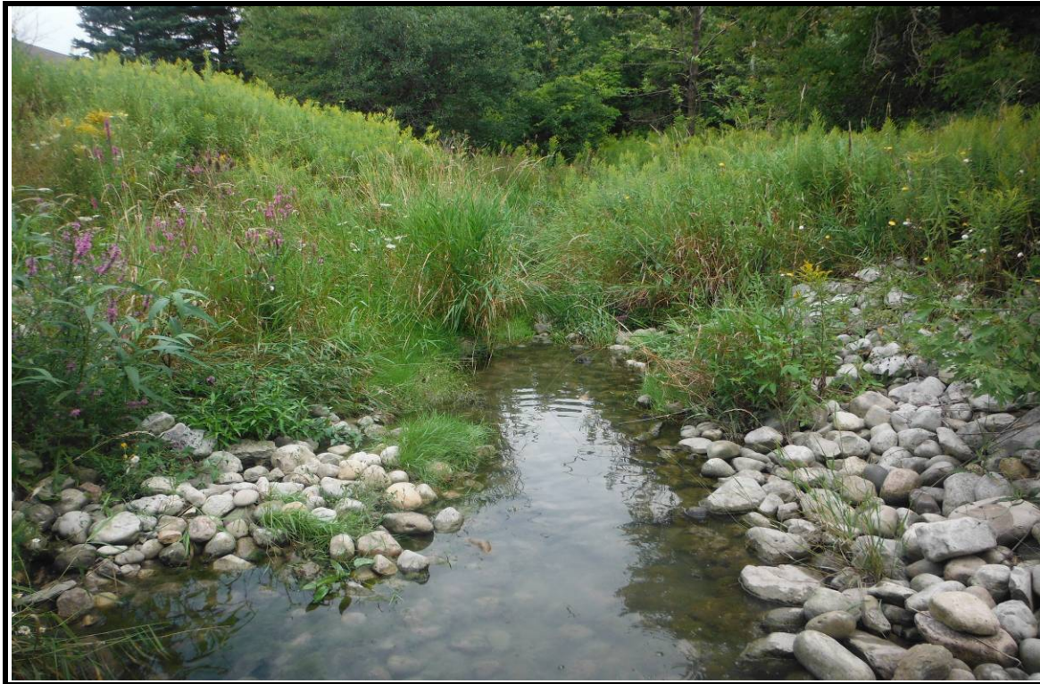
PHOTOGRAPH NO.: 14 - Culvert 10 FROM: In channel on downstream side LOOKING: Downstream COMMENT:
