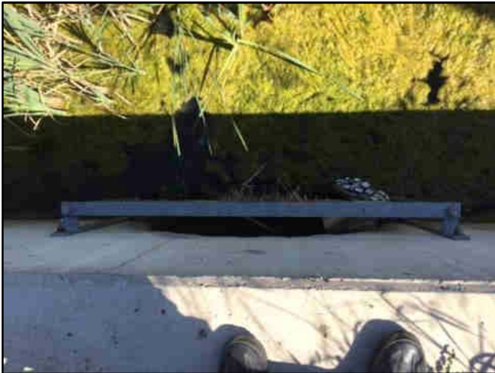
Photo 16. Drainage Feature #6 – Standing Water at Culvert Outlet
