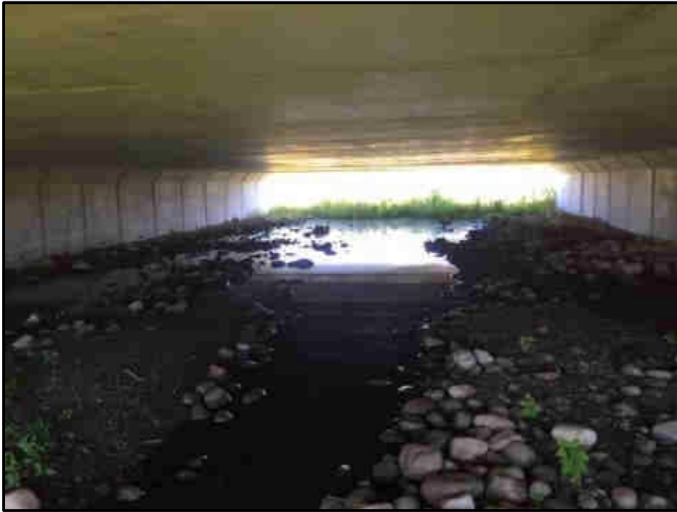
Photo 13. Levi Creek North – Standing Water within Culvert Looking West
