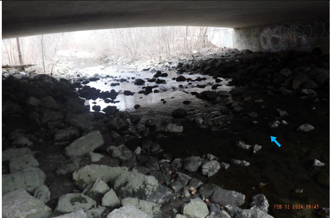
The channel was historically reinforced with riprap within and downstream of the Kirwin Drive stream crossing.
