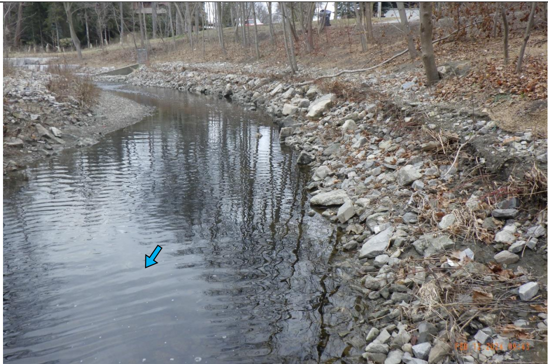
Sections of the treatment were in poor condition. For example, riprap had become detached and displaced in-channel. Till exposure was also documented along the channel bed.
