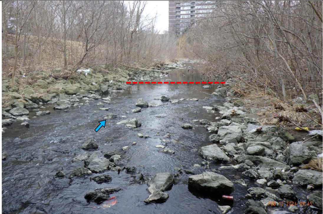
The riprap treatment extended downstream of Kirwin Drive. The treatment was in moderately stable condition. There was limited evidence of scouring and channel banks were well vegetated. The approximate proposed sewer crossing is delineated in red.
