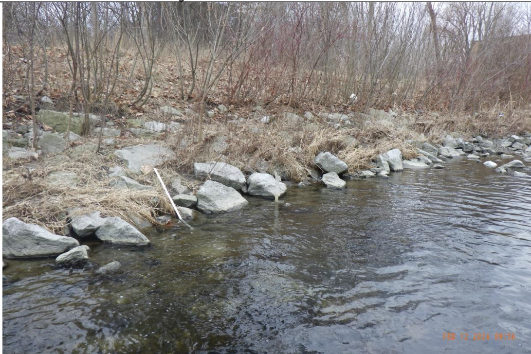
Channel banks were vegetated and protected with riprap. The treatment was in good condition at the time of assessment.
