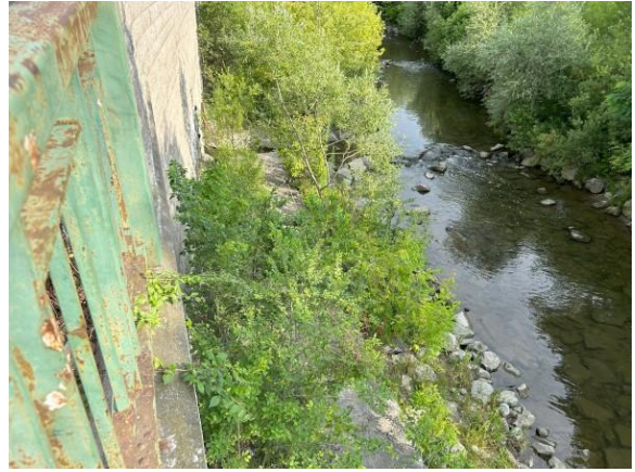
Photo 10: Cooksville Creek west bank wall at Jaguar.
