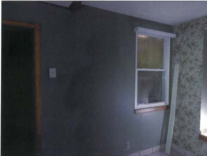
Plate 48: View of new structural opening and window located on the southern elevation of the rear addition..
