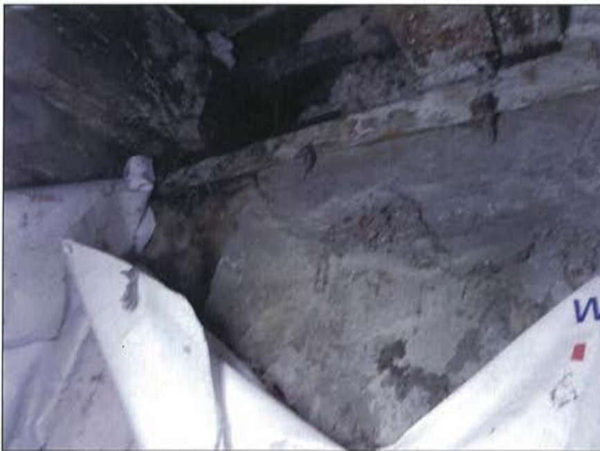
Plate 65: Detail of original sill plate sitting on top of parged concrete which conceals original stone foundations.
