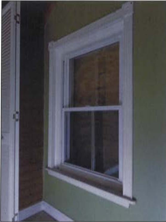
Plate 58: View of original structural opening and new window on south wall (east half).
