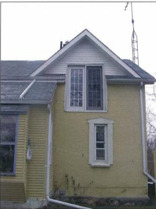
Plate 18: View of addition and alteration, showing gabled dormer and sliding, glass door.
