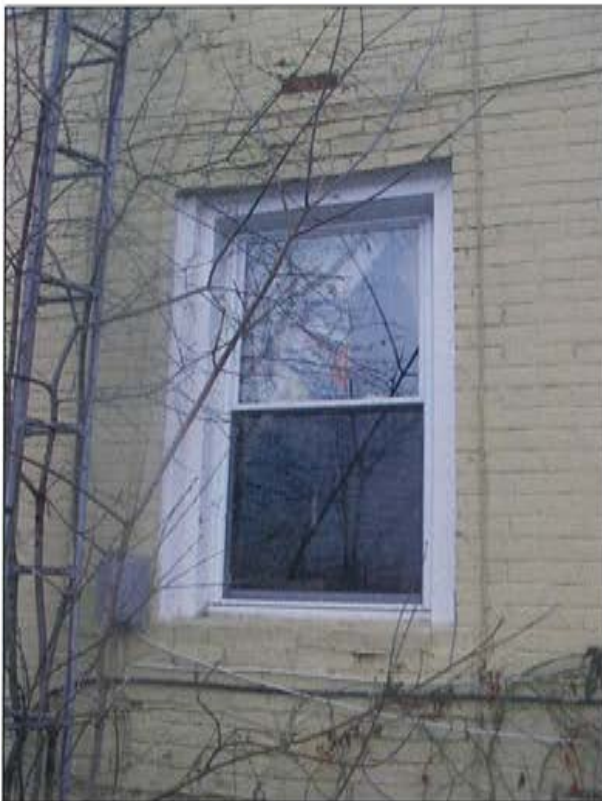
Plate 23: Ground floor window on southern elevation, lacking original voussoirs and sill.
