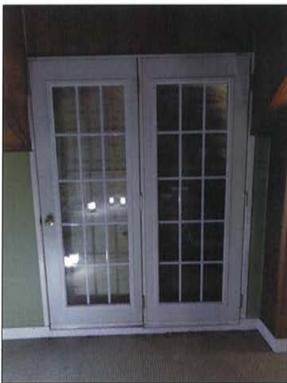
Plate 61: New French doors added on the west wall (south half) in the upper storey.
