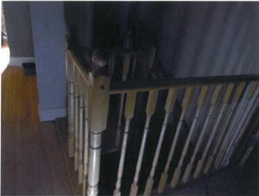
Plate 44: Location context of spiral staircase behind original central staircase, showing railing and balusters. This staircase is a recent addition.
