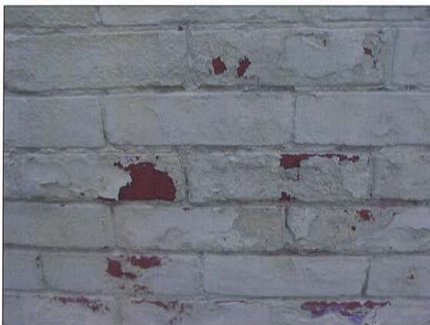
Plate 4: Peeling paint on eastern elevation, exposing original red brickwork
