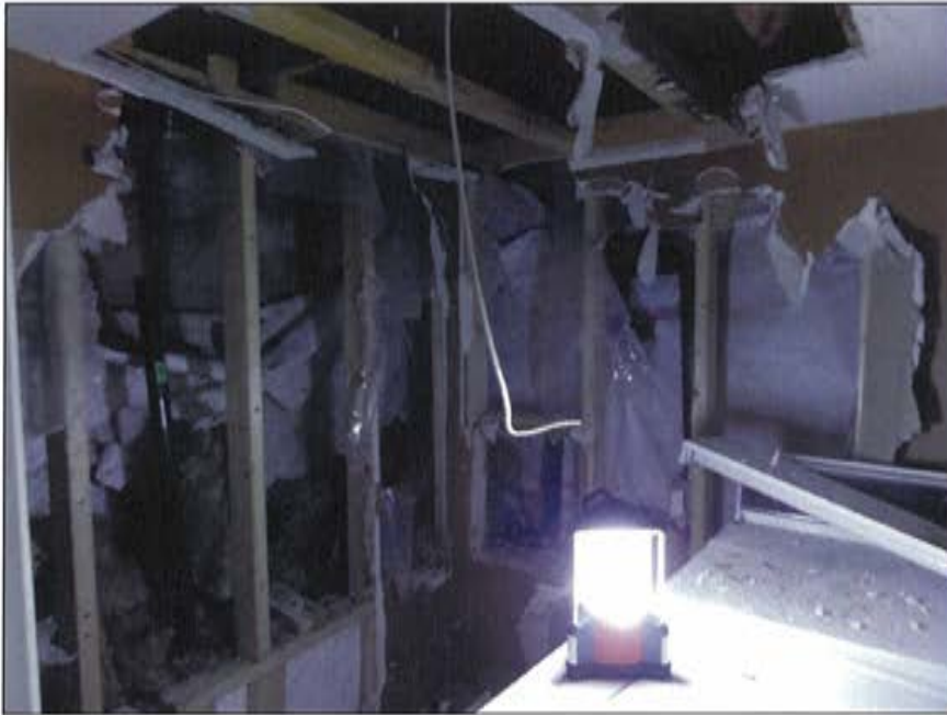
Plate 64: View of Area 3 (laundry room) showing removed drywall, wall studs, and concrete parging in background.
