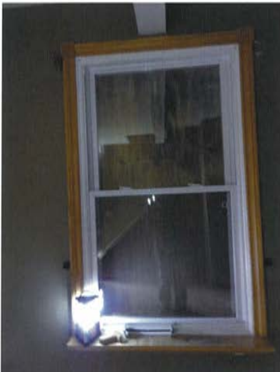
Plate 53: View of original structural opening on south wall of Family Room showing new window, trim and sill.
