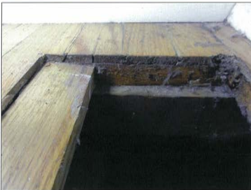
Plate 39: Cross section of flooring in Living Room showing extant narrow floor boards on top of older flooring.
