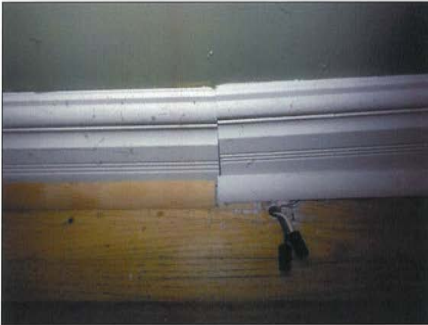
Plate 36: Detail of baseboards in Living Room showing example of typical new baseboards that have been installed in the house.
