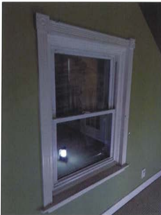
Plate 59: View of original structural opening and new window on south wall (west half).
