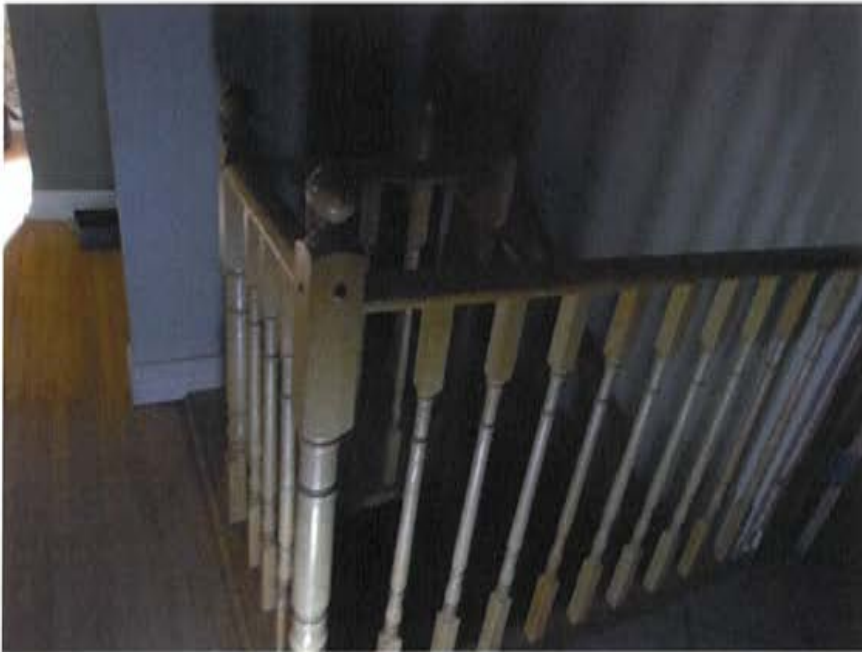
Plate 44: Location context of spiral staircase behind original central staircase, showing railing and balusters. This staircase is a recent addition.
