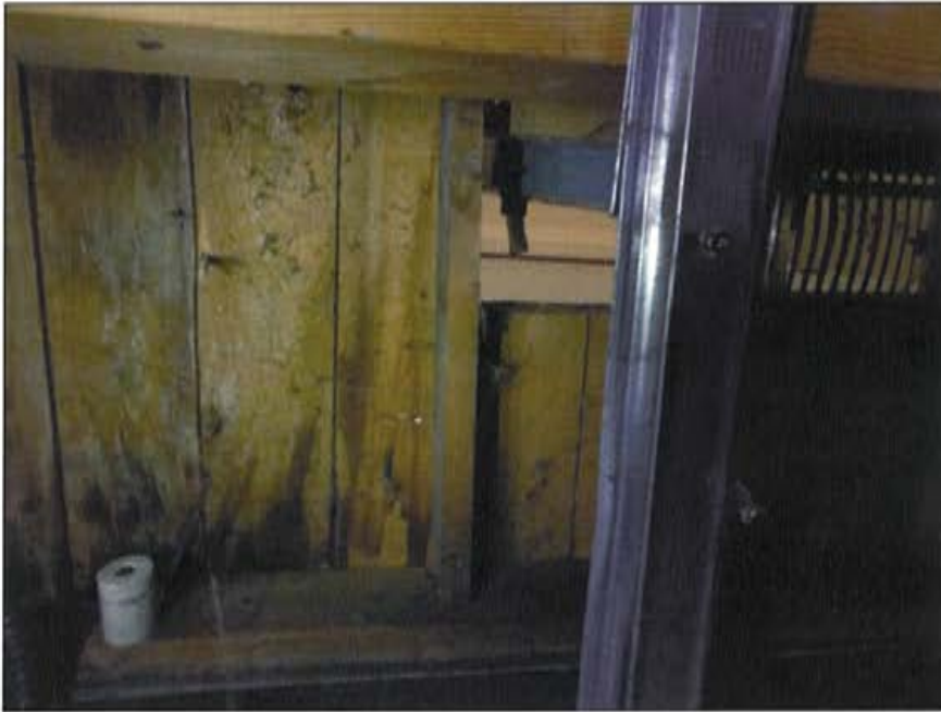
Plate 40: View from basement of location illustrated in Plate 39 showing floor joists, subfloor and hardwood boards on top of the subfloor, running in a direction opposite to the extant narrow hard wood flooring found in the Living Room.
