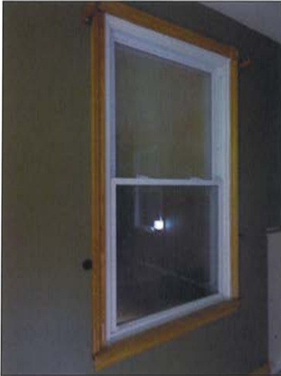
Plate 52: View of original structural opening on east wall of Family Room showing new window, trim and sill.
