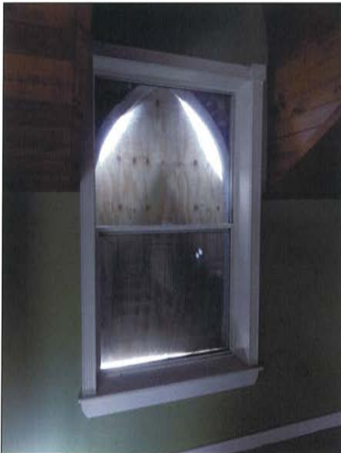
Plate 57: View of pointed window on east wall showing rectangular window and pointed structural opening.
