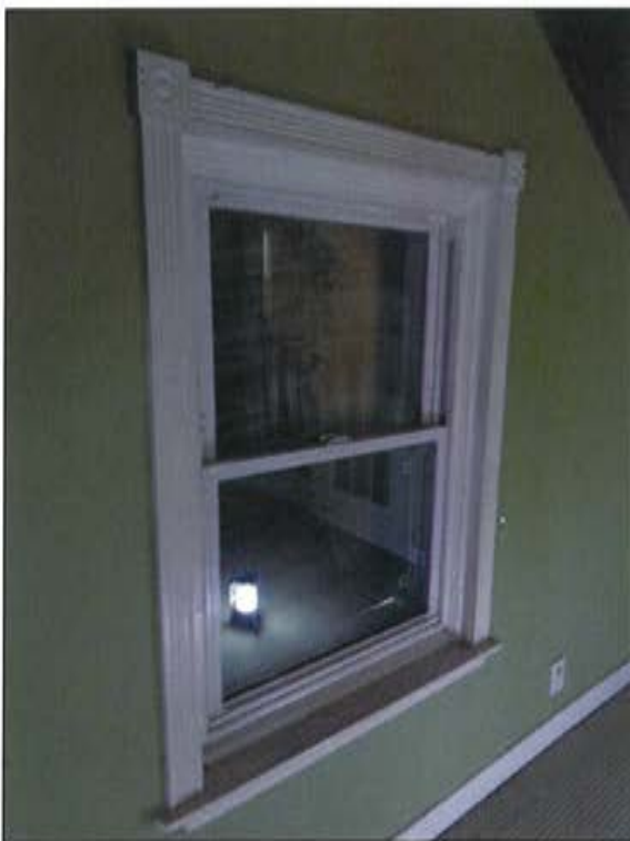
Plate 59: View of original structural opening and new window on south wall (west half).
