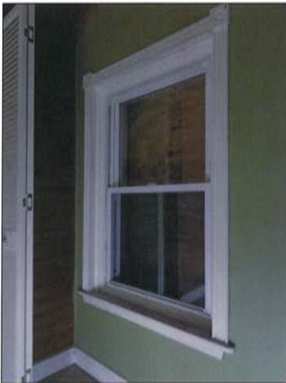
Plate 58: View of original structural opening and new window on south wall (east half).
