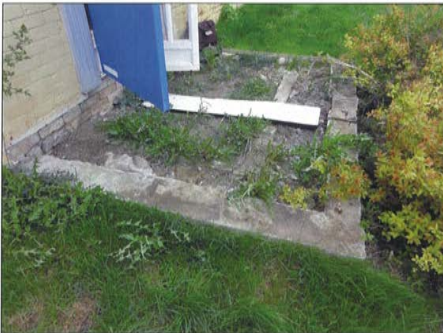
Plate 31: Detail of primary entrance to residence in May 2011 showing location of previous wooden deck and detail of poured concrete base.
