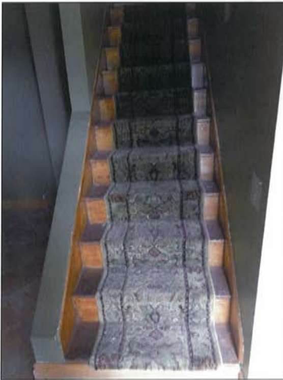
Plate 54: View of central staircase on first floor showing removed partition wall (left) and overall arrangement and materials.
