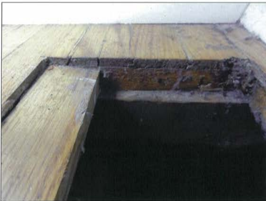
Plate 39: Cross section of flooring in Living Room showing extant narrow floor boards on top of older flooring.
