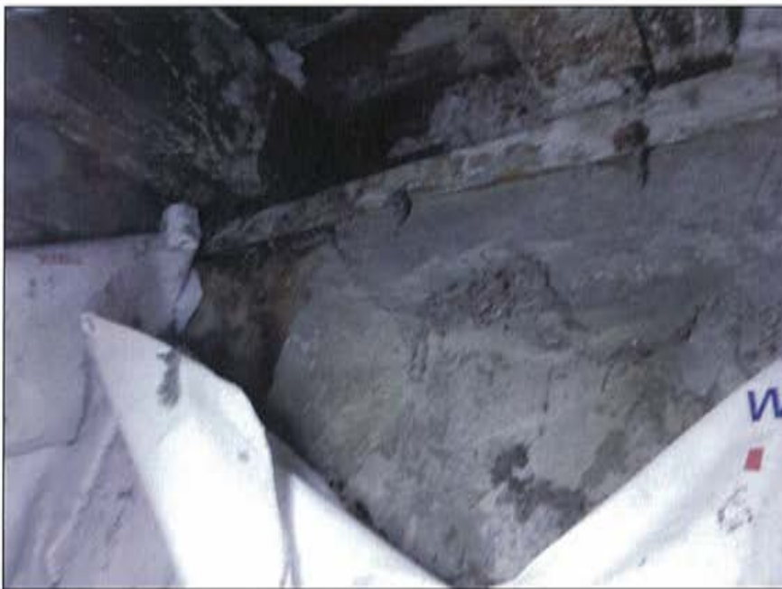
Plate 65: Detail of original sill plate sitting on top of parged concrete which conceals original stone foundations.
