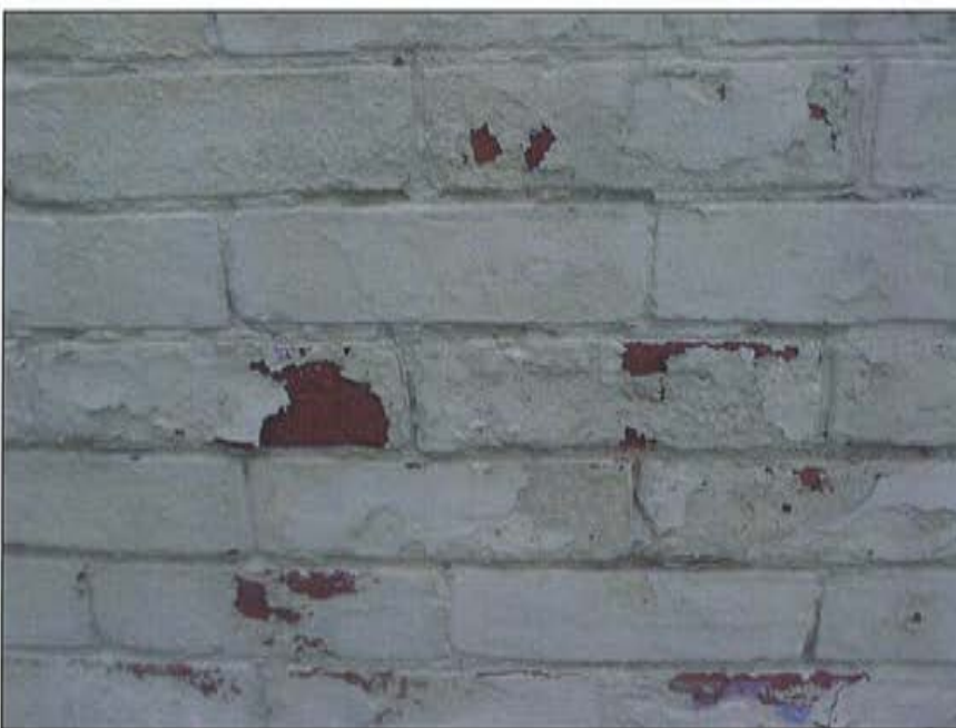
Plate 4: Peeling paint on eastern elevation, exposing original red brickwork
