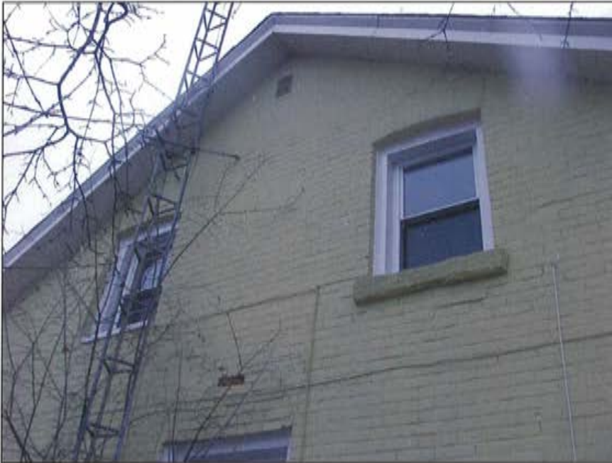
Plate 22: View of upper storey windows on southern elevation, showing new windows and retention of original structural opening and brick voussoirs in the upper storey.
