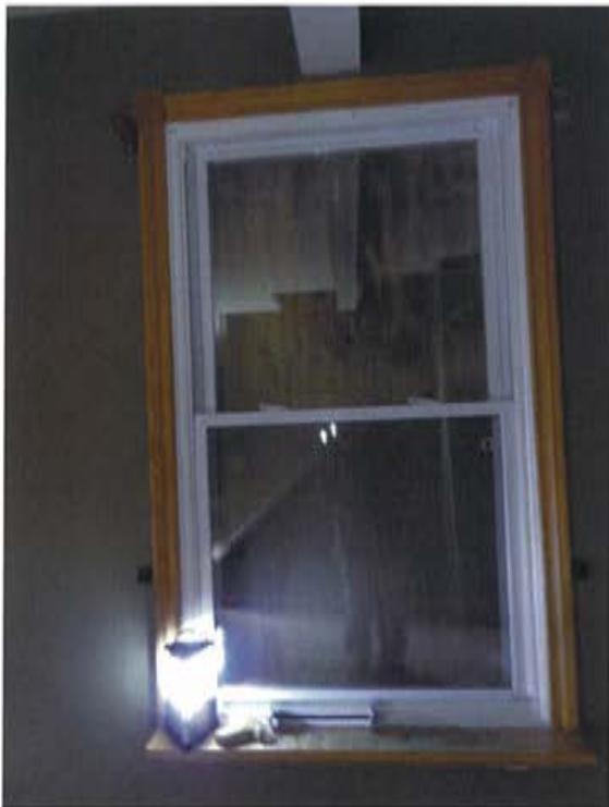
Plate 53: View of original structural opening on south wall of Family Room showing new window, trim and sill.
