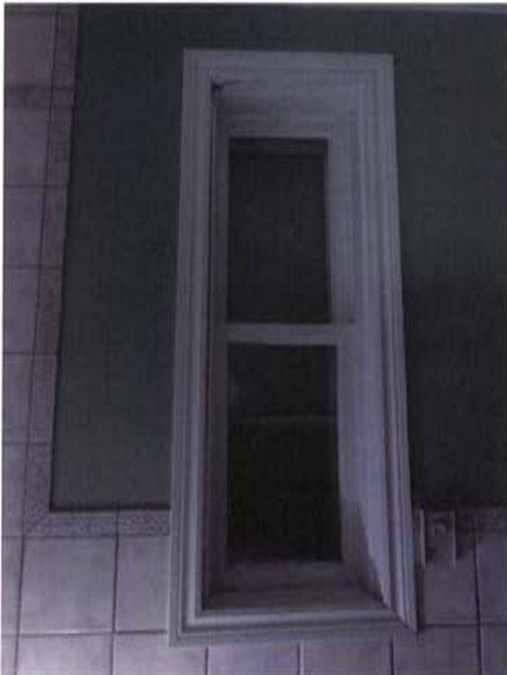
Plate 47: View of window in bathroom showing wooden sashes and older wooden trim.
