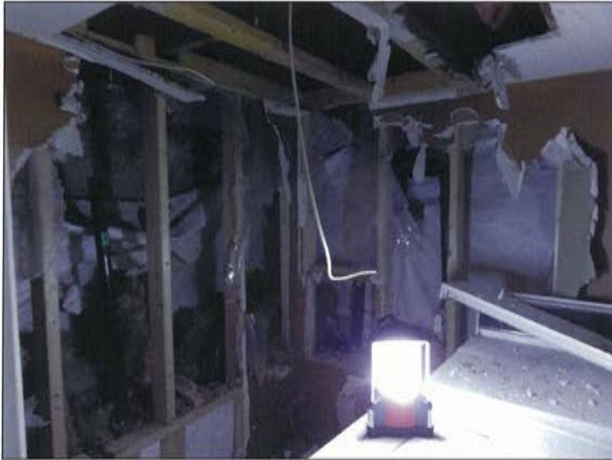
Plate 64: View of Area 3 (laundry room) showing removed drywall, wall studs, and concrete parging in background.
