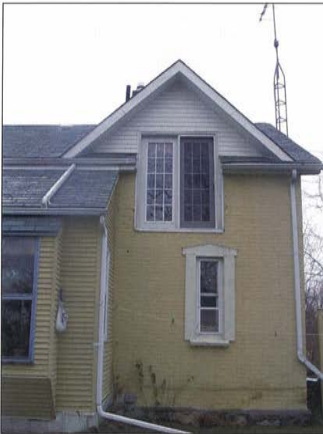
Plate 18: View of addition and alteration, showing gabled dormer and sliding, glass door.
