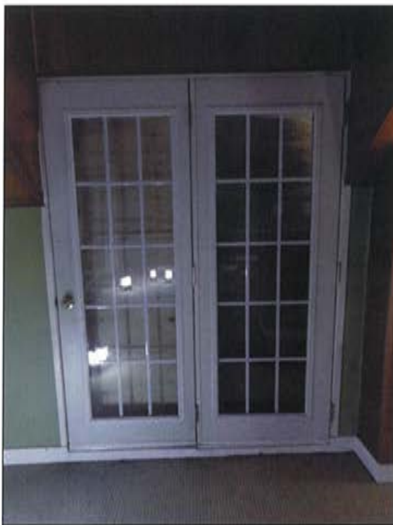
Plate 61: New French doors added on the west wall (south half) in the upper storey.
