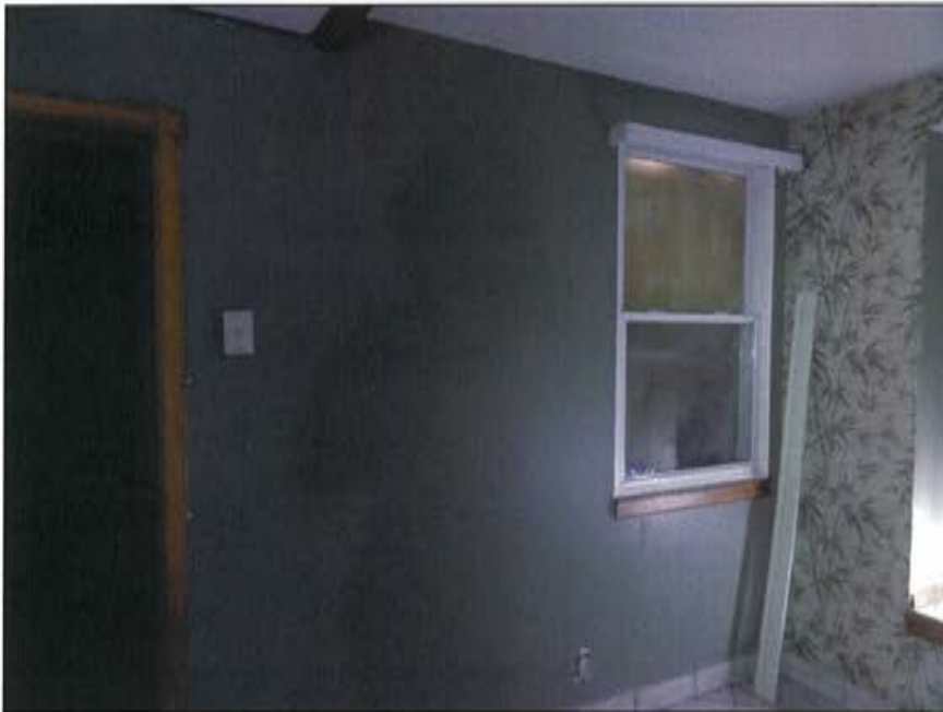
Plate 48: View of new structural opening and window located on the southern elevation of the rear addition..
