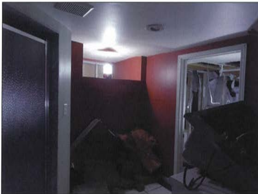
Plate 63: View of Area 2 (bathroom) showing shower in foreground and Area 3 in background.
