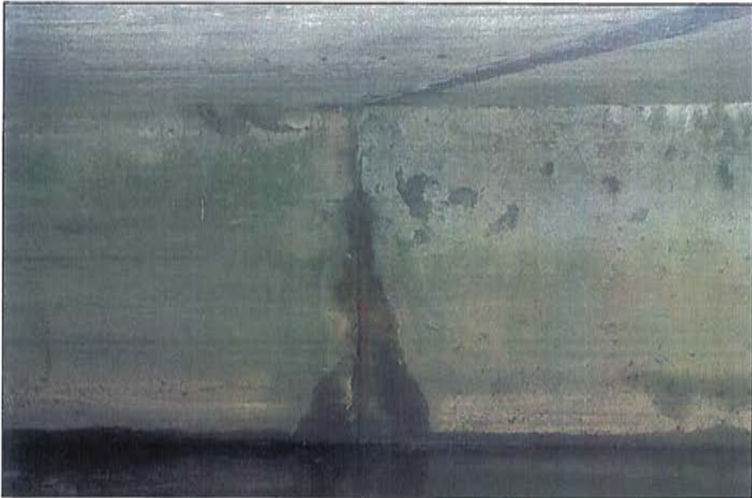
Photo 17: West wall, south construction joint: birds' nests.
