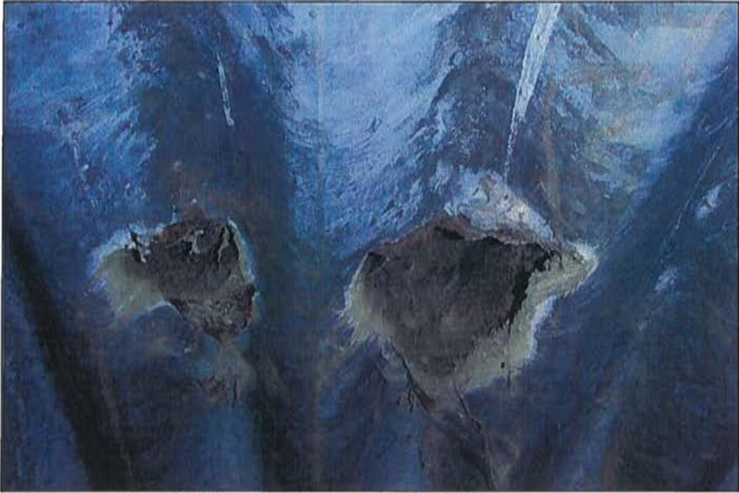
Photo 5: Top of CSPA, near inlet: 0.1 m diameter holes.
