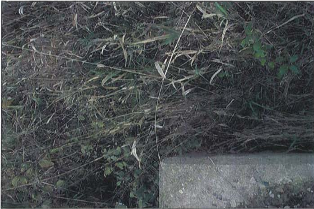
Photo 9: Embankment erosion, east approach, north side.
