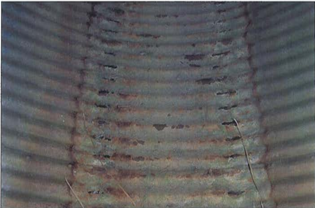
Photo 6: Floor at inlet end: corroded through.
