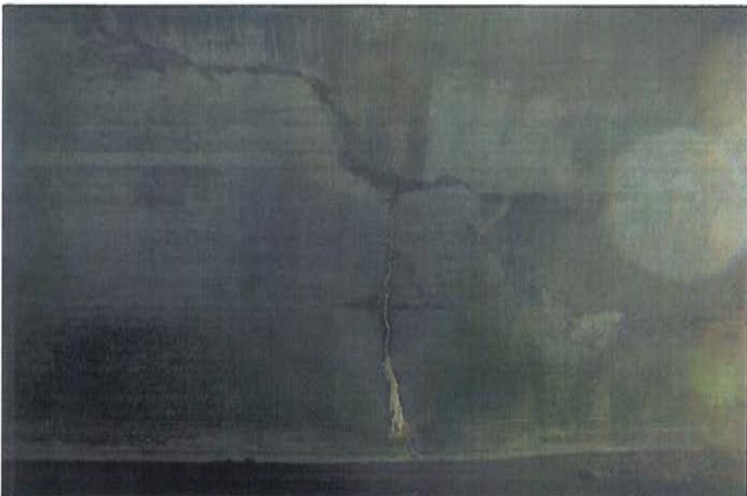
Photo 14: West wall: stained medium vertical crack.
