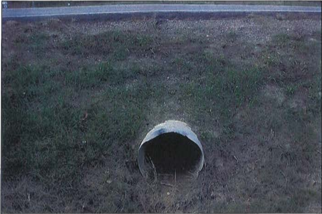
Photo 1: 12+787, outlet end, looking north: perched.
