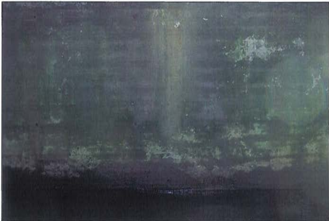
Photo 15: East wall: erosion.
