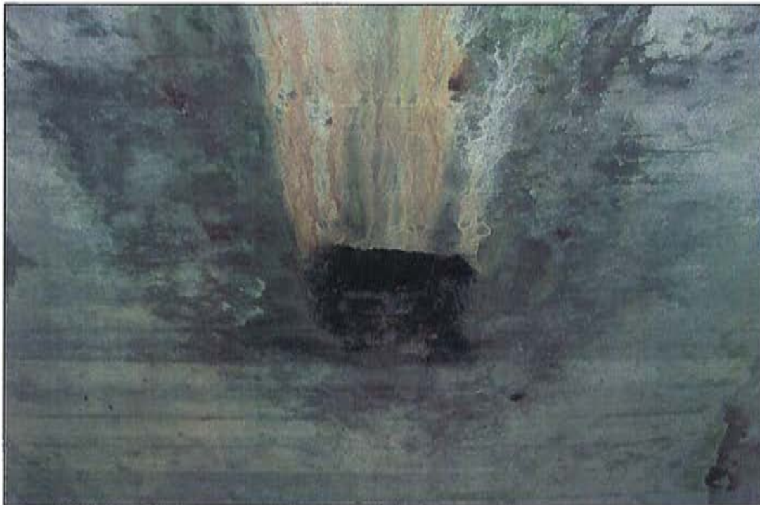
Photo 17: Underside of arch: stained hole and exposed rebar.
