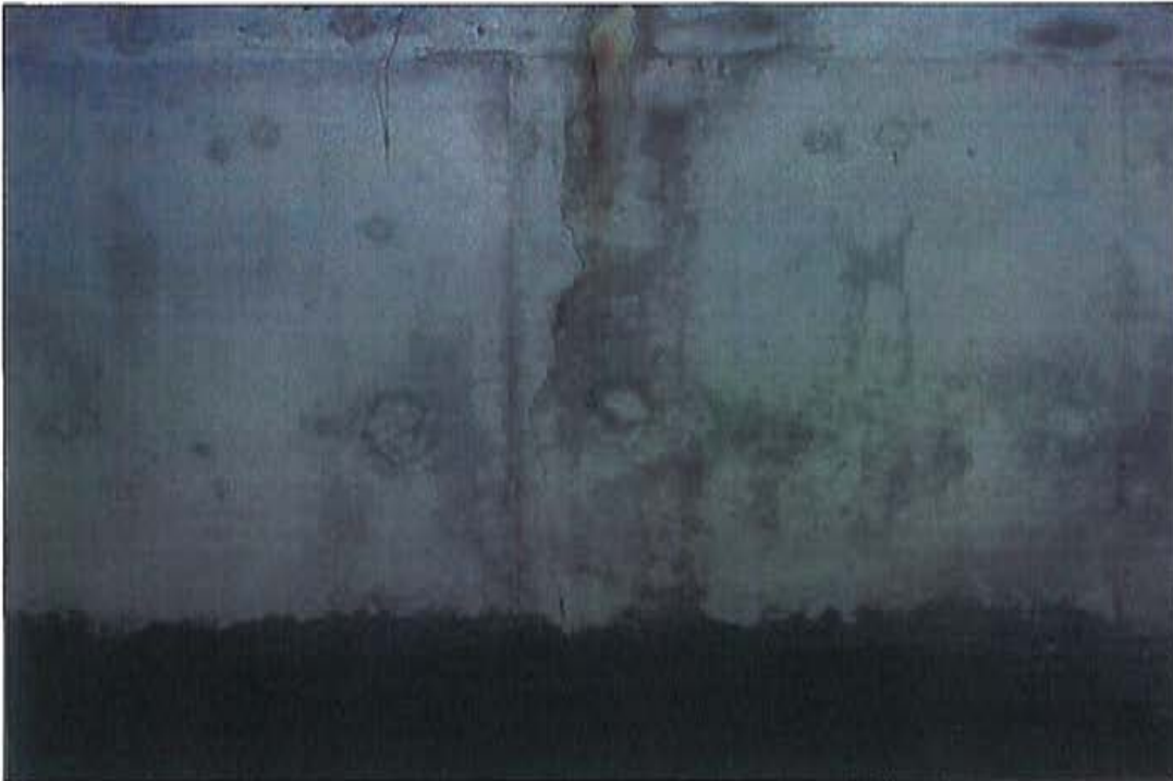
Photo 15: East wall: wide vertical crack.
