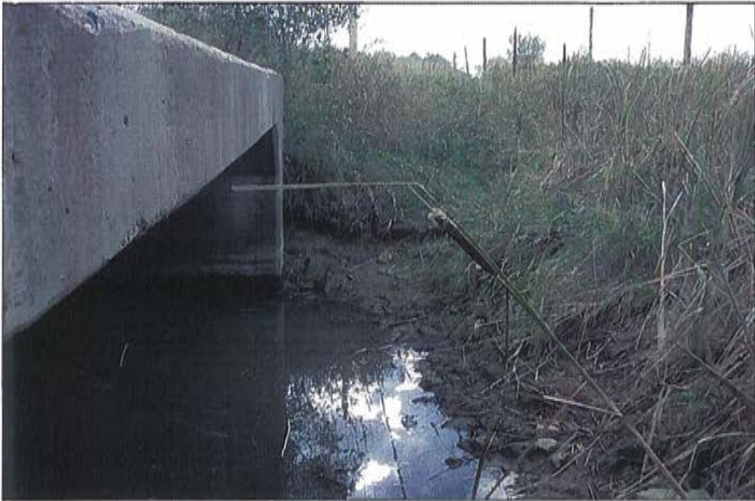
Photo 11: Embankment erosion, west approach, north side.
