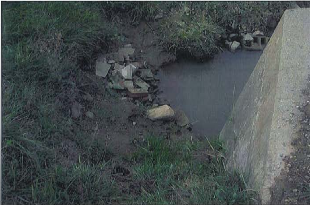
Photo 10: Embankment erosion, west approach, north side.
