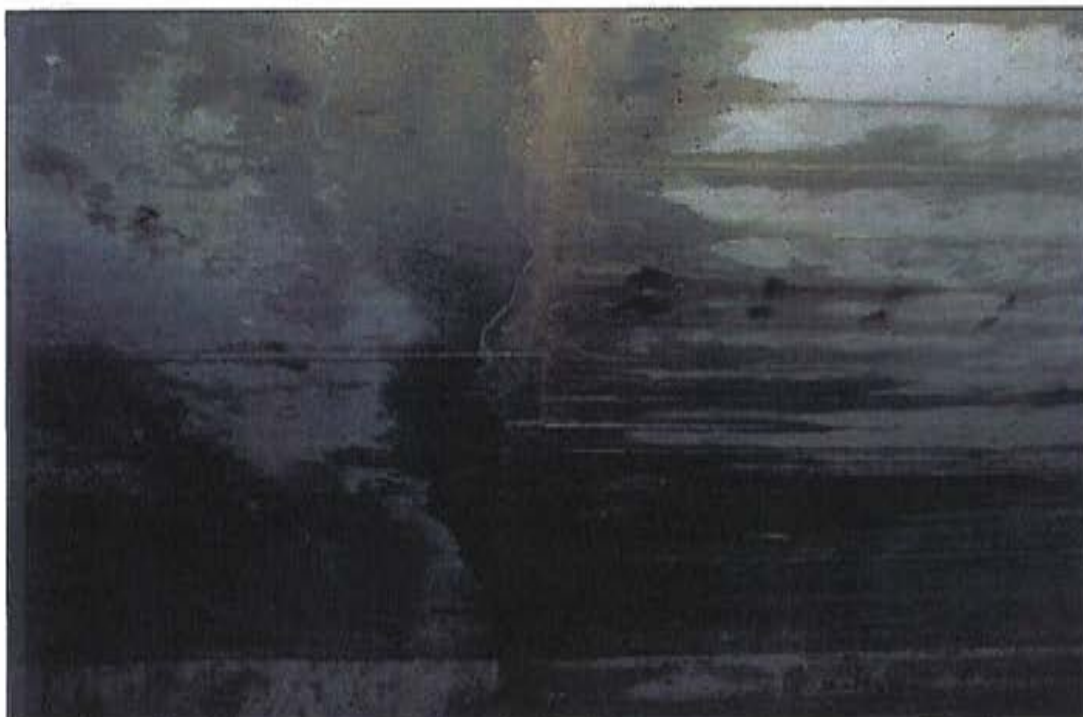
Photo 18: Underside of culvert barrel, looking west: wet area and holes in the slab.
