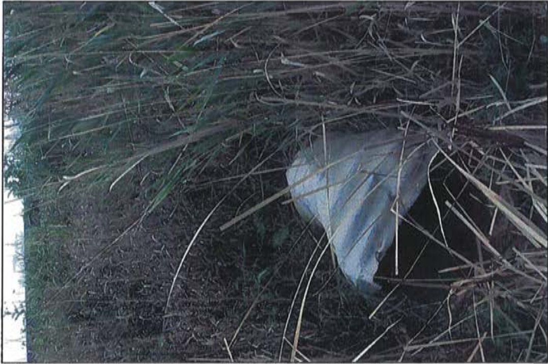
Photo 3: Inlet end, looking south: impact damage; blocked by vegetation.
