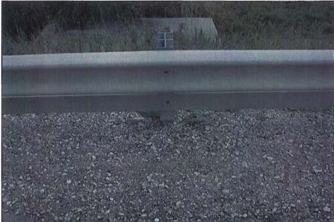
Photo 11: Steel beam guide rail with channel, north and south sides.
