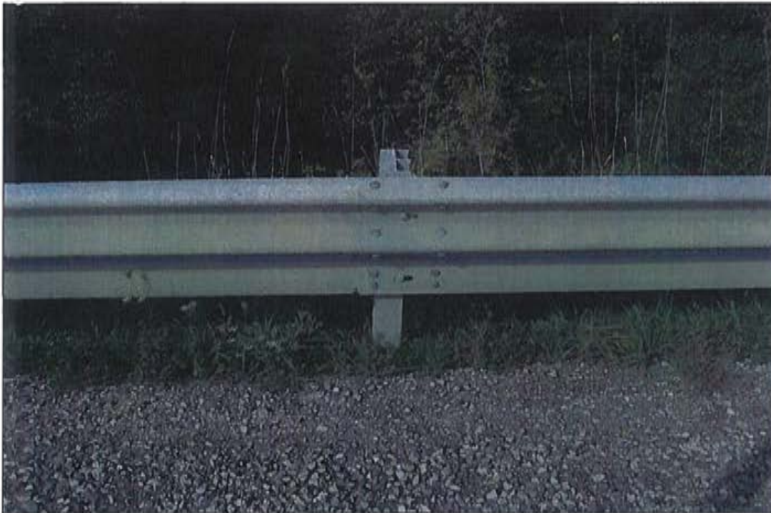
Photo 7: Steel beam guide rail, north and south sides, channel and steel post.
