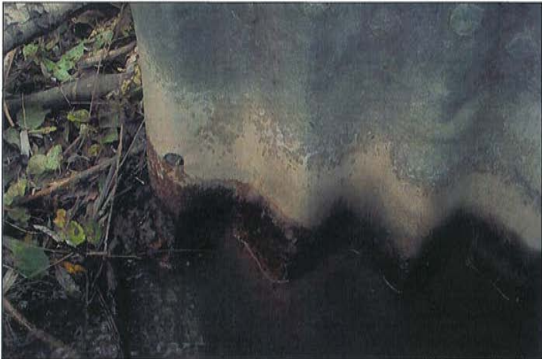
Photo 6: Corrosion through CSPA at inlet, east wall.
