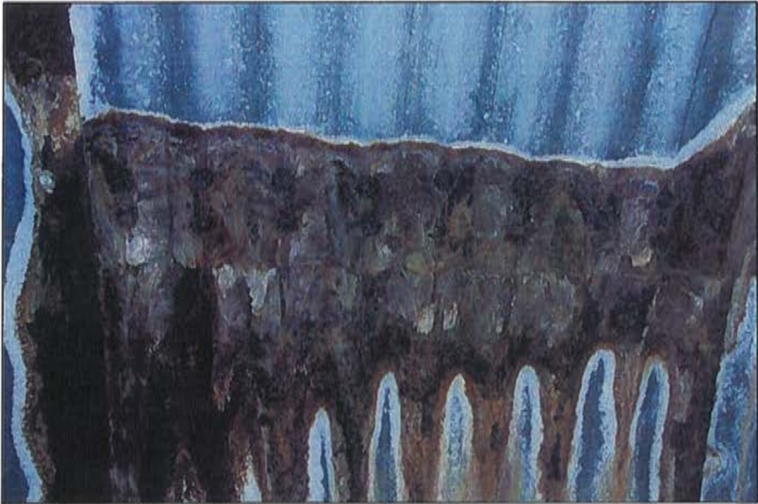
Photo 3: Outlet, east wall: severe corrosion of plate.
