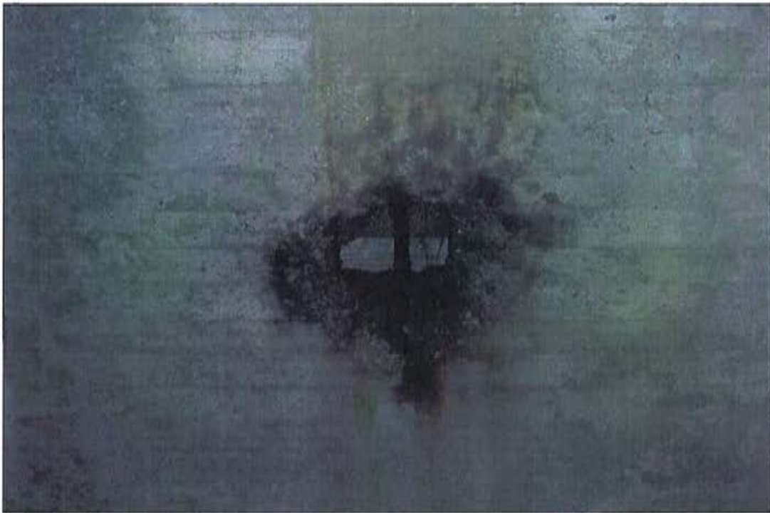
Photo 15: Underside of arch: hole.
