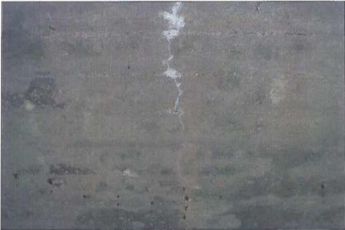
Photo 27: Underside of deck: stained medium longitudinal crack.
