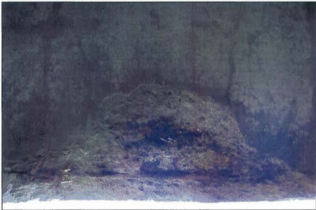
Photo 16: Slab at outlet: spall.
