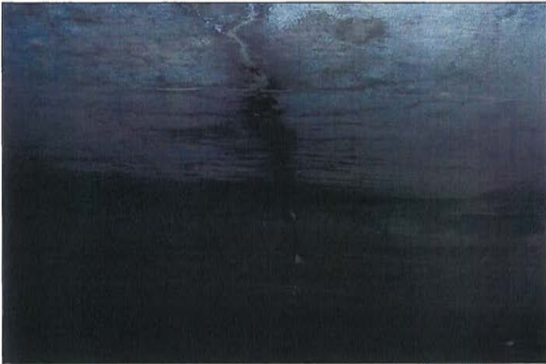
Photo 13: West wall and slab: medium stained crack.
