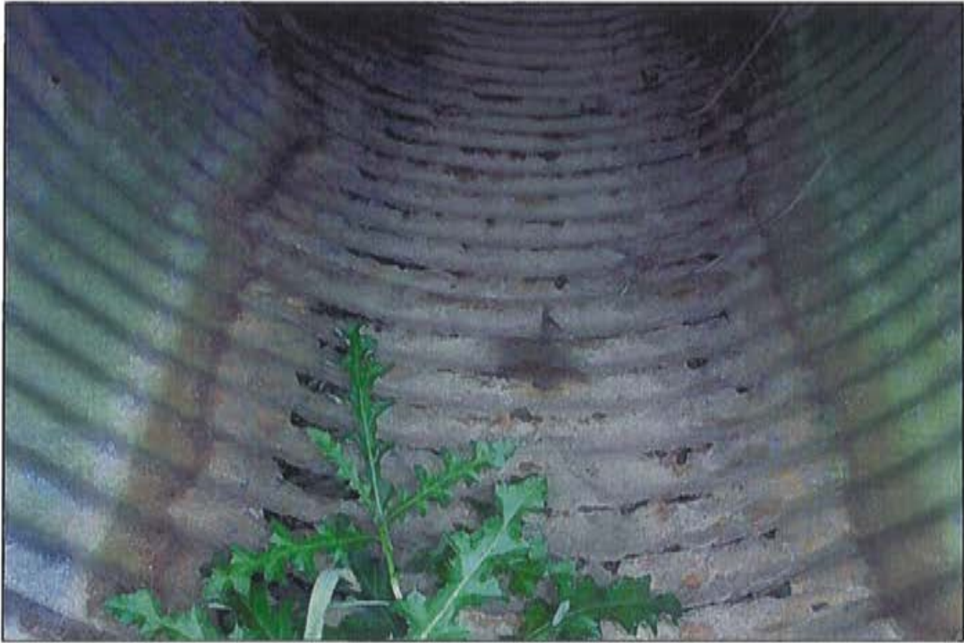
Photo 5: Inlet end: severe corrosion of bottom of CSP.
