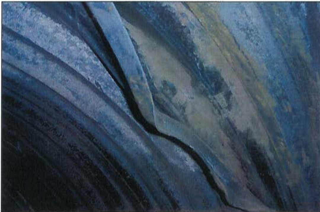
Photo 4: Outlet, west wall: deformation 4.88 north of outlet.
