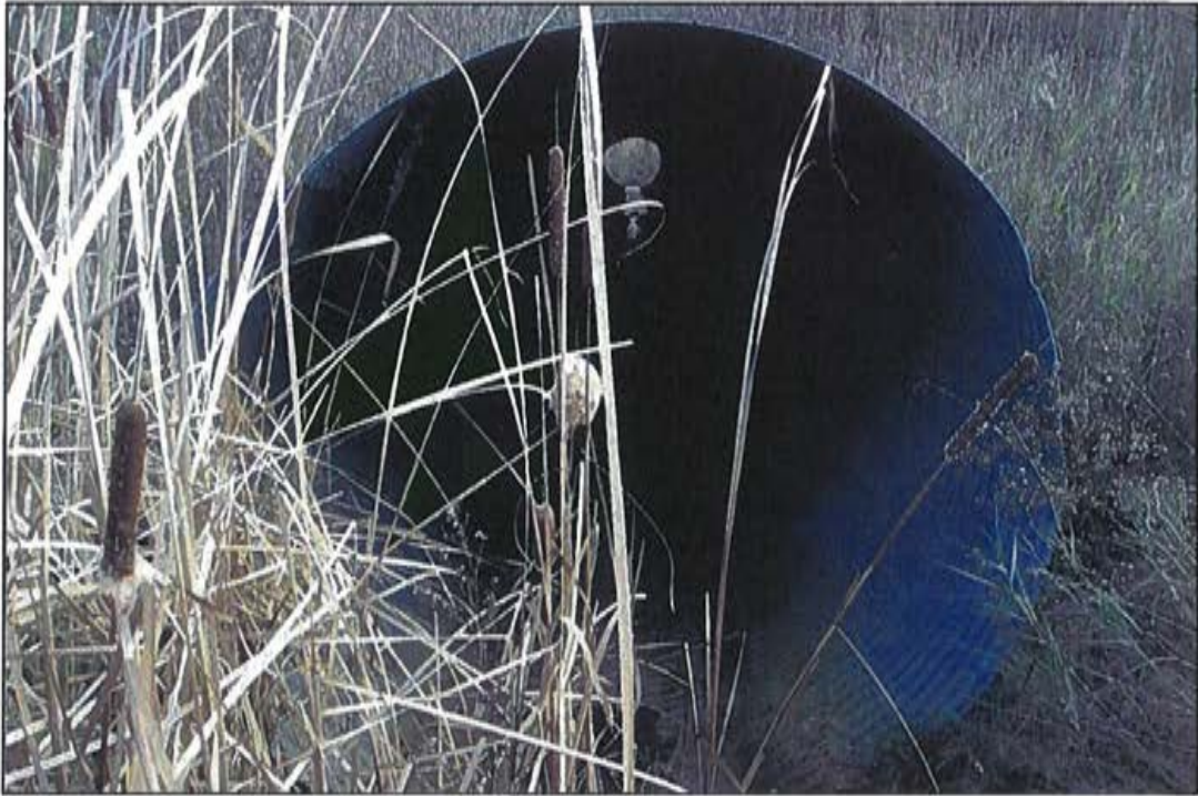
Photo 5: Inlet end, looking south: perched.
