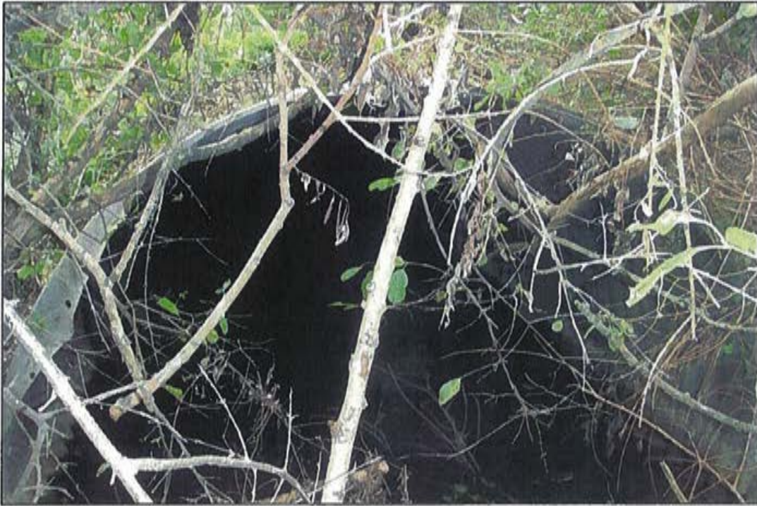
Photo 3: Inlet: blocked by debris.
