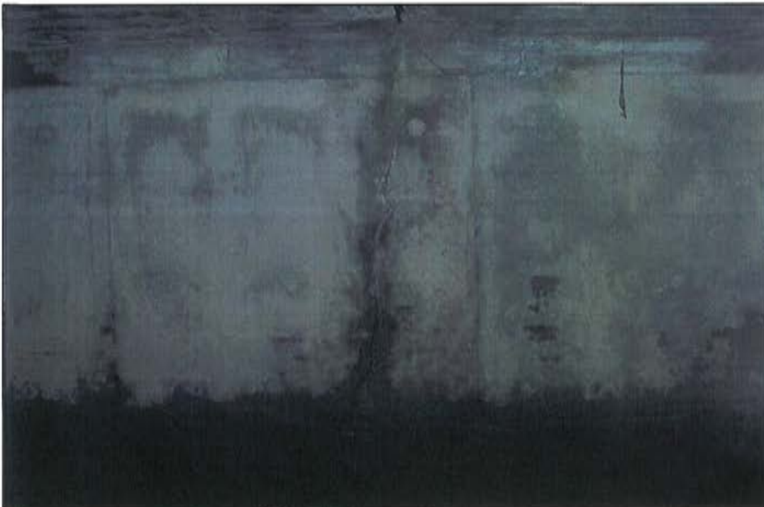
Photo 16: West wall: wide vertical crack.
