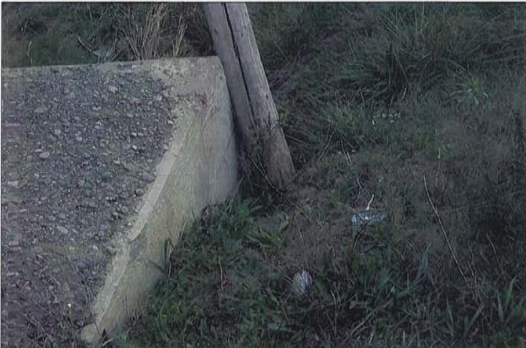
Photo 14: Embankment erosion, west approach, south side.
