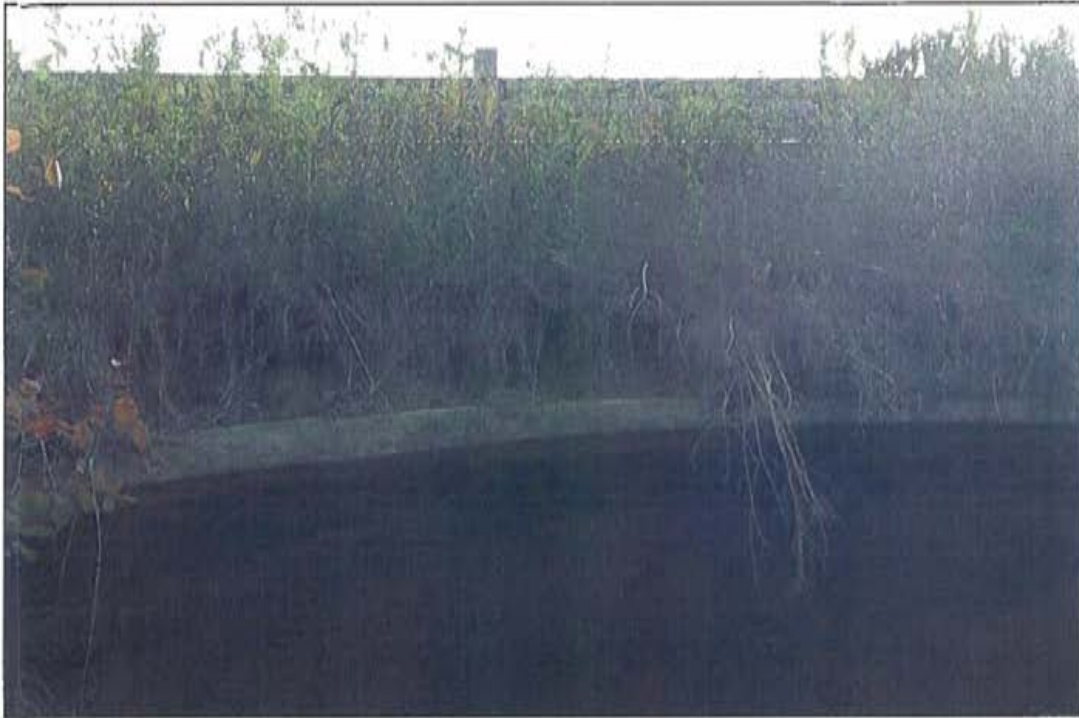
Photo 11: North side: unstable fill above crown.
