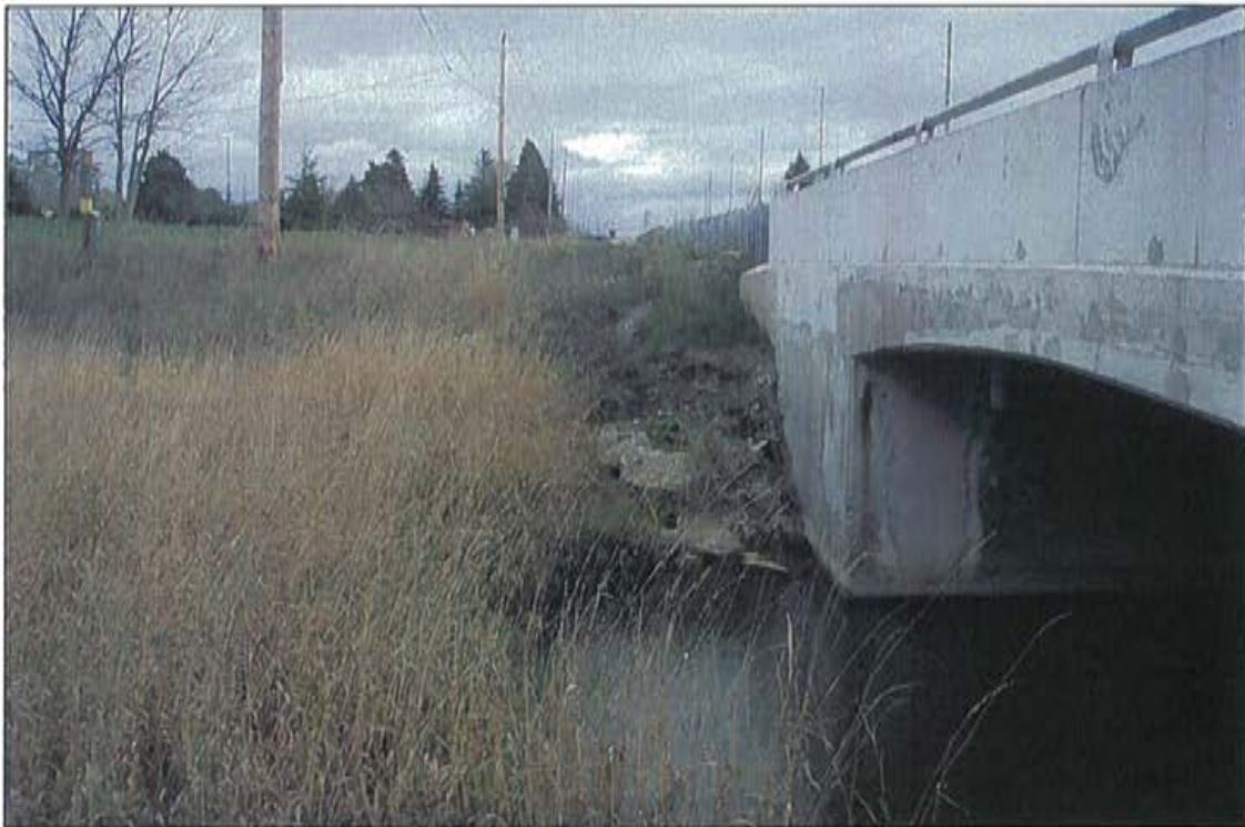
Photo 32: Embankment, east approach, north side: erosion.
