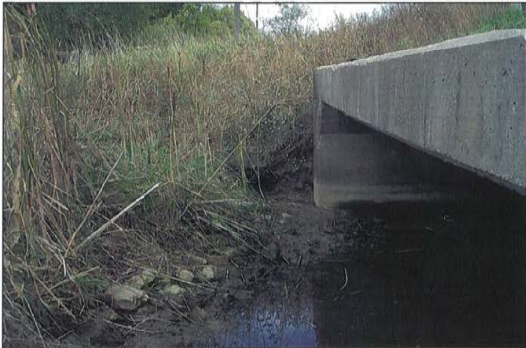
Photo 10: Embankment erosion, east approach, north side.
