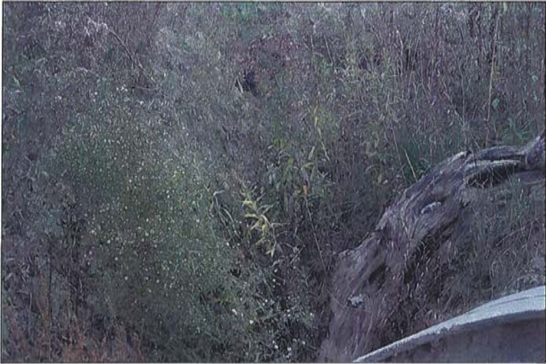
Photo 7: Embankment, north side: erosion.
