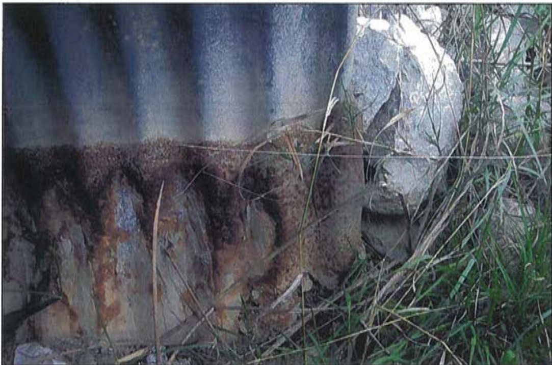
Photo 2: Outlet, east wall: severe corrosion.
