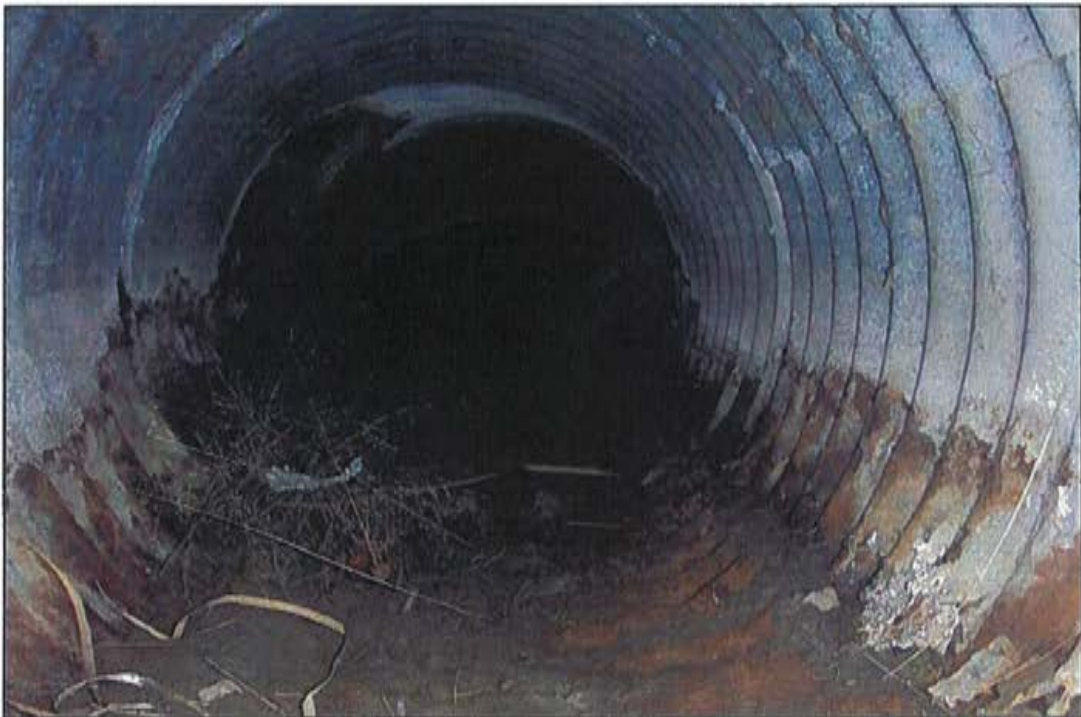
Photo 2: Inlet end, looking north: blocked.
