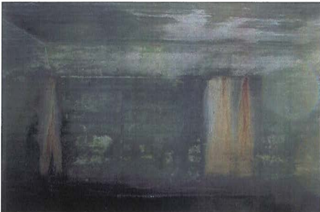
Photo 18: East culvert wall: exudation, wet area.
