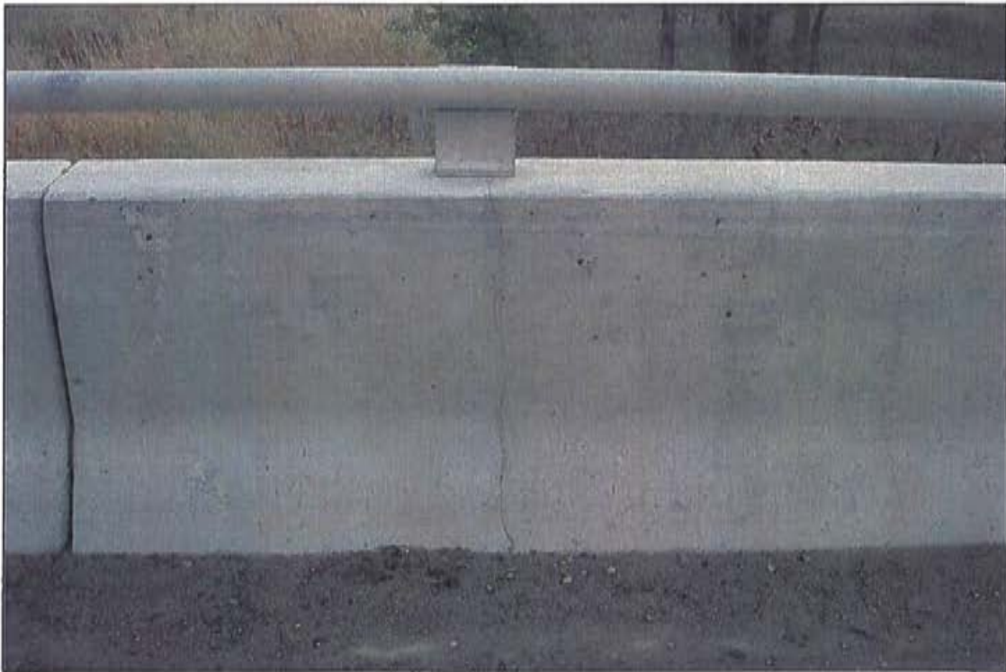
Photo 7: Concrete barrier, south side: medium crack.
