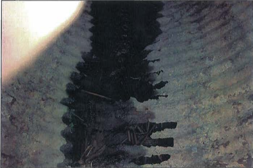
Photo 3: Inlet end: severe corrosion through bottom of CSP.
