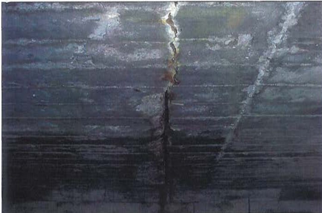
Photo 17: Underside of culvert barrel: spall and delamination.
