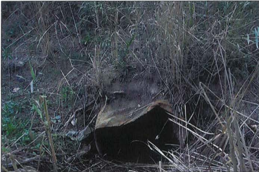
Photo 2: Outlet, looking north: deformation and impact damage.
