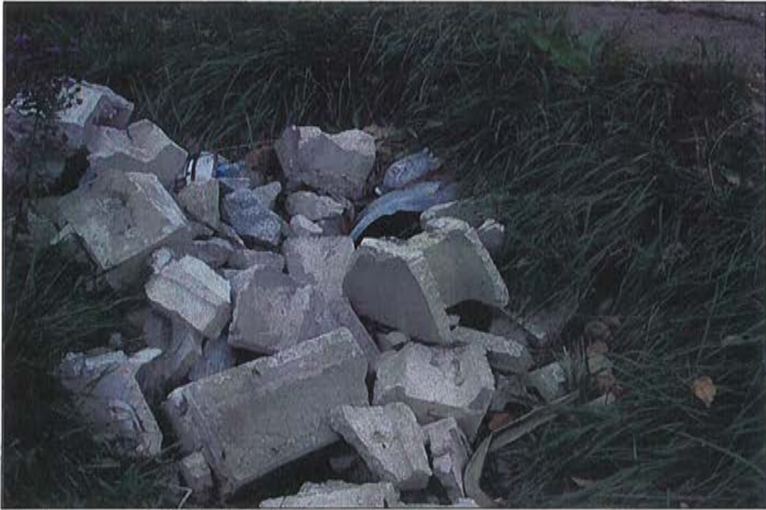
Photo 3: Inlet end: blocked with concrete debris.
