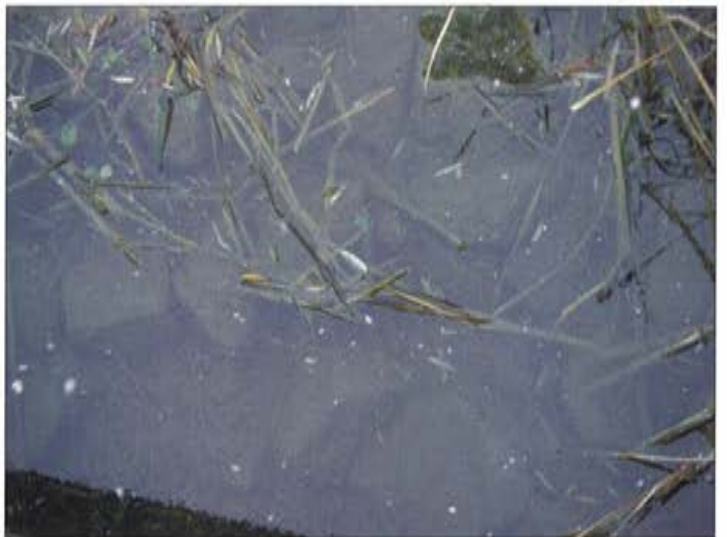
Photo 6c: Stn 6, standing water at north culvert. Nov 08, 2007.
