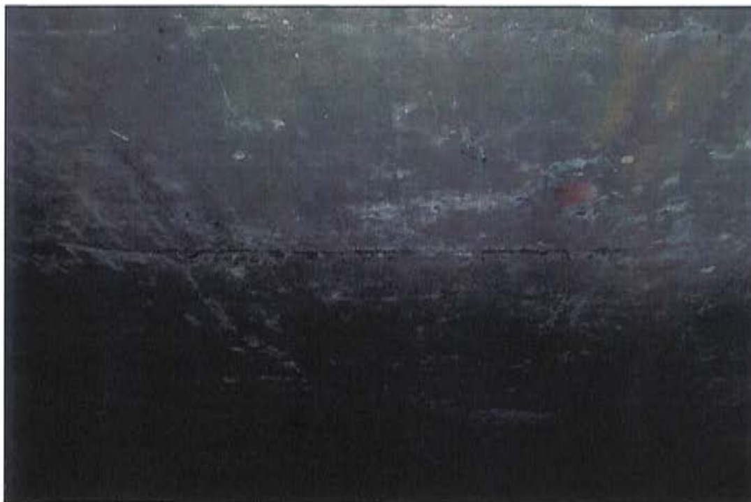
Photo 16: Culvert slab: spall.
