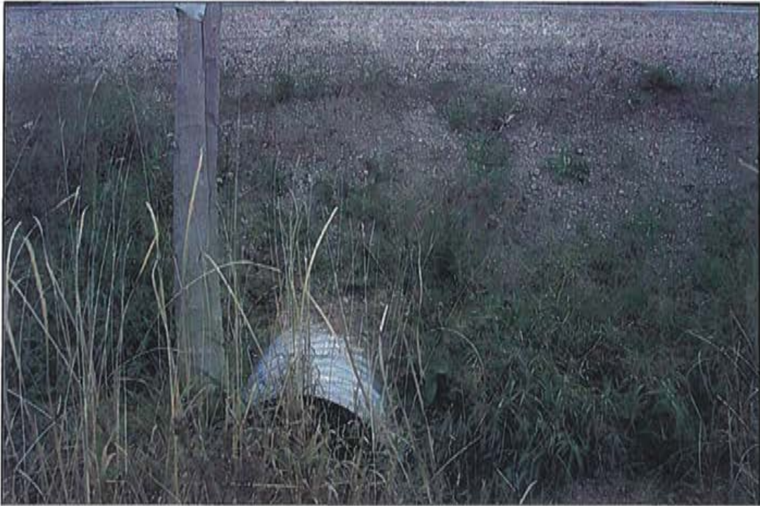
Photo 3: Inlet, looking south: blocked with vegetation.
