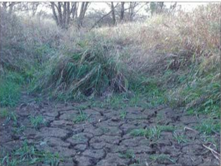
Photo 12b: Stn 12, The Gore Road tributary. 5-8m north (u-s) of culvert on north side of Mayfield rd. Nov 13, 2007.
