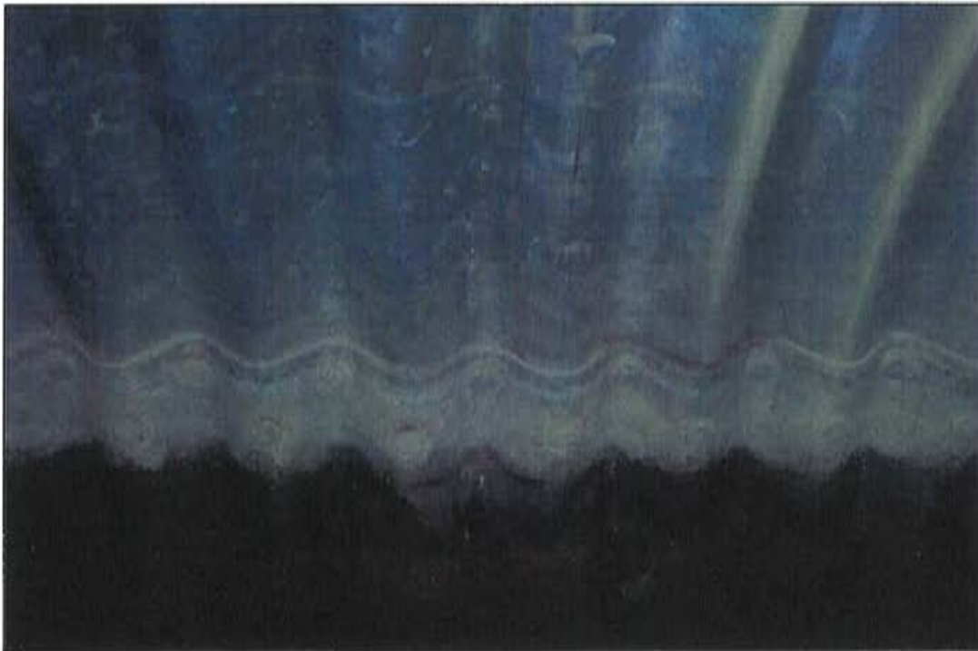
Photo 4: Impact damage, west wall at inlet.
