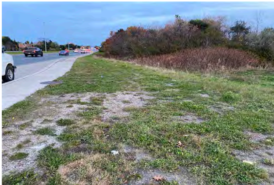
Image 44: LID area 16 showing disturbance, facing southeast
