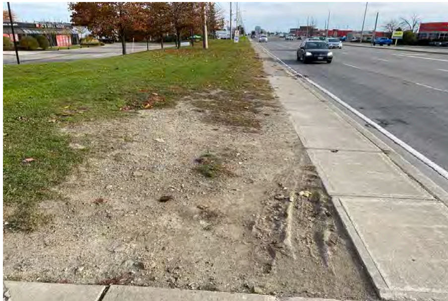
Image 33: LID area 13 showing disturbance, facing southeast
