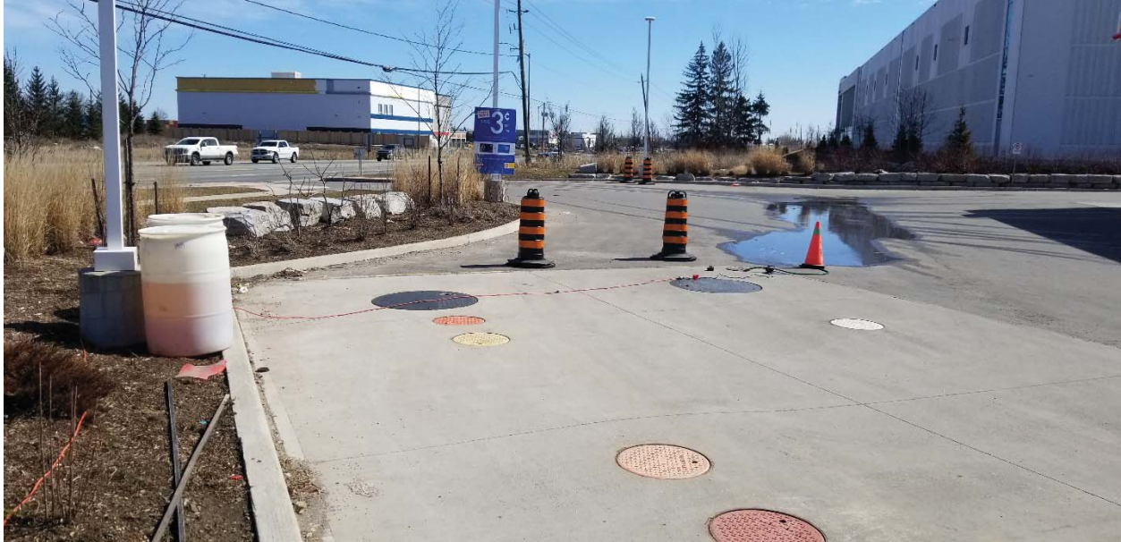
Photo 35: While completing reconnaissance at the Shell Gas Station, two drums were noted at the north east corner of the property adjacent to the fuel storage tanks and the Site. The drums appear to be filled with a dyed fuel. It was also noted that a small pump was inserted into an observation well around the fuel storage tanks and was discharging water directly into a neighboring catch basin in the parking lot. The drums, pump and discharge water are visible in the photo.
