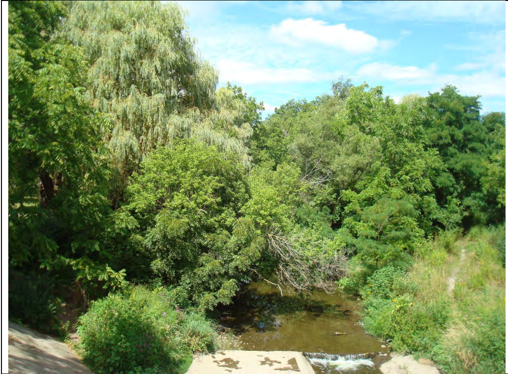
Photo 9. FOD 7-5 community and upstream limit of concrete channel at Church St., looking north.
