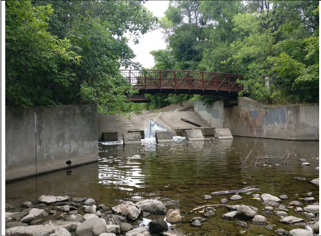
Photo 13. Weir at downstream limit of concrete channel. Looking north towards Pedestrian Bridge 3.
