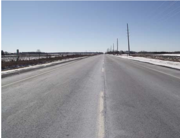
Figure 4-6 - Good Pavement Structure with mild rutting
