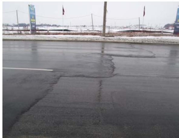
Figure 4-9 - Recently repaved area showing ramping
