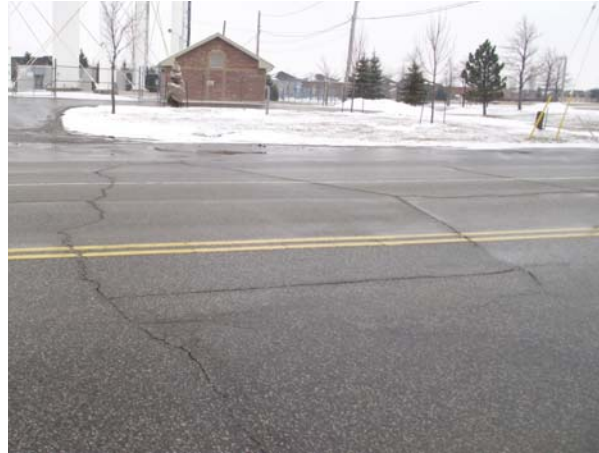
Figure 4-7 - Moderate transverse cracking
