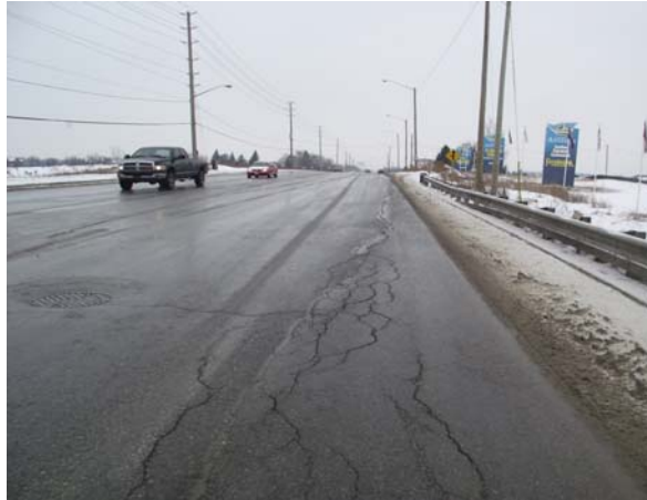
Figure 4-10 - Severe longitudinal cracking
