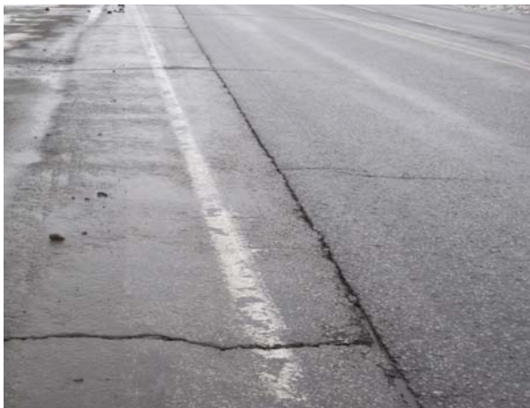
Figure 4-8 - Severe longitudinal cracking
