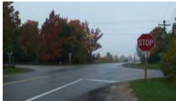
Figure 16: Faded Stop Bar Pavement Marking at Intersection of Bush Street and Shaws Creek Road
