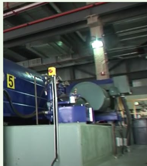
Thickening & Dewatering (G.E. Booth Wastewater Treatment Plant)
