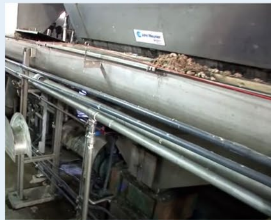
Screens and Grit Removal
