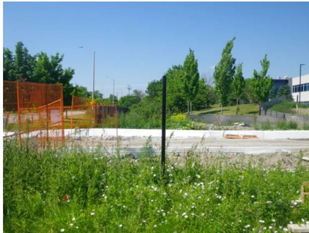
Image 4: View of access road under construction and flagged utility line (bottom left) near southeast corner of Clarkson WWTP.
