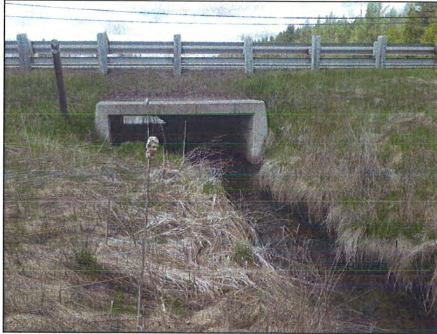
Tributary of Shaw's Creek: Looking north (upstream) from south of Queen Street East.
