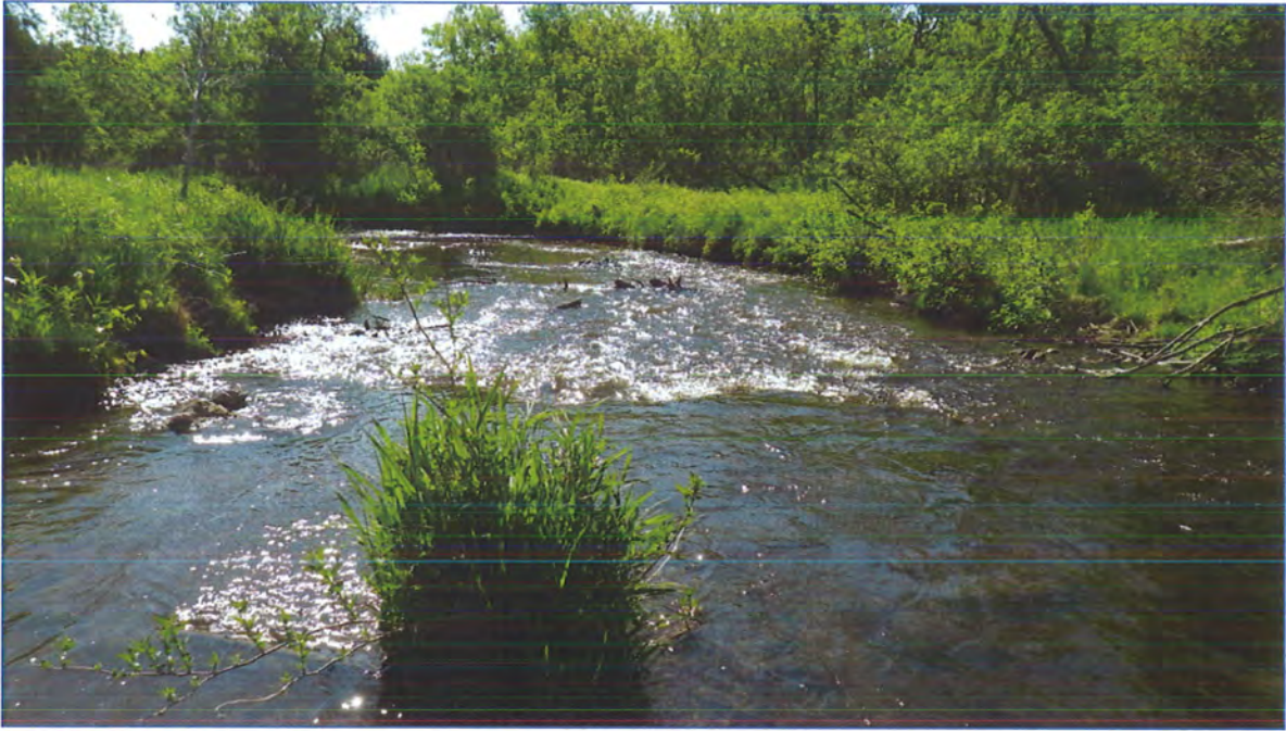
Photo 7: Shaws Creek - View downstream of bridge at Highway 136; coarse material in channel and bank erosion/undercutting along banks visible.
