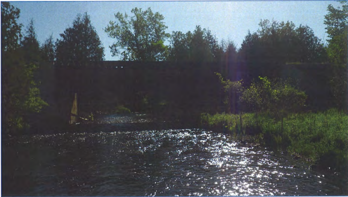
Photo 1: Shaws Creek - View downstream of railway crossing at upstream extent of study reach; left abutment exposed and floodplain extends 7 m into bridge span.
