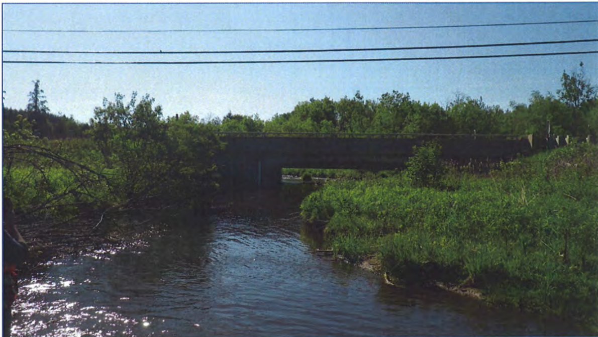
Photo 6: Shaws Creek - View downstream of bridge at Highway 136; note the leaning /failed shrubs along left bank due to erosion and the misalignment of the channel with the bridge opening.
