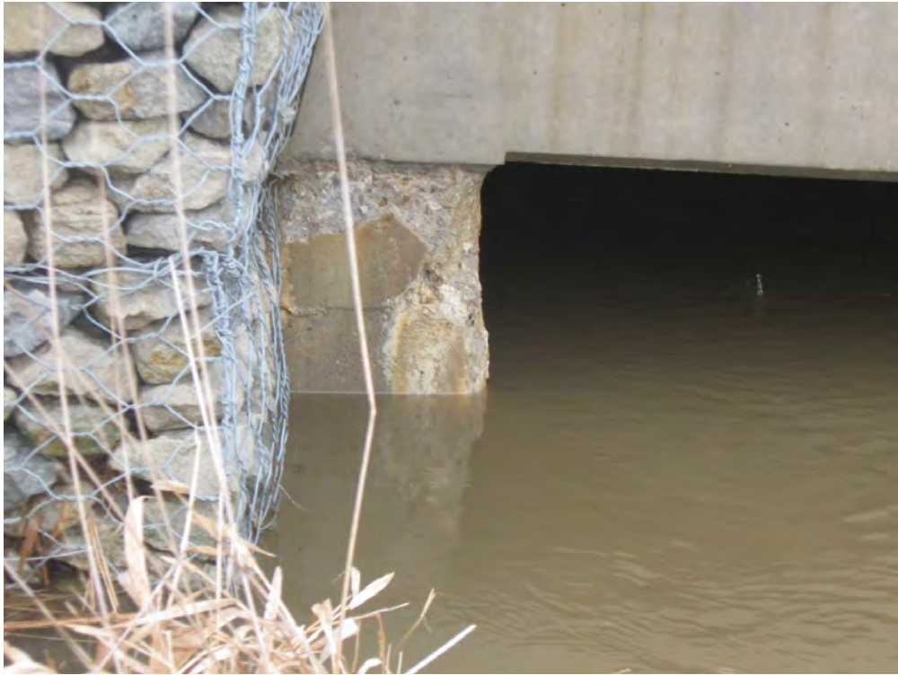
3. Severe scaling on North- West Culvert Wall
