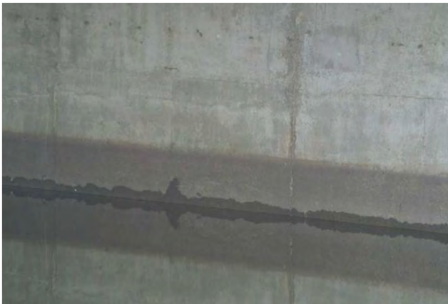
Plate 14: Detail of the north abutment. Note the indication of fluctuating water level.
