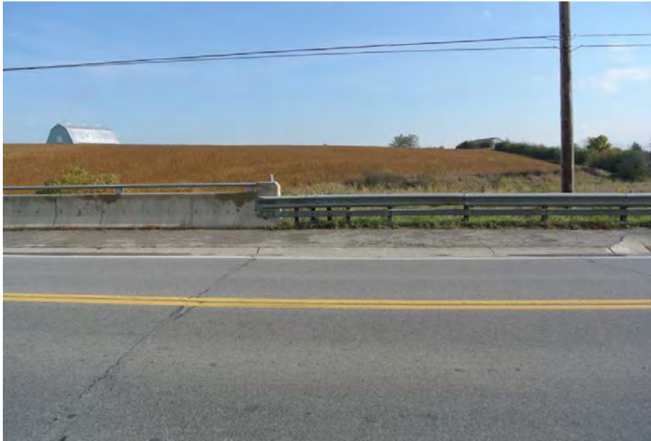
Plate 9: Detail of metal barrier system and concrete railing system located at the southeast corner of the bridge.
