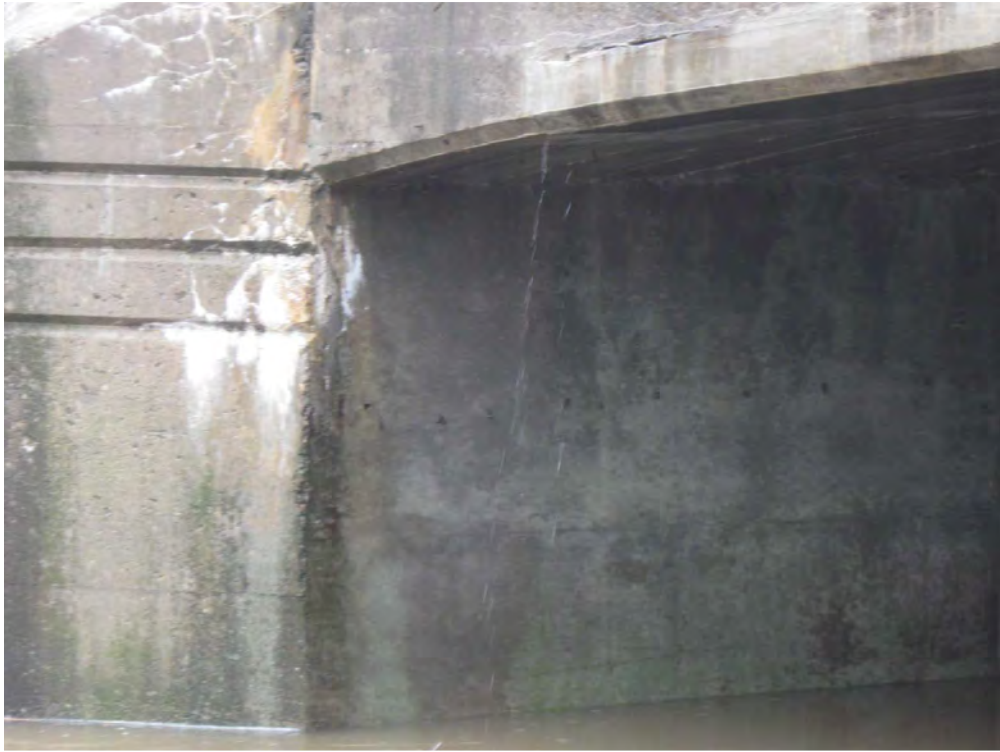
7. Efflorescent and staining on wingwall
