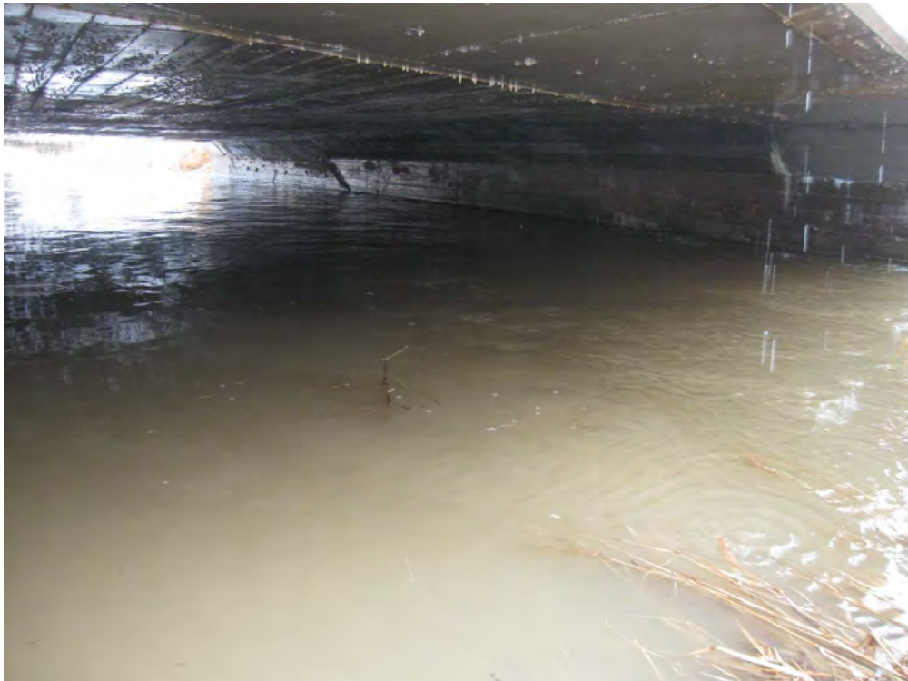
4. Efflorescence and leaking construction joint in soffit
