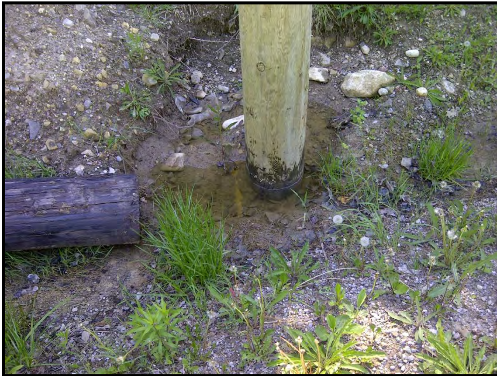
Figure 5 Winston Churchill Blvd. - Depress Areas near a Hydro Pole in Shoulder
