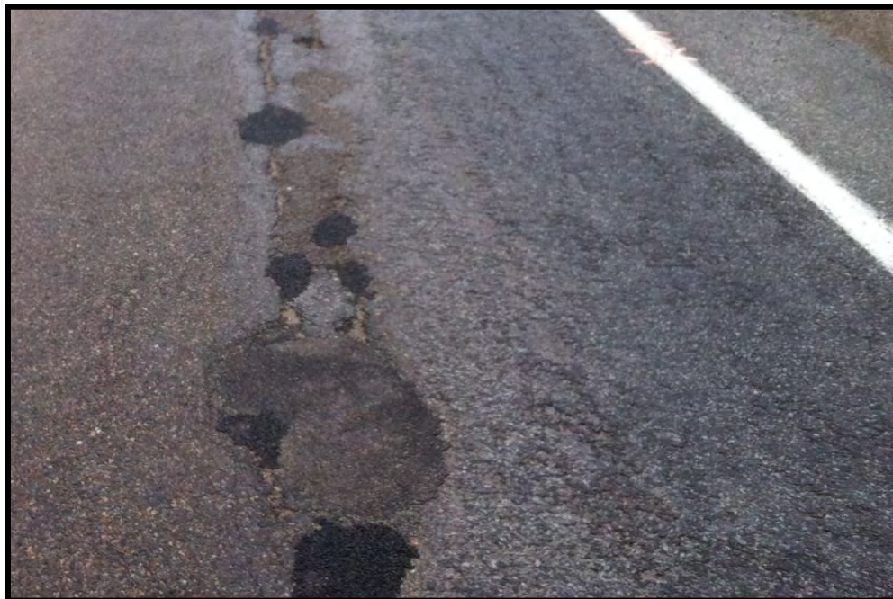
Figure 2 Winston Churchill Blvd. - Close up on Pavement Surface Condition: Failing Patch Work, Severe Ravelling
