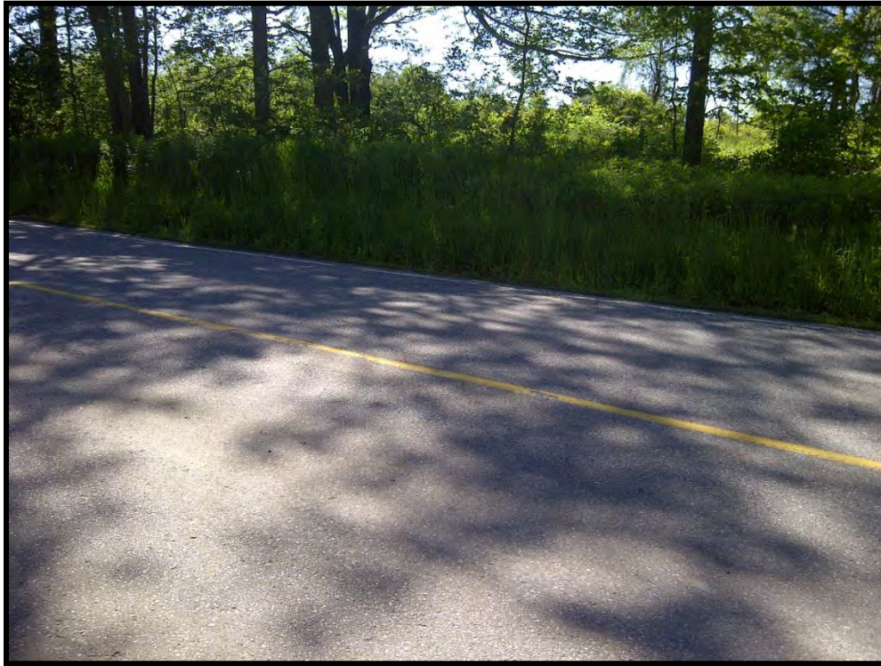
Figure 7 Olde Base Line - Typical Condition of Roadway
