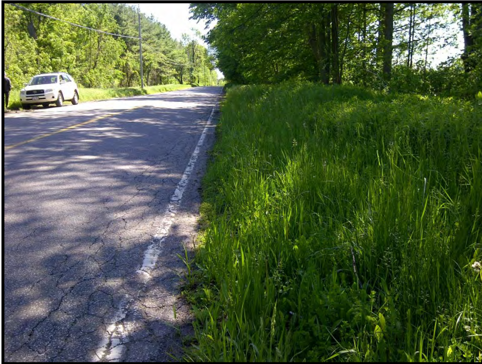
Figure 9 Olde Base Line - Very Narrow (or No) Shoulder, Tall Grass, Extensive Pavement Edge Cracking
