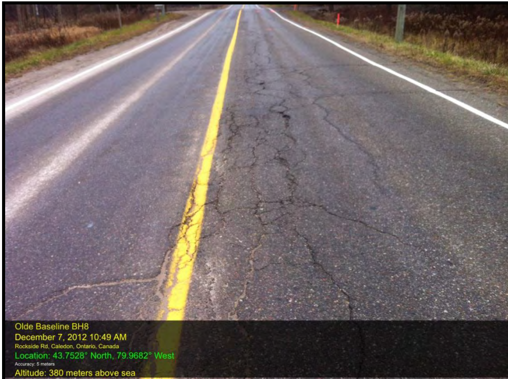
Figure 8 Olde Base Line - Multiple High Severity Longitudinal Cracks
