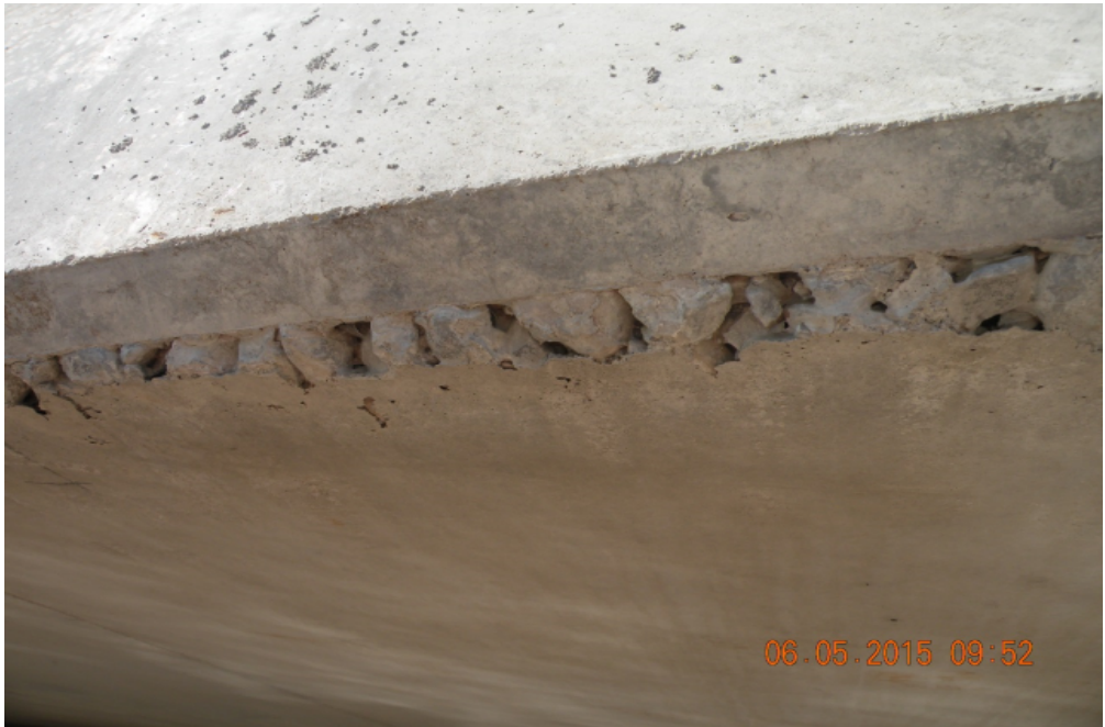
Honeycombing at Soffit
