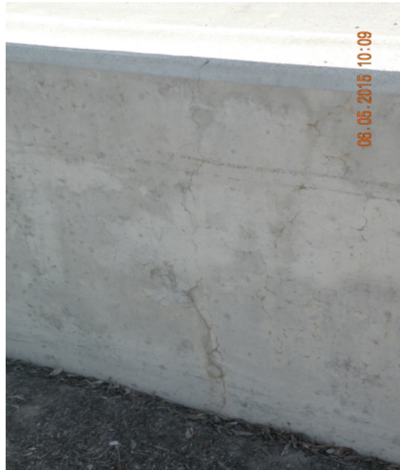
Narrow Crack on Interior Parapet Wall
