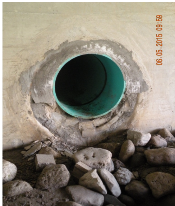
Spalling around PVC Inlet
