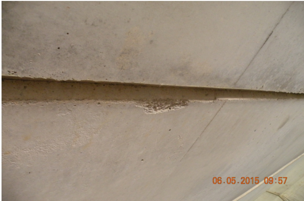
Spall at Soffit Joint
