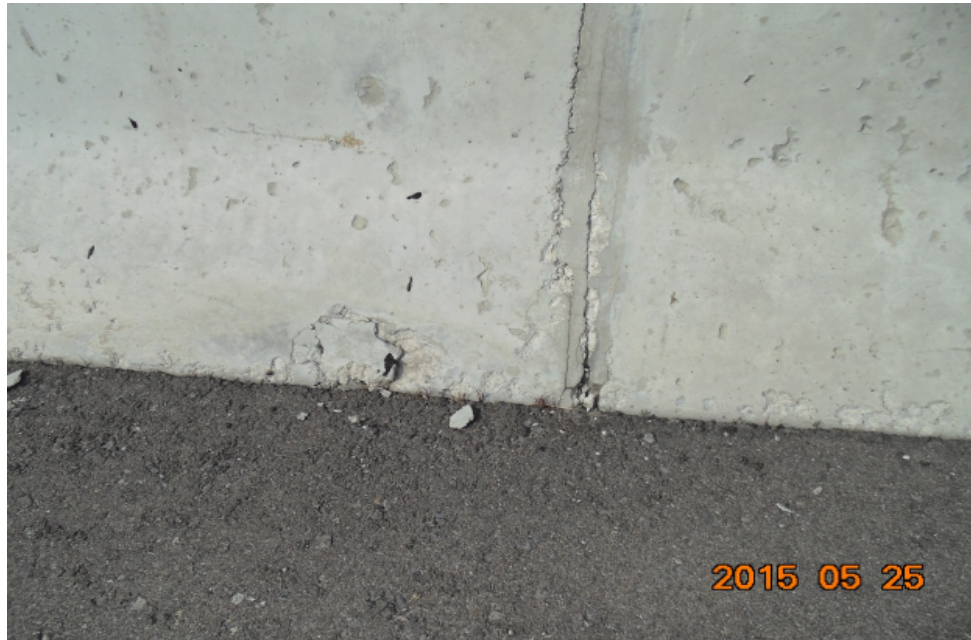
Typical Scaling on Barrier Wall
