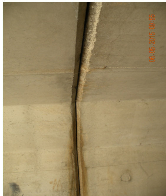
Joint with Staining and Scaling
