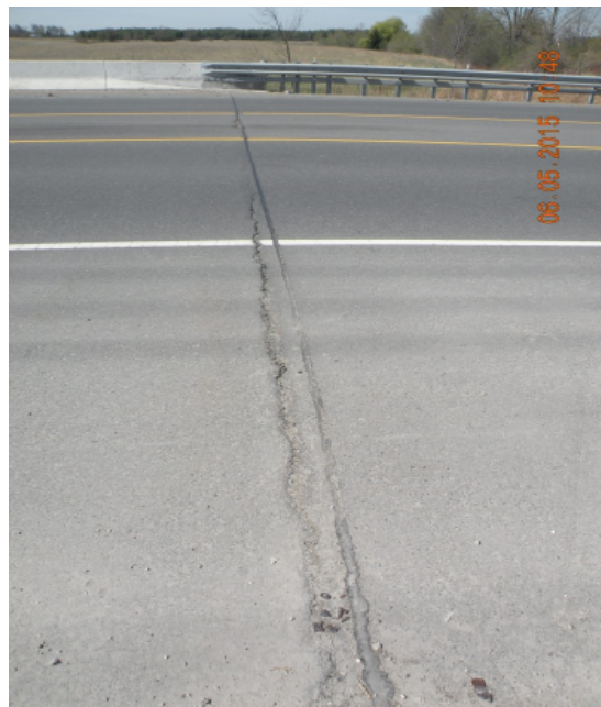
Crack on Approach Wearing Surface
