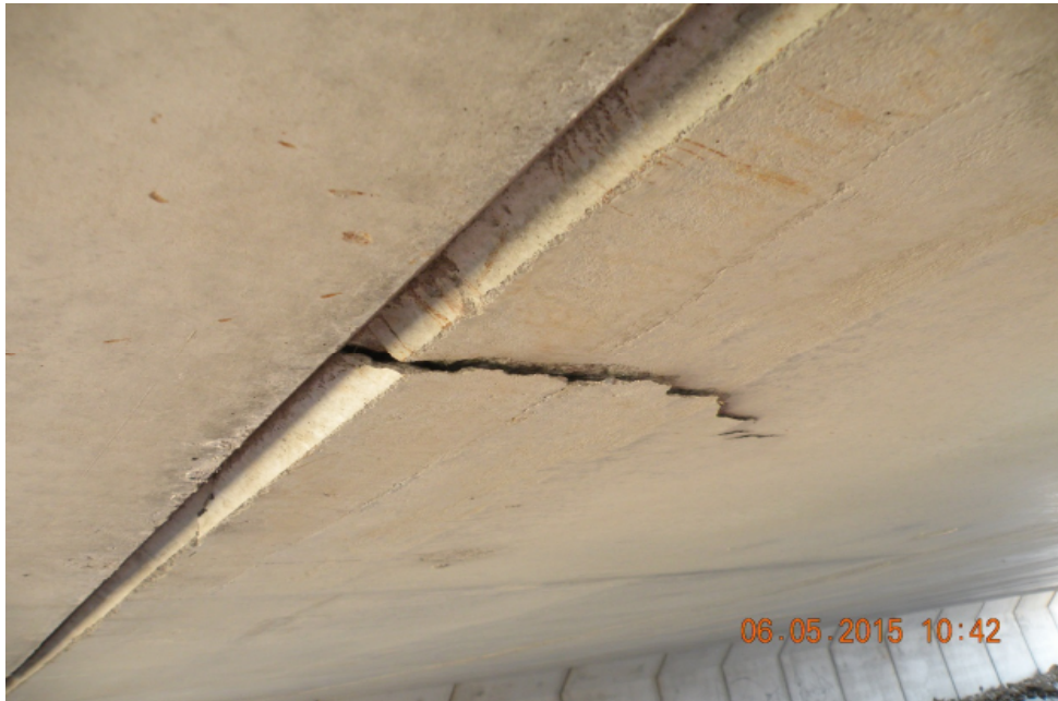
Delamination in third panel from West End
