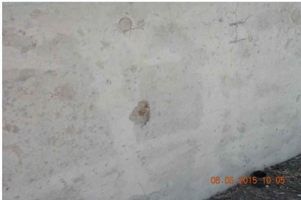
Spall on Interior Parapet Wall
