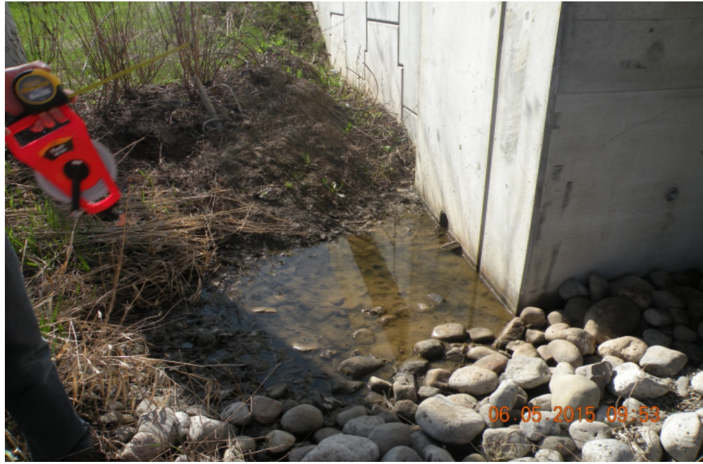
Typical Ponding at Abutment Corners
