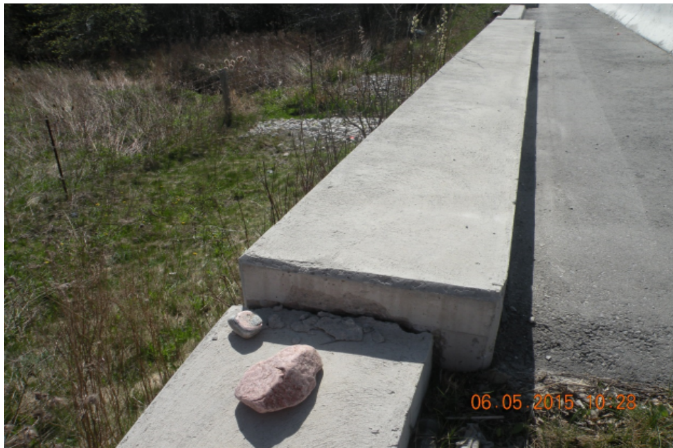
Disintegrated Concrete at RSS Connection
