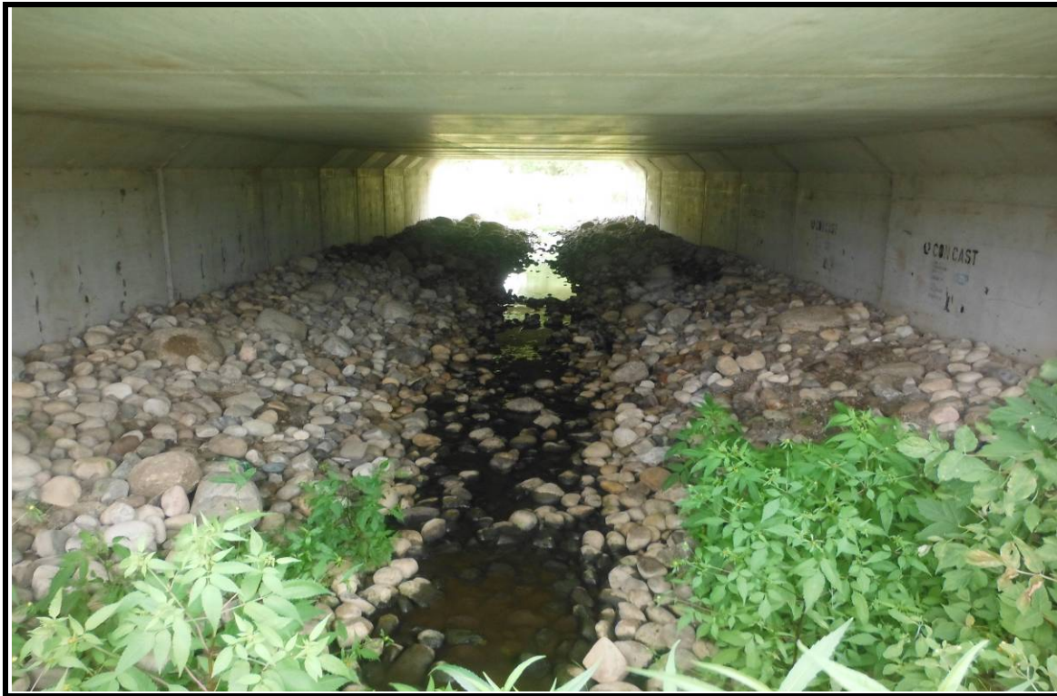
PHOTOGRAPH NO.: 9 - Culvert 8 FROM: Downstream side of culvert LOOKING: Through culvert COMMENT:
