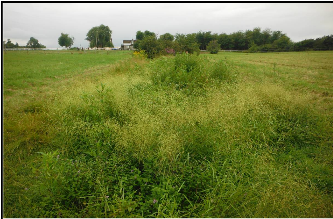
PHOTOGRAPH NO.: 10 - Culvert 8 FROM: Upstream of culvert at road LOOKING: Upstream at channel COMMENT:
