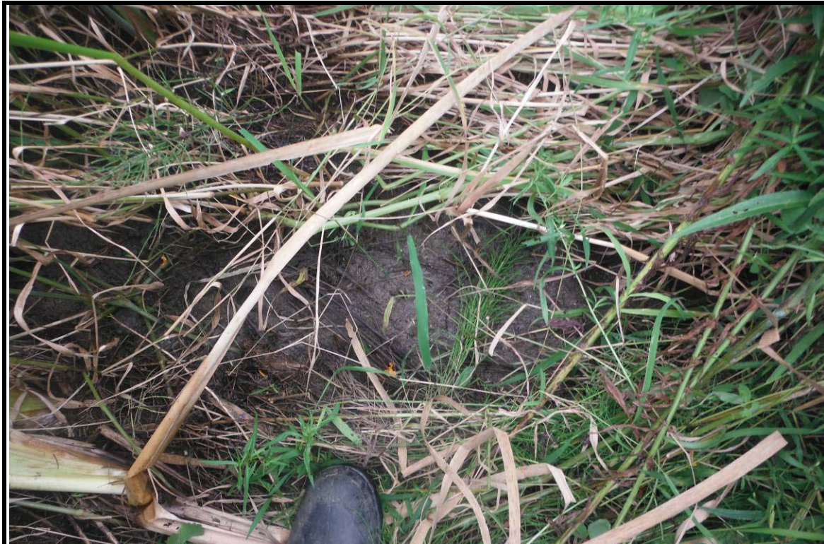
PHOTOGRAPH NO.: 3 - Culvert 3 FROM: In channel LOOKING: At channel bed COMMENT: Note lack of flows
