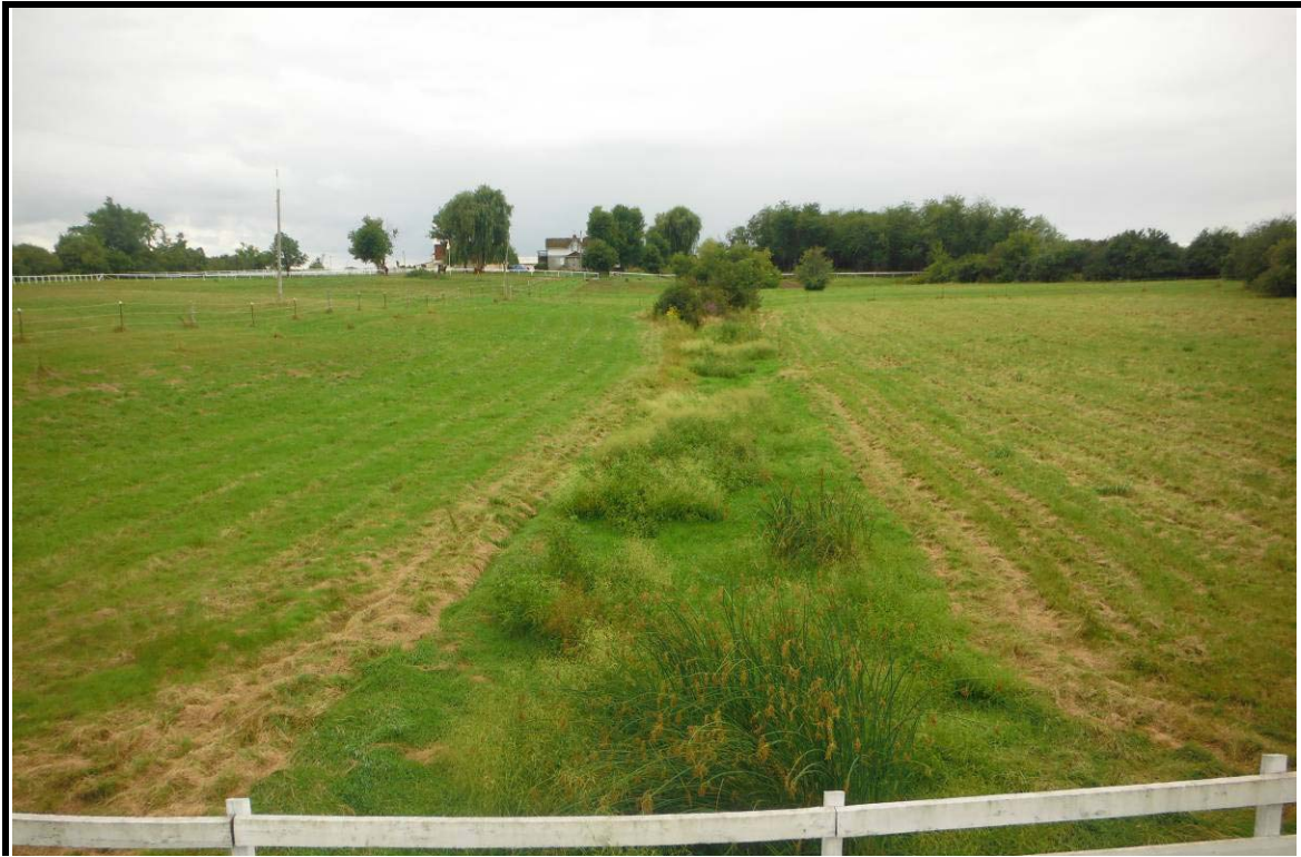
PHOTOGRAPH NO.: 11 - Culvert 8 FROM: From road culvert LOOKING: Upstream at channel COMMENT:
