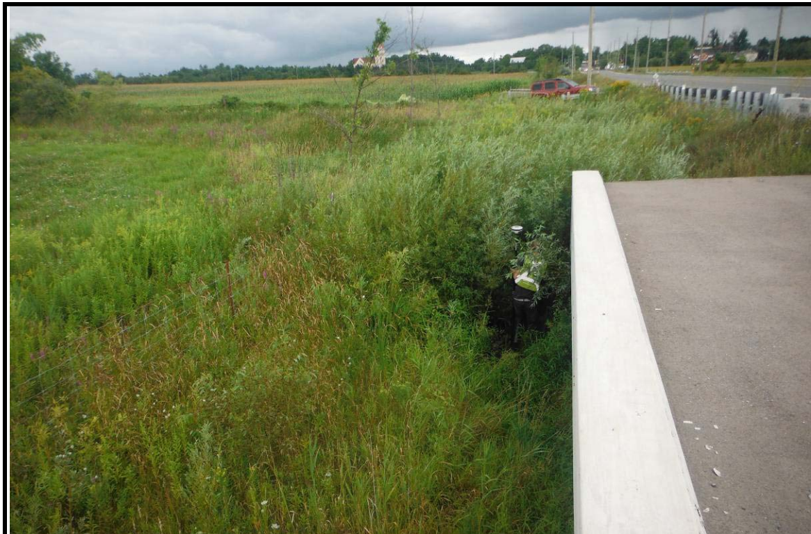
PHOTOGRAPH NO.: 4 - Culvert 3 FROM: From road culvert LOOKING: Upstream at channel COMMENT:
