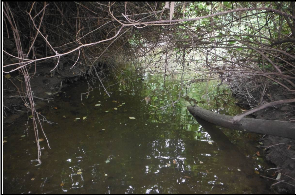
PHOTOGRAPH NO.: 12 - Culvert 10 FROM: In channel on downstream side LOOKING: Upstream COMMENT:
