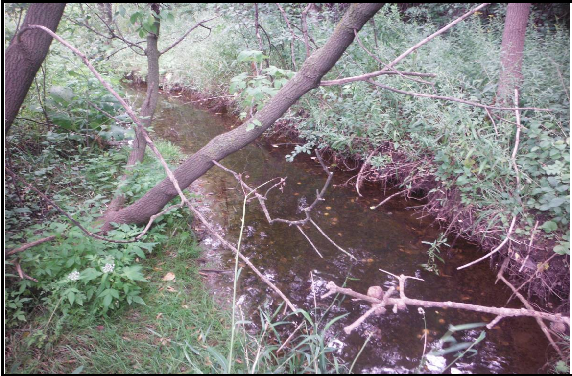
PHOTOGRAPH NO.: 7 - Culvert 8 FROM: In channel on downstream side LOOKING: Downstream COMMENT:
