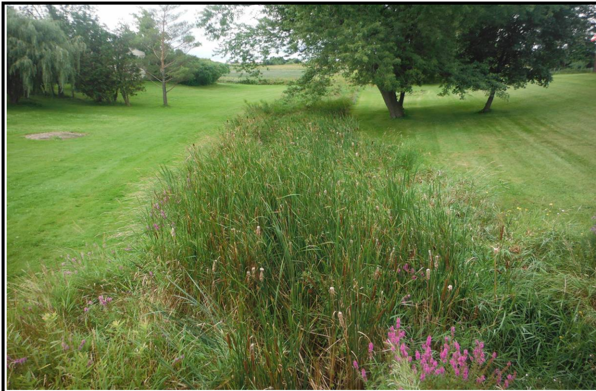
PHOTOGRAPH NO.: 17 - Culvert 10 FROM: In channel on upstream side LOOKING: Upstream at channel COMMENT:
