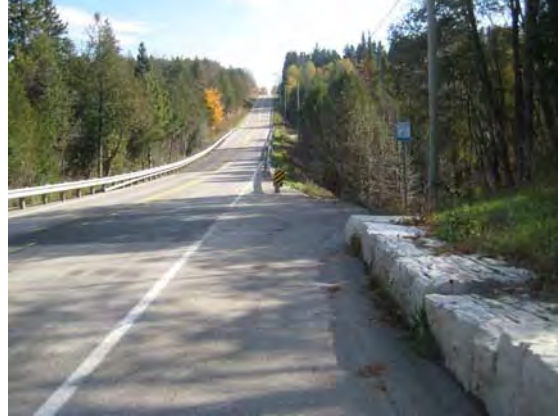
Plate 26: Southeast view along Winston Churchill Boulevard across valley. Road is raised above valley floor/steeply sloping lands. No potential.
