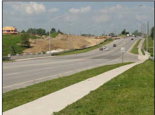
Plate 6: View of the bridge that carries Mayfield Road across Etobicoke Creek and of ongoing construction.
