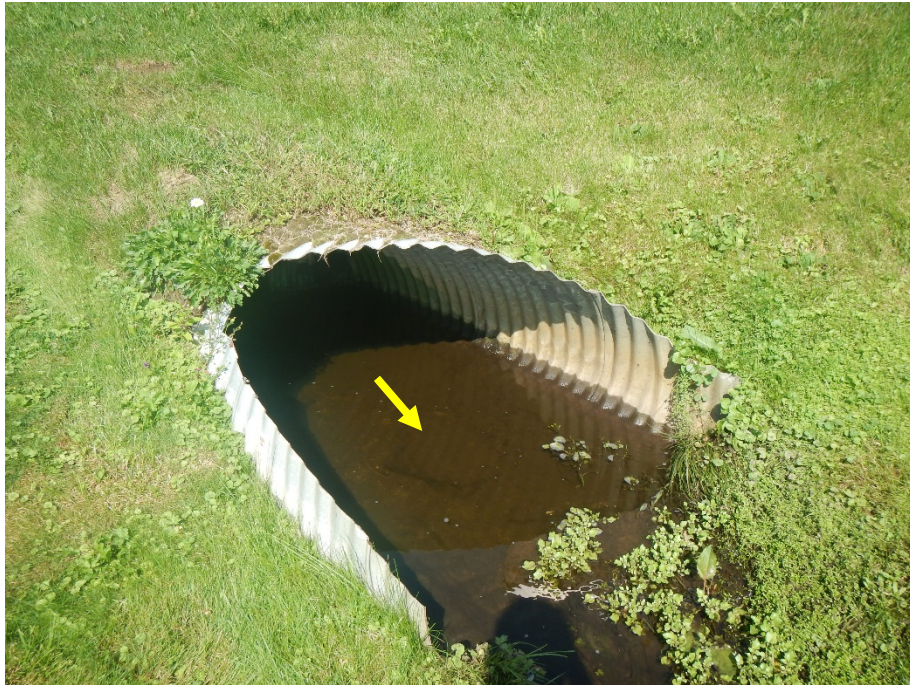
An elliptical culvert directed flows from the upstream forest reach (CVT-1) into a short, open channel to the west of Airport Road. Water seepage was observed at the upstream extent of the segment, evidence of a possible groundwater upwelling.
