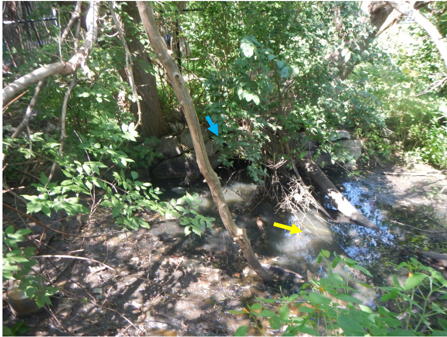
The downstream end of Crossing 2 (blue arrow) was backwatered, with standing water present within the culvert itself and downstream for approximately 10 m.
