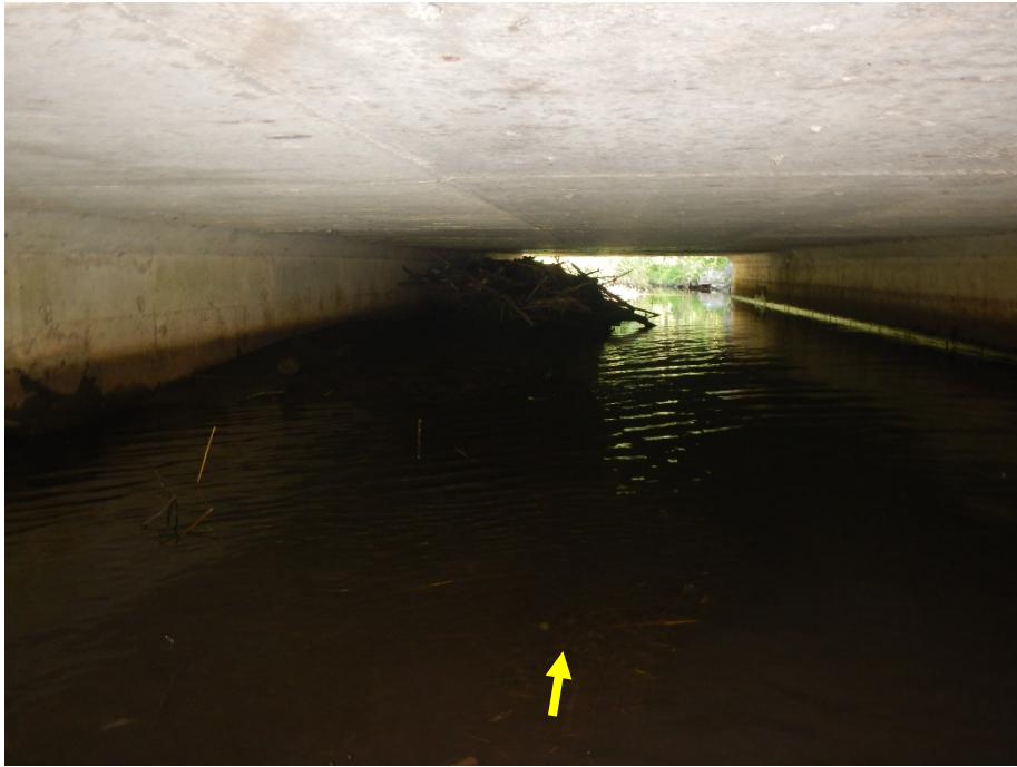
A woody debris jam was present which partially impeded flows within Crossing 3 beneath Airport Road.
