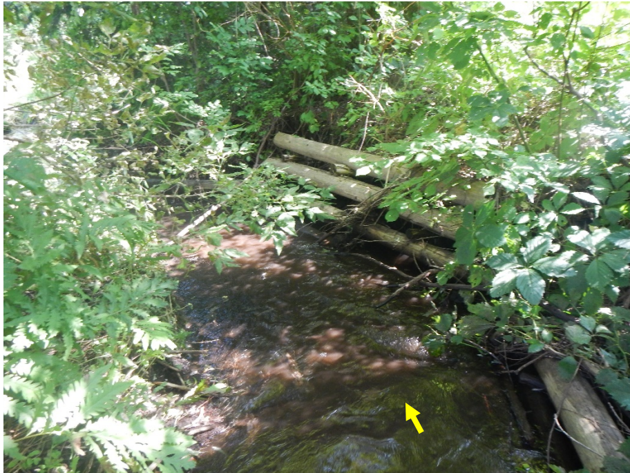
A crib wall was present along the outer bank of a left bend in the channel. There was significant loss of material within and behind the crib wall.
