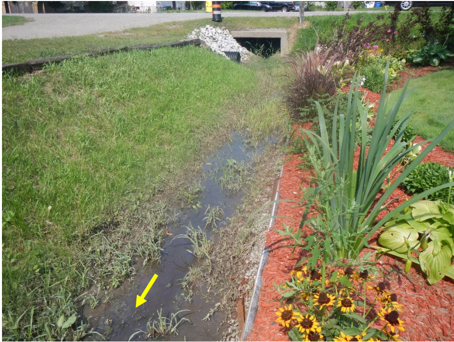
On the west side of Airport Road, the Crossing 7 outlet was partially blocked by rip rap, limiting its capacity to convey flows.
