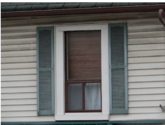
Figure 19: Detail of replaced window on the second floor of the east elevation.
