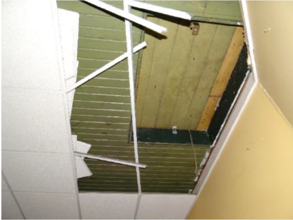
Figure 29: Attic hatch visible in the living room where ceiling panels were removed.
