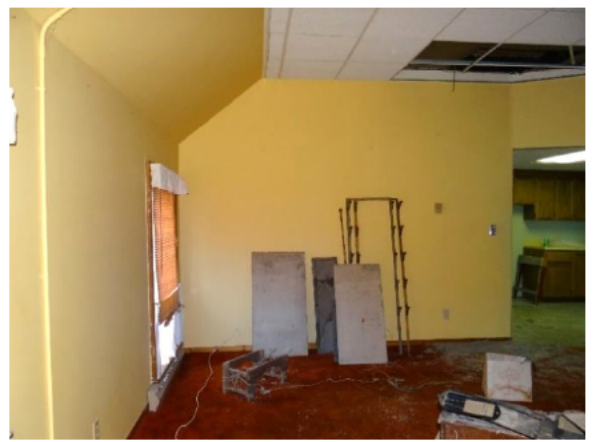
Figure 28: Living room, looking south with the kitchen at right. Note the drop panel ceilings and low baseboards.
