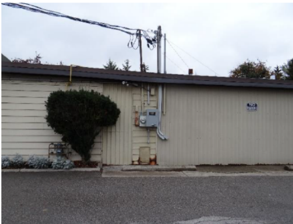
Figure 17: Detail of the change in vinyl siding signalling the 1985 addition at right and the earlier addition at left.
