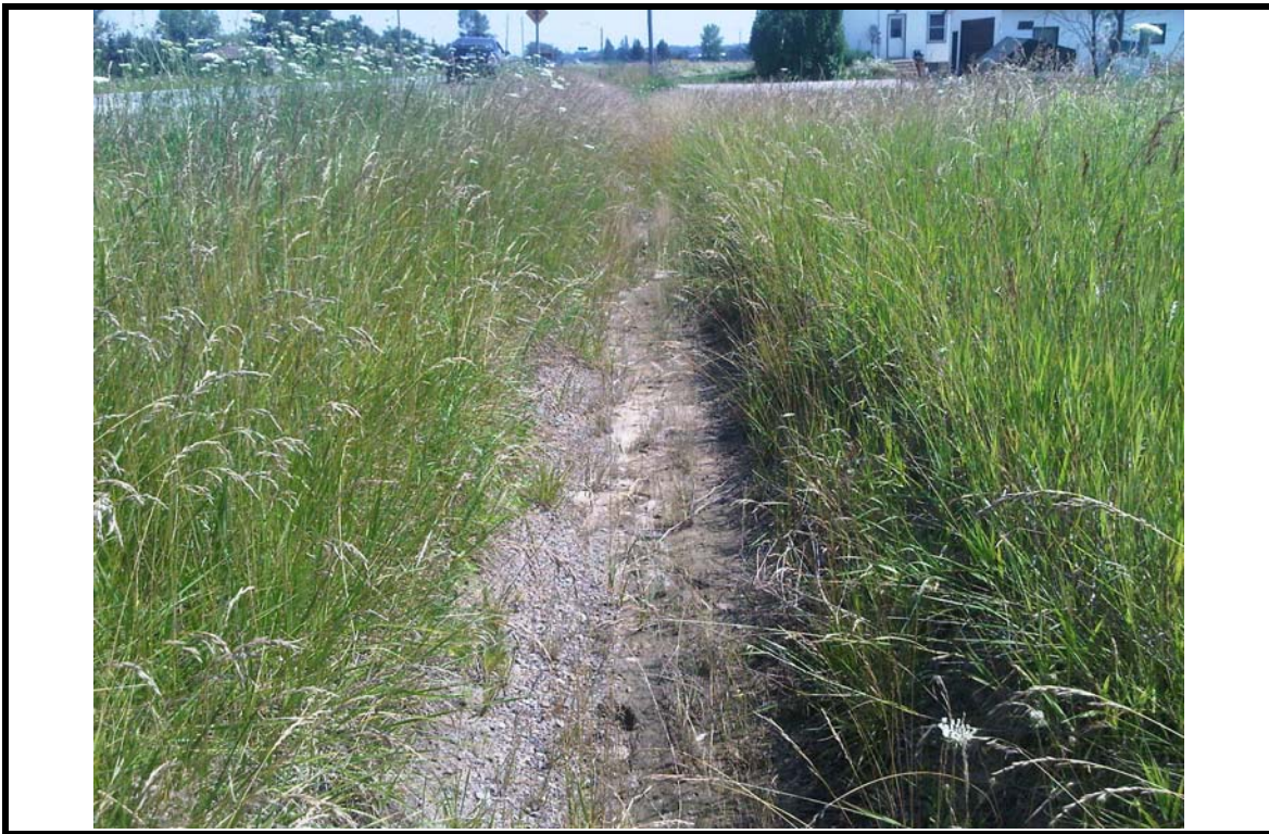
PHOTOGRAPH NO.: 6 FROM: LOOKING: At Ditch on downstream side of the road COMMENT: Reach D
