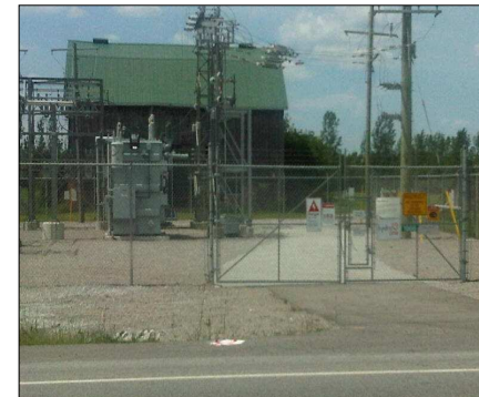
Hydro One Networks Station
