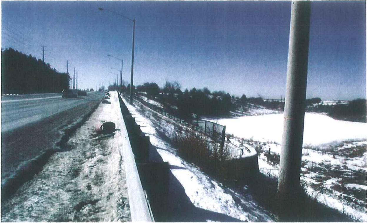
Mayfield Road\Section1\ Looking Towards West\Wetland Area at the North side of Mayfield Rd. , See the Retaining Wall to support the Road Embankment
