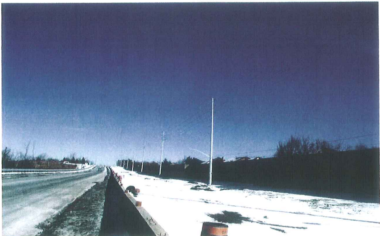
Mayfield Road\Section2\ Looking Towards East\Widening Construction for the Southside of Mayfield ,East of Kennedy Rd.
