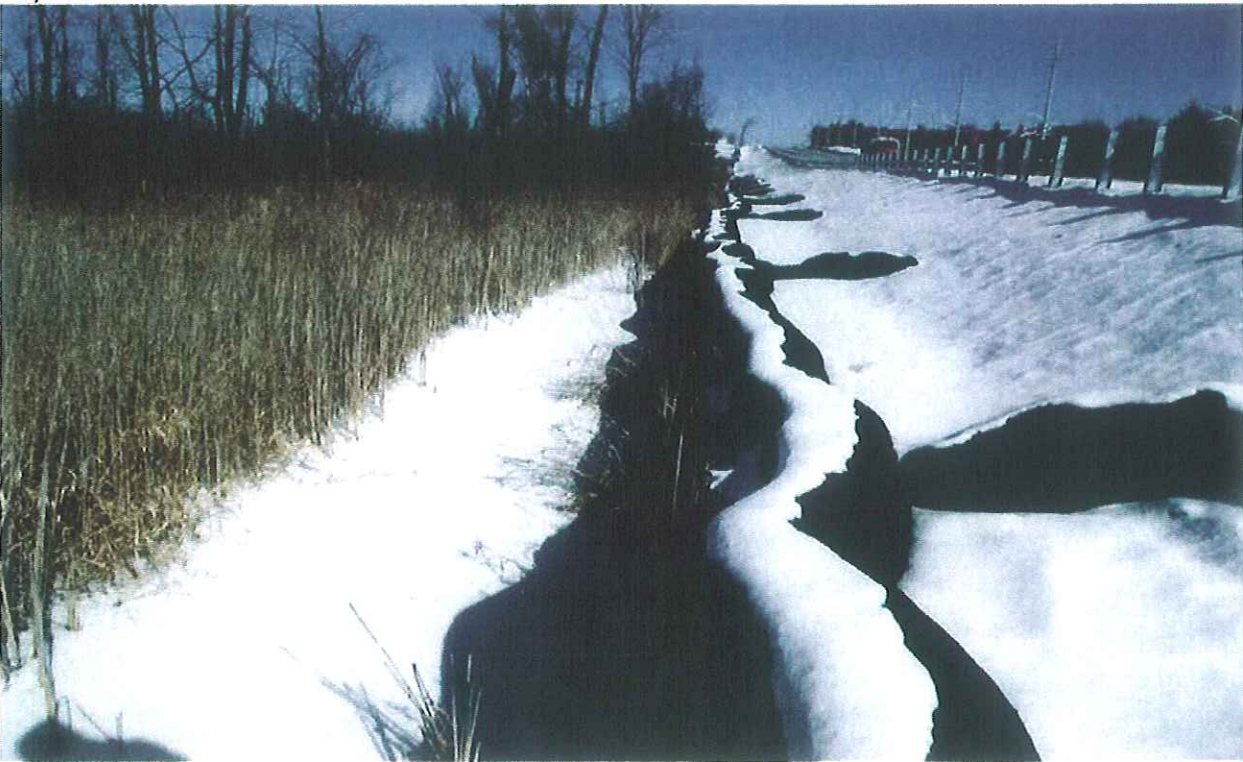
Mayfield Road\Section2\ Looking towards East\Steel Sheet Piles at the North Side of Mayfield Rd. as Retaining walls for the road Embankment (Approx. 400 m long)
