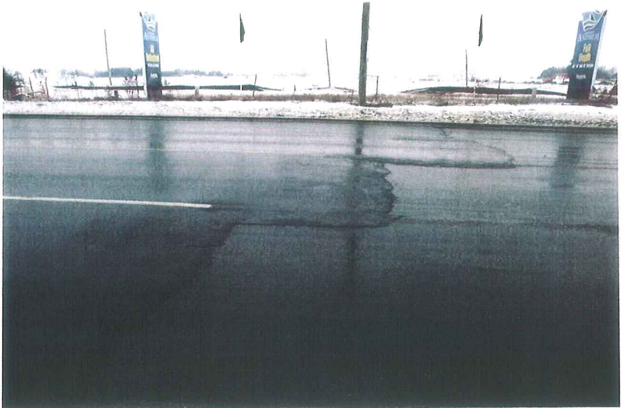
Mayfield Road\Section2\ Looking towards North\End of Section 2 and Starting of Section 3, about 150 m West of Kennedy Rd.
