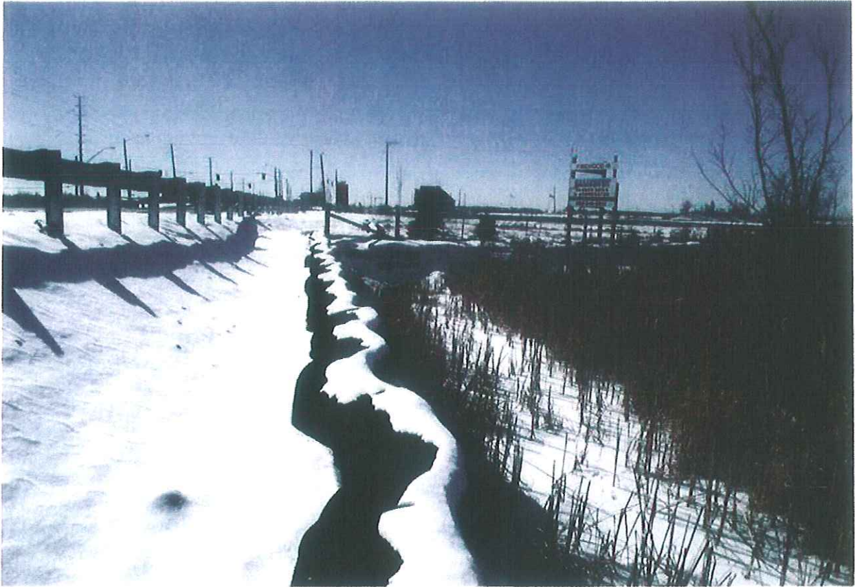
Mayfield Road\Section2\ Looking towards West\Steel Sheet Piles at the North Side of Mayfield Rd and Wetland Area to the North OF Mayfield Rd and East of Kennedy Rd.
