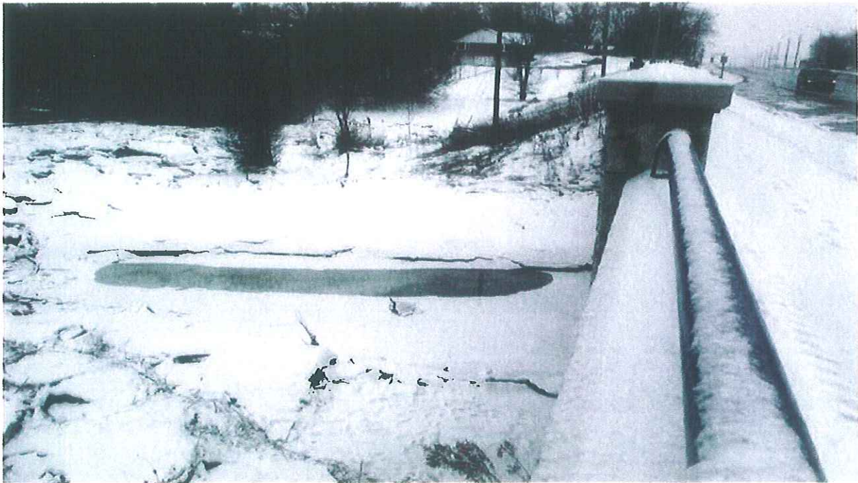
Mayfield Road\ Section 3\Looking towards West\Structural Bridge crossing a Tributary\700 m West of Kennedy Road
