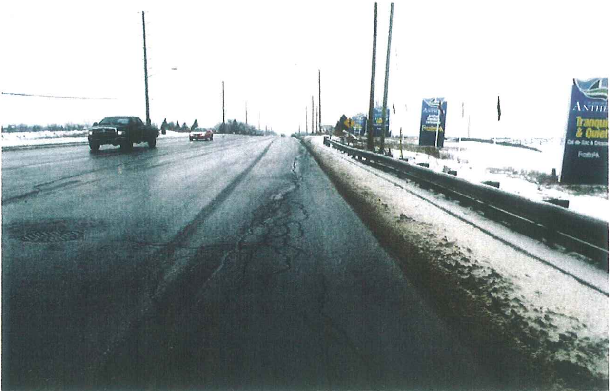
Mayfield Road\Section2\ Looking towards West \ from Kennedy Road to 150 m Westerly\see cracks and distortion area\ new Subdivision will be constructed at the North Side of Mayfield Rd. , West of Kennedy Rd.
