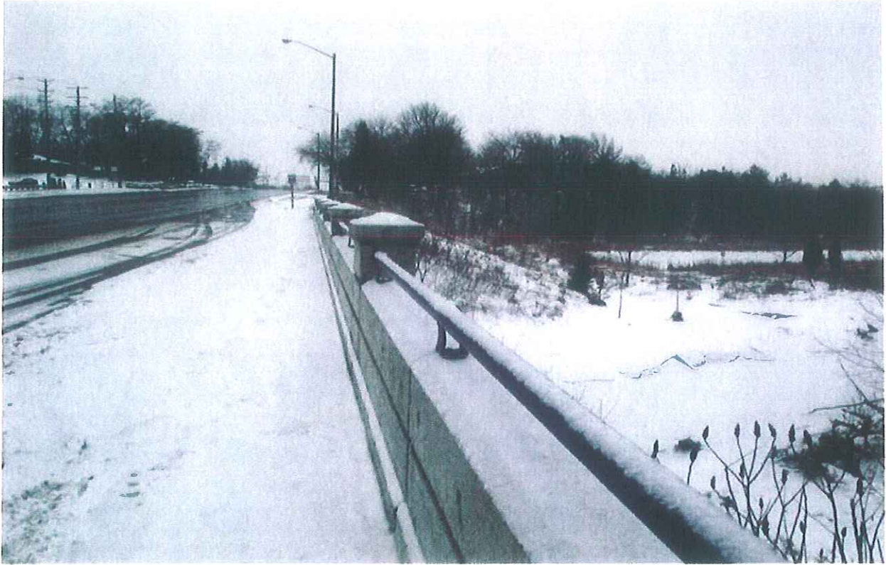
Mayfield Road\ Looking towards West\Structural Bridge crossing Tributary\700 m West of Kennedy Road
