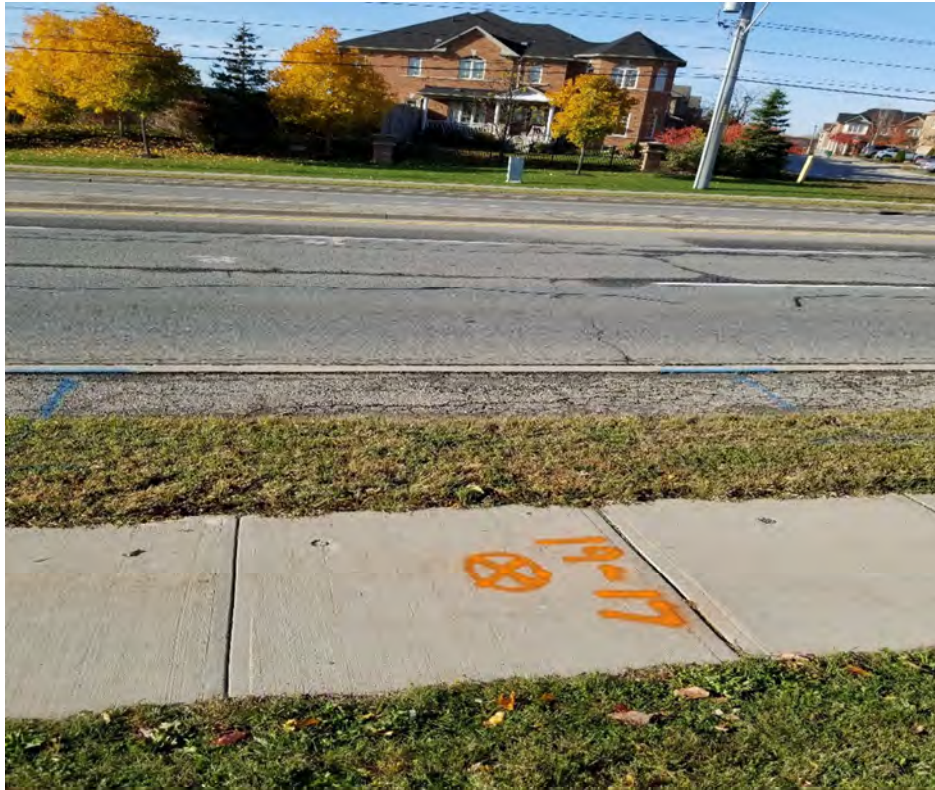
Photo 3 – Slight to Moderate Pavement Edge Cracking on Airport Road
