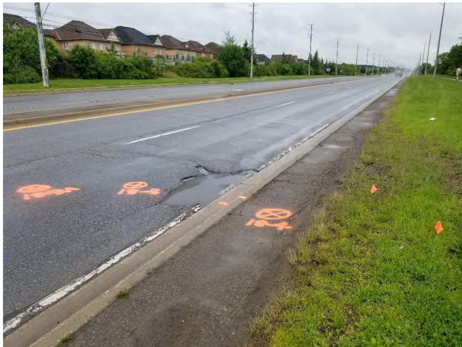
Photo 4 – Severe Pothole and Very Slight Rutting on Airport Road
