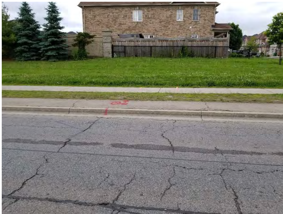
Photo 2 – Slight to Moderate Map Cracking on Airport Road
