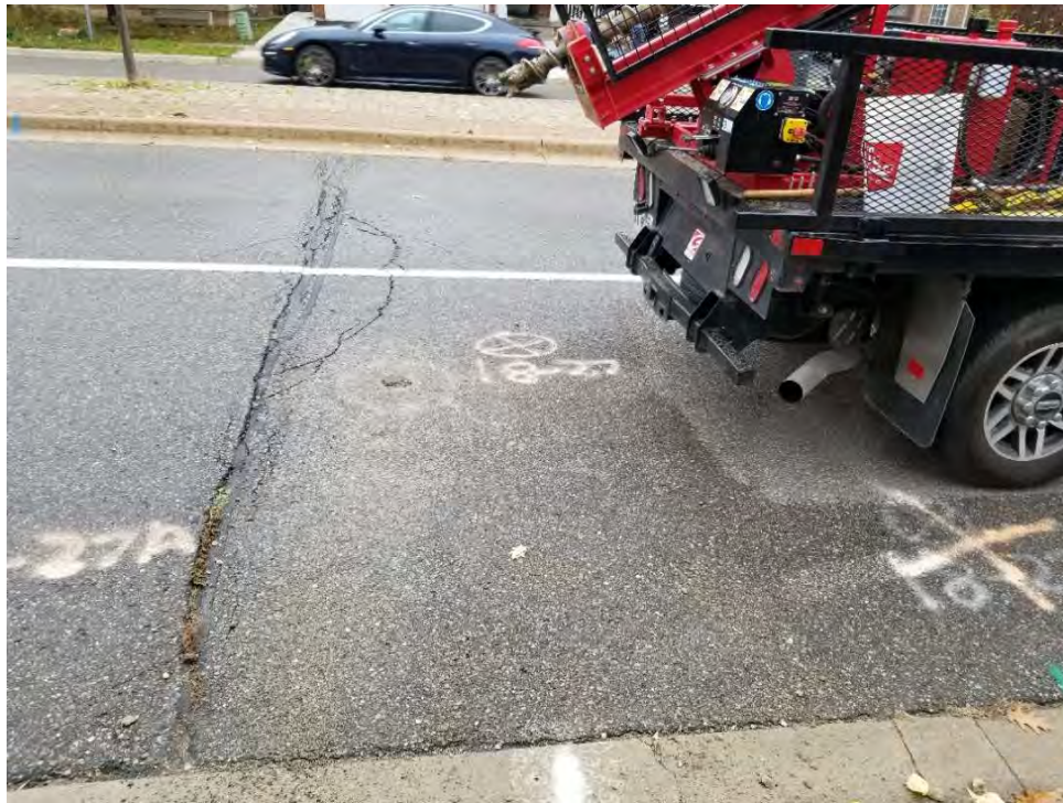
Photo 1 – Severe Transverse Cracking near Airport Road and Brock Drive Intersection
