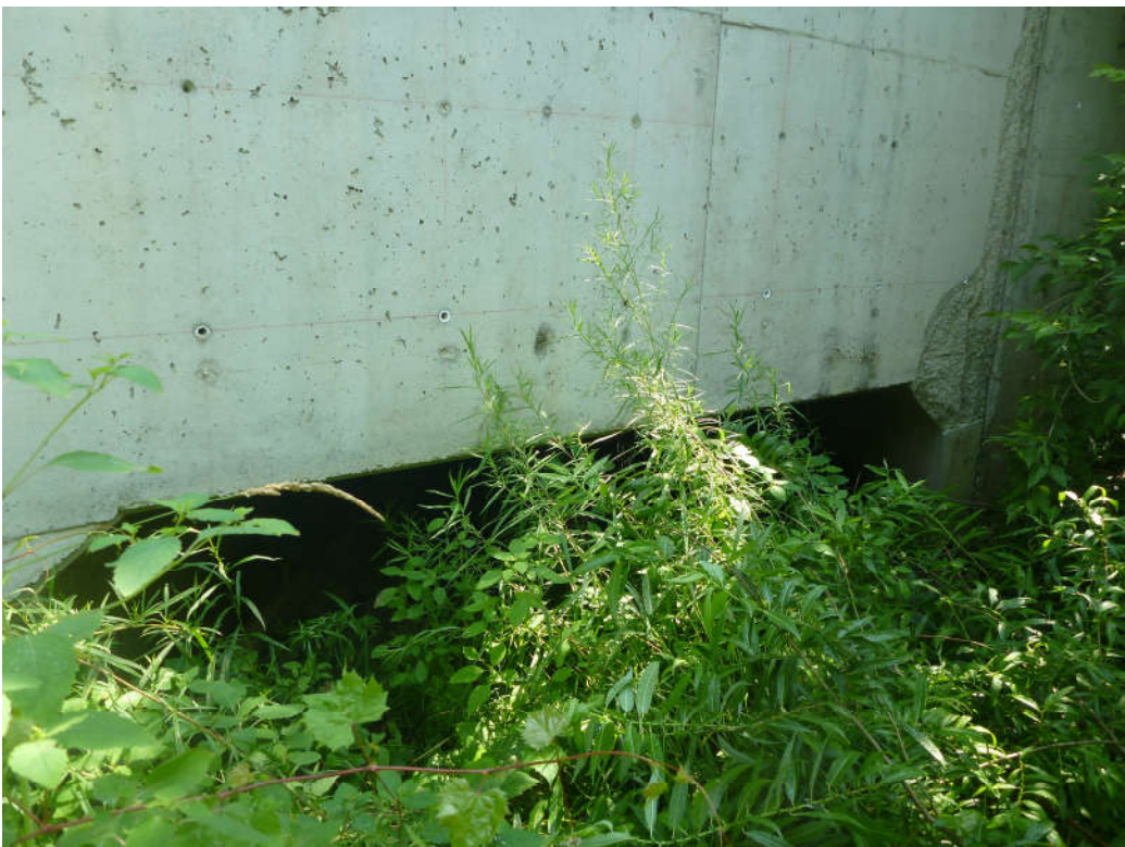
Photo 14 – Vegetation within channel at culvert under Airport Road
