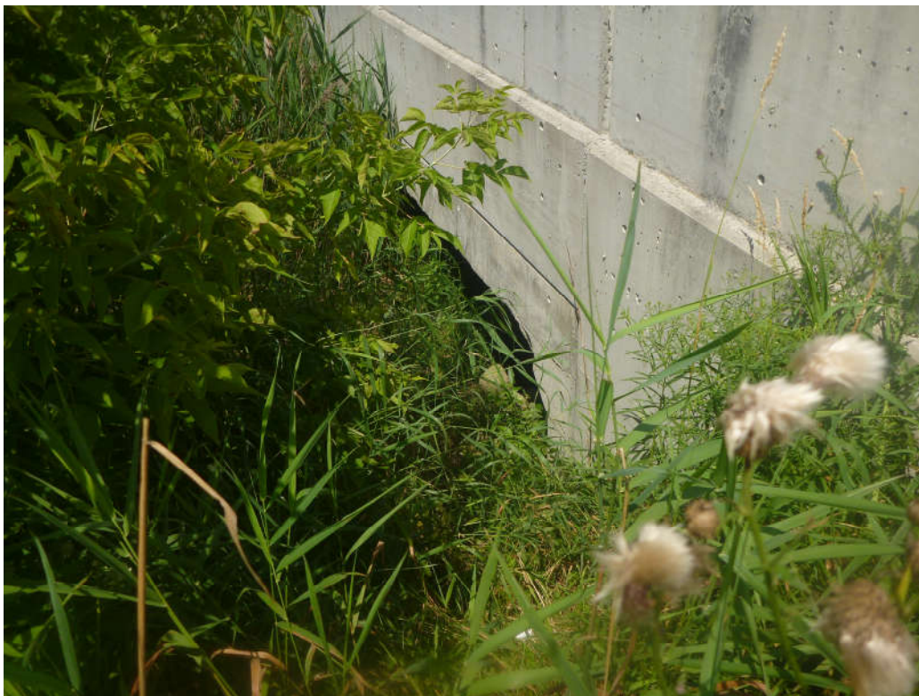
Photo 4 – Vegetation within channel at culvert under Airport Road
