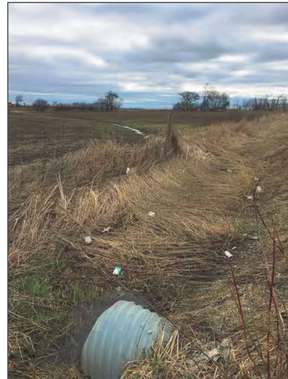
Crossing 5: HUM5-B (roadside ditch on east side of Airport Road), looking south
