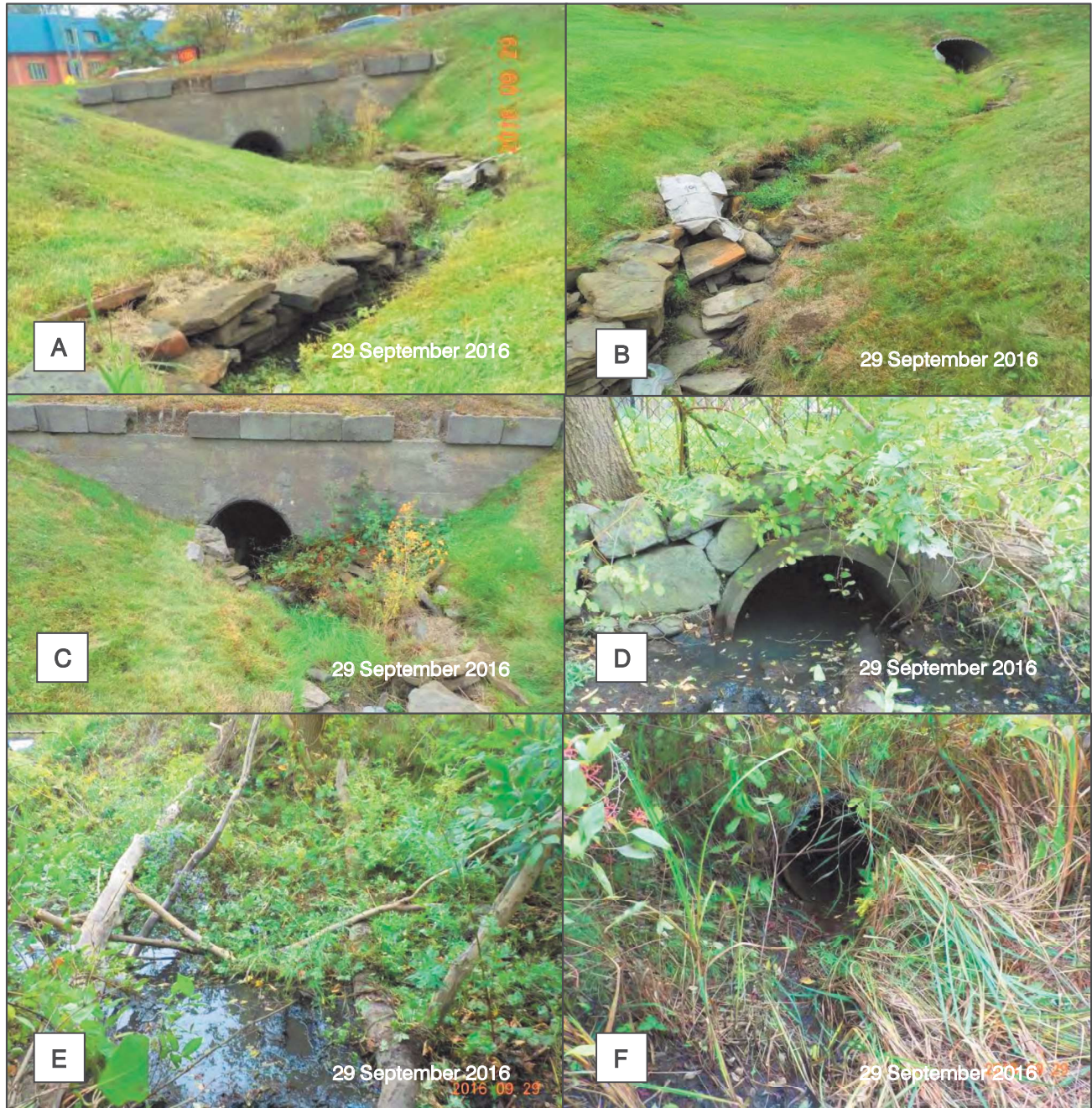
Figure 20. Crossing 2: (A) View of upstream end from upstream; (B) View upstream towards the adjacent culvert; (C) View of the upstream culvert opening; (D) View of the downstream culvert opening; (E) View downstream from downstream culvert opening; (F) View of the culvert located downstream of the Crossing 2 culvert.
