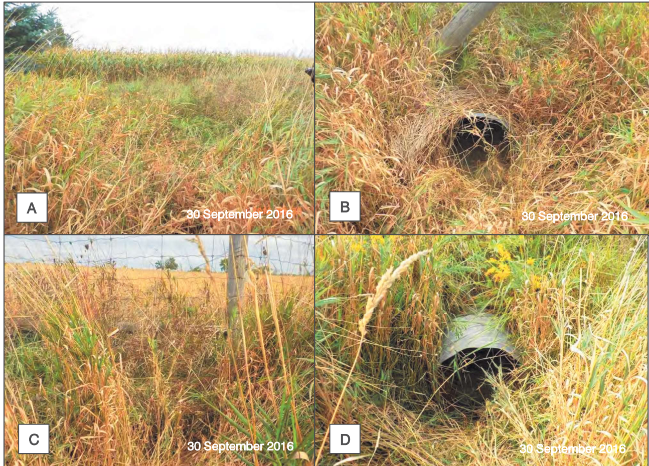
Figure 23. Crossing 5: (A) Looking west from structure; (B) Looking at crossing structure, west side; (C) Looking east from crossing structure; (D) Crossing structure, east side.
