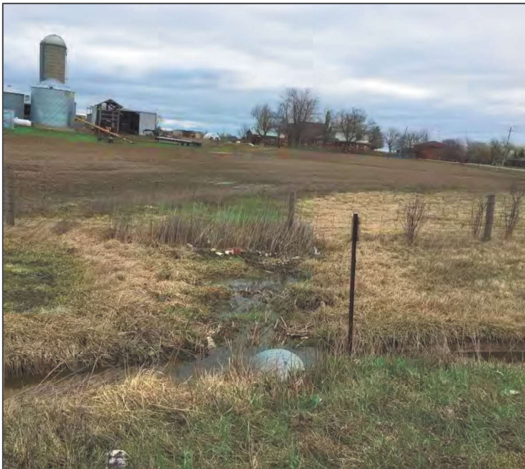
Crossing 6: HUM6-D (swale on east side of Airport Road), or looking south-east from the crossing structure
