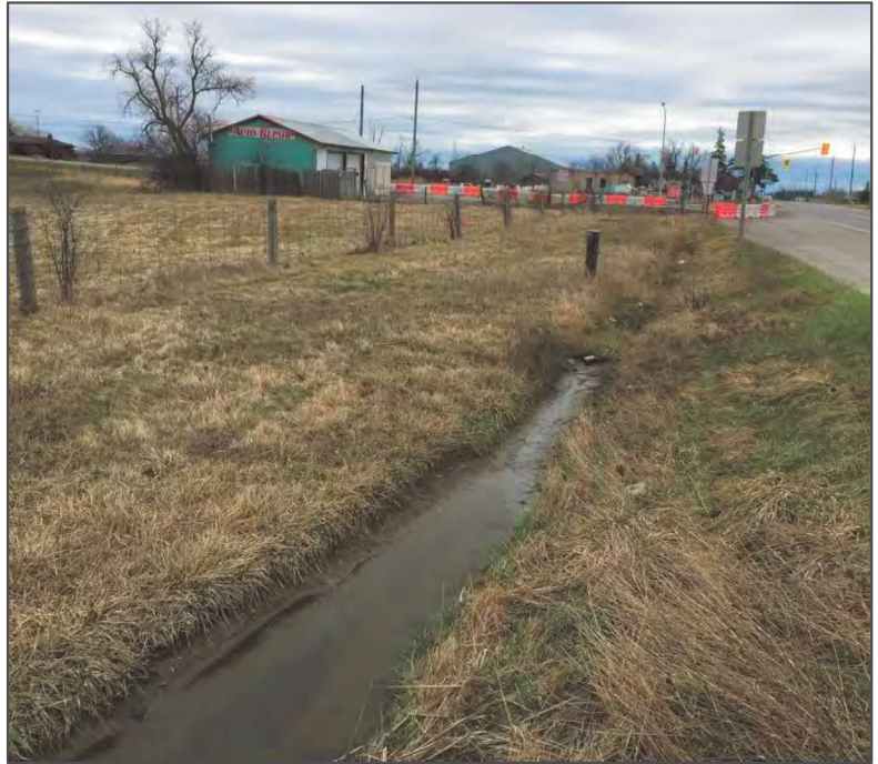
Crossing 6: HUM6-C (roadside ditch on east side of Airport Road), looking south
