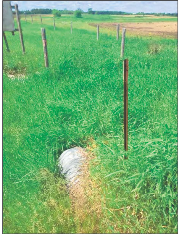
Crossing 6: HUM6-B (undefined feature on west side of Airport Road), looking west from crossing structure
