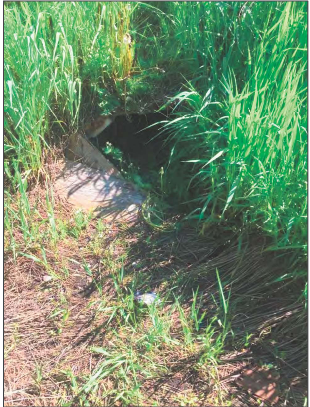
Crossing 4: HUM4-A (roadside ditch on west side of Airport Road), looking at the crossing structure
