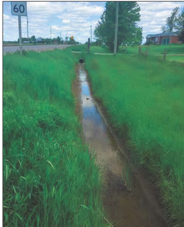
Crossing 6: HUM6-C (roadside ditch on east side of Airport Road), looking north from crossing structure
