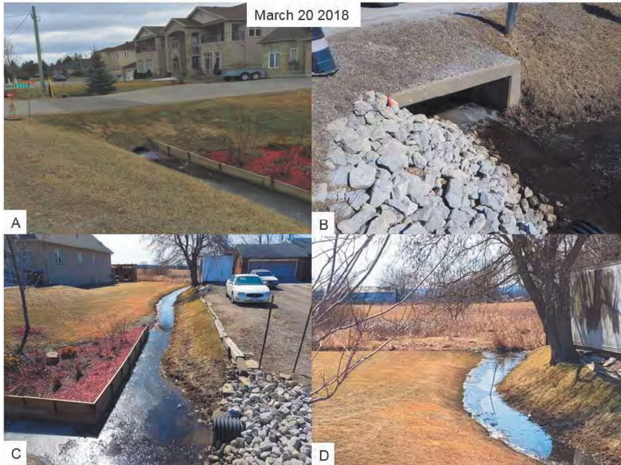
Figure 16b: Crossing 7: (A) Looking upstream towards Airport Road where the watercourse crosses underneath the road. (B) Box culvert at Airport road water flowing southwest. (C) Standing on top of box culvert looking downstream in the southwest direction. Watercourse is flowing through private residential property (D) View of wetland on private property downstream of box culver
