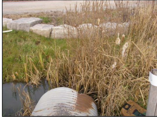
Site 16 facing upstream (north) of Mayfield Road at roadside ditch and armourstone retaining wall: note watercourse flows from right side of photo
