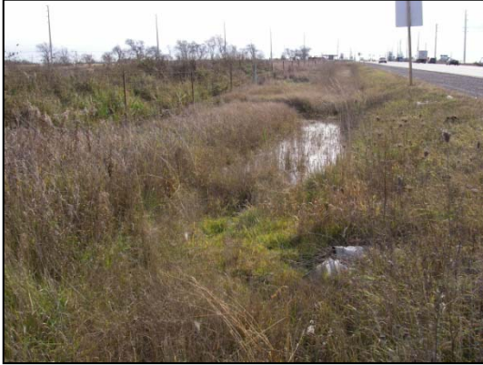
Site 8 downstream (east) of Highway 50 facing south along right-of-way at pooled area downstream of culvert: note berm just outside of right-of-way on left side of photo
