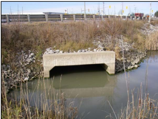
Site 12 facing northwest at downstream end of culvert under Highway 50 conveying water from Site 11
