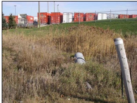
Site 2 downstream (east) of Highway 50 facing east at channel that has been diverted to the north and around the industrial facility
