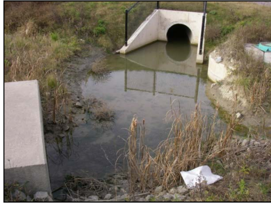
Site 13 facing west at pool upstream of Mayfield Road culvert (left side of photo) and at pipe likely conveying flows from Site 14: note submerged vegetation in foreground of pool
