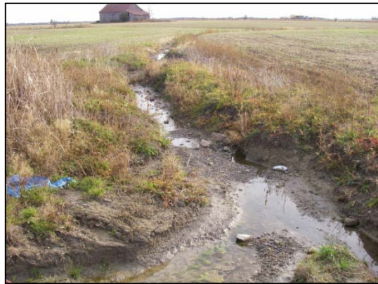
Site 17 downstream (south) of Mayfield Road right-of-way where water from Mayfield Road crossing and storm water outfall join
