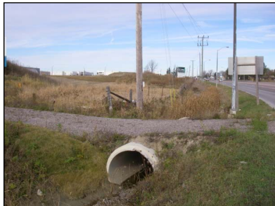
Site 13 facing upstream (north) at new pipe culvert that provides access to new pond that likely receives from Site 14
