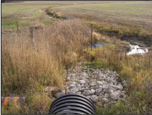
Site 17 downstream (south) of Mayfield Road facing south at right-of-way and channel through agricultural fields
