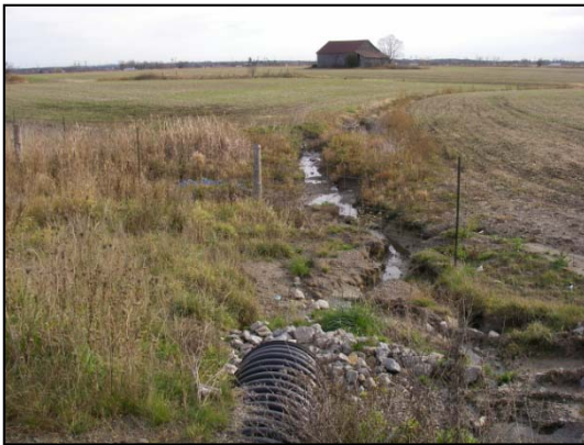
Site 17 facing downstream (southeast) from storm water outfall pipe at Site 17 channel: note water from Mayfield Road culvert enters channel from left of photo
