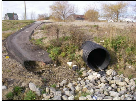
Site 17 storm water outfall and surface drainage chute from Mayfield Road located to south of roadway just west of the Site 17 crossing
