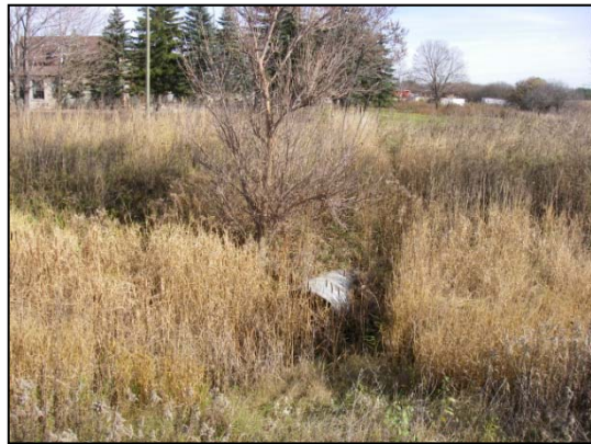
Site 4 downstream end of channel from Highway 50 culvert facing east at CSP through berm
