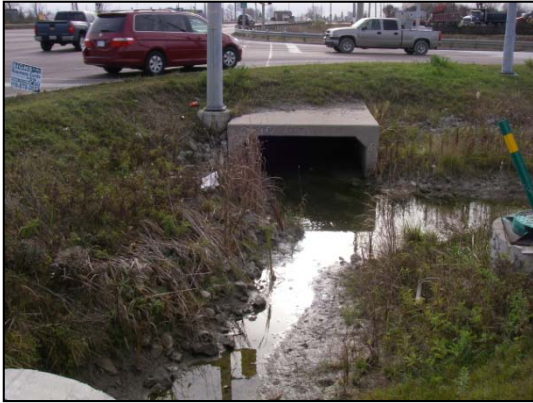
Site 13 facing downstream (south) from new pipe culvert at upstream end of Mayfield Road culvert: note water to right of culvert likely from Site 14
