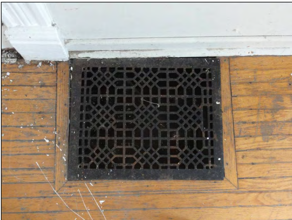
Plate 38: Decorative heating grill in floor of the den.
