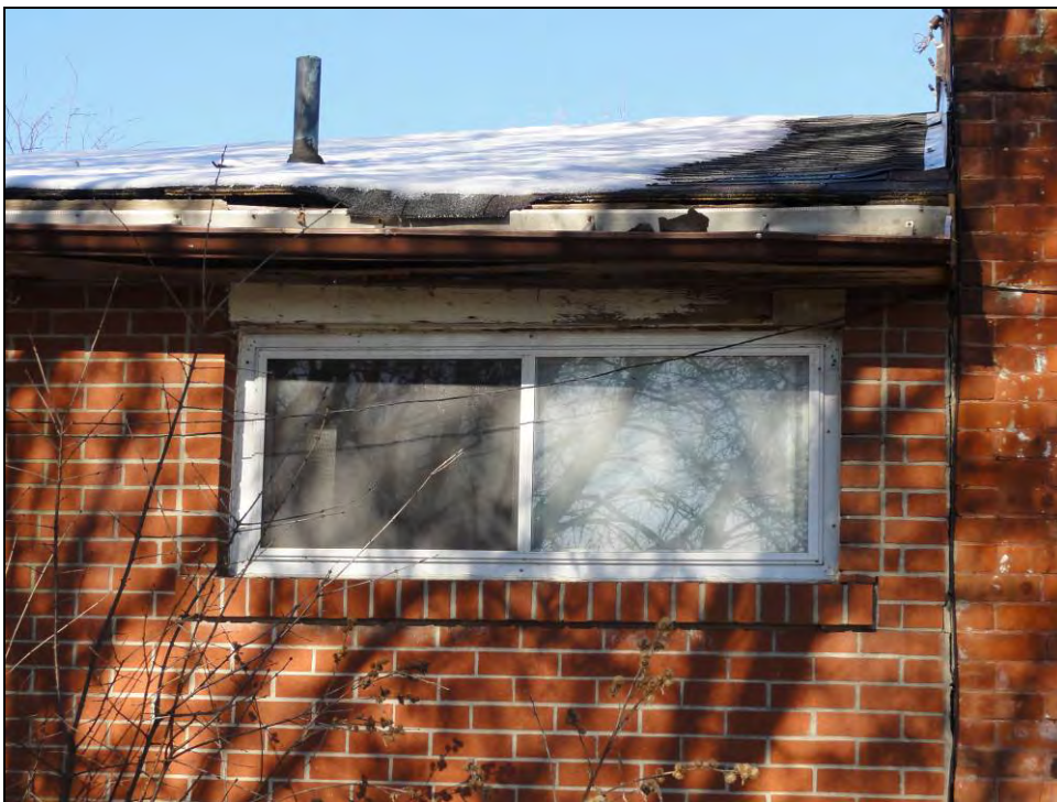
Plate 16: View of modern, side-sliding sash window in c.1960s rear accretion. Note the change in brickwork between front and back sections of the house.
