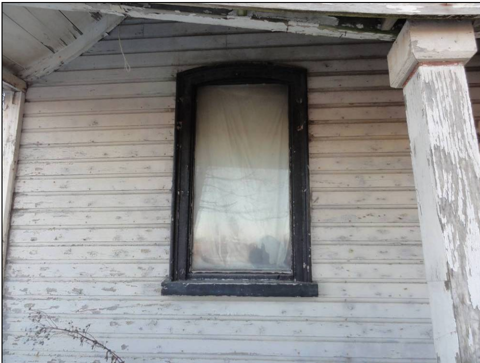
Plate 18: Representative photograph of window opening with modern glass and original decorative casing.
