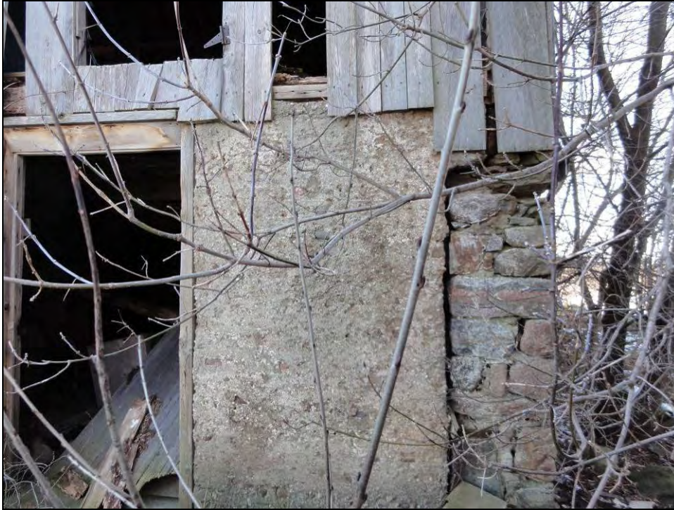
Plate 57: East elevation of barn, north corner, showing stone and poured concrete foundations.
