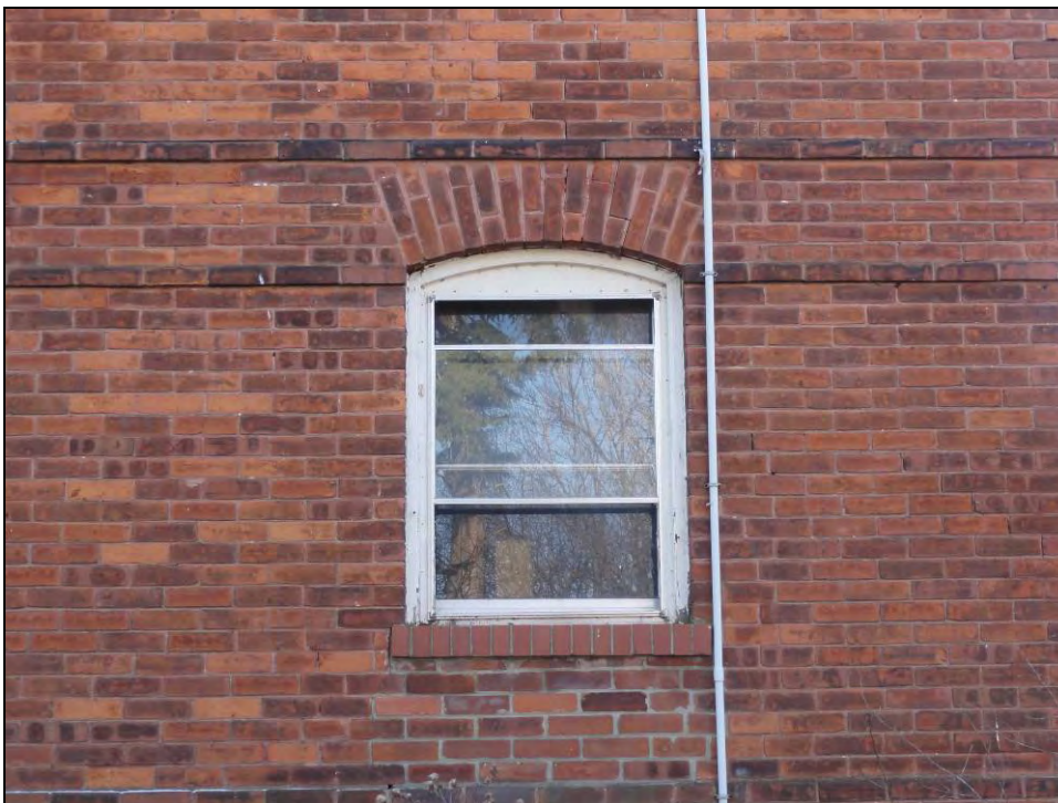
Plate 14: Slightly smaller window opening located on main floor of the north elevation.
