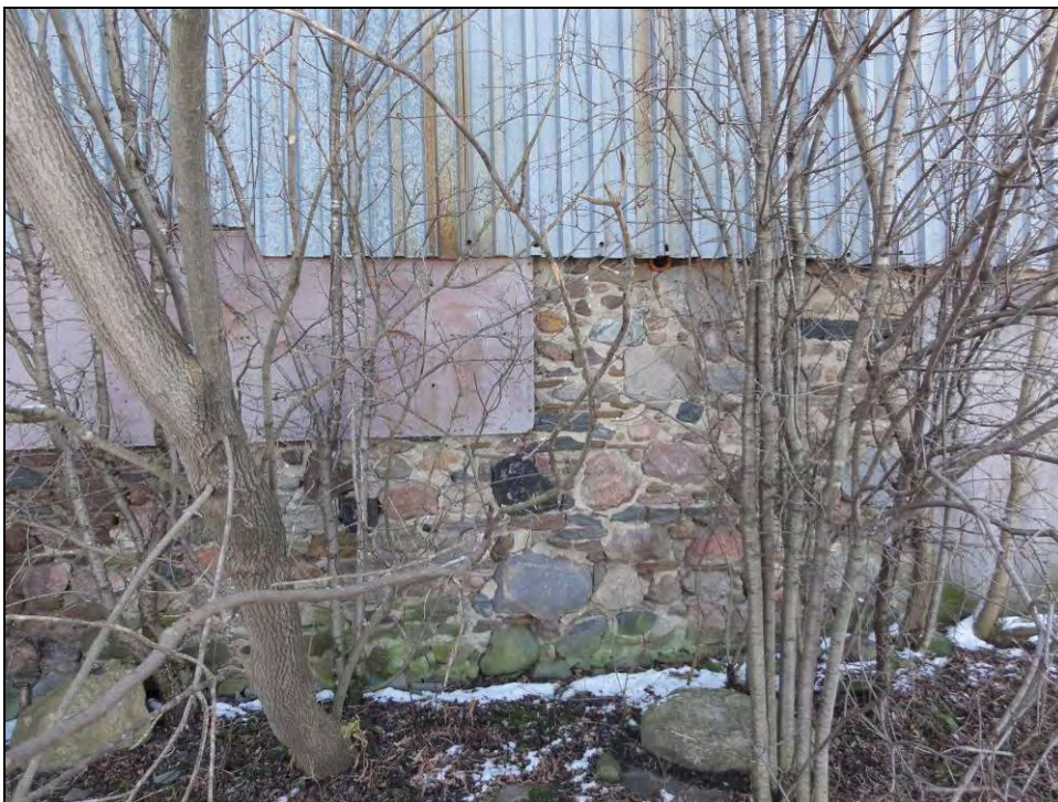
Plate 58: Detail of stone foundations on the north elevation, and blocked up windows.
