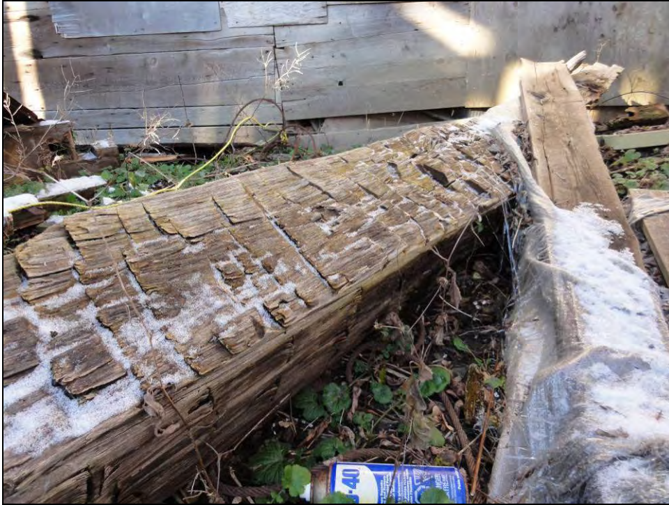
Plate 63: Detail of hewn structural beams that have collapsed.
