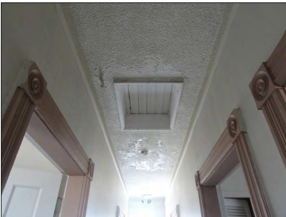
Plate 32: Access to the attic. Note the decorative casing around the doorways to Bedrooms No. 1 and 2, and the Bathroom.
