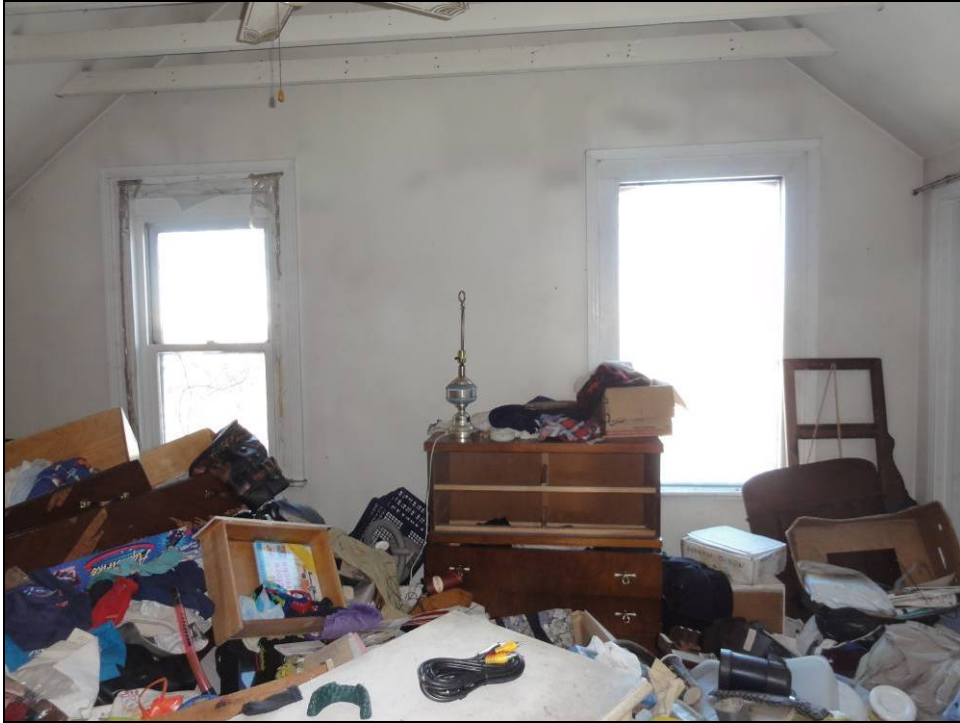
Plate 31: View of the bedroom located on the north side of the house.
