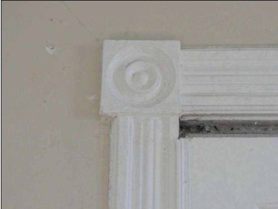
Plate 47: Bullseye rosette block at corner of front door casing in the den.
