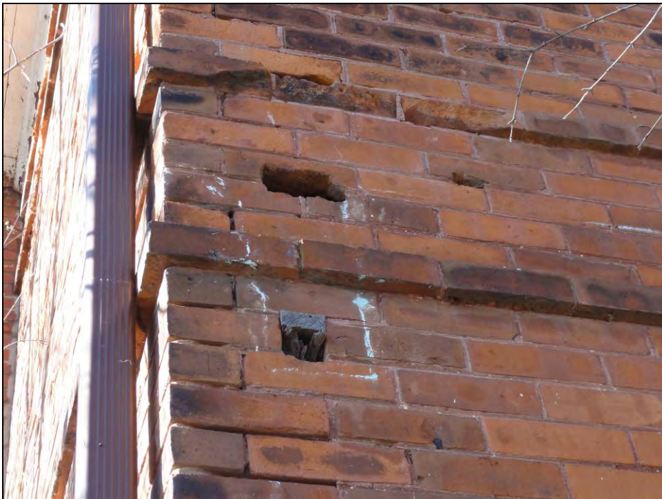
Plate 10: South corner of front elevation, showing remnants of wooden frame porch in exterior brickwork.
