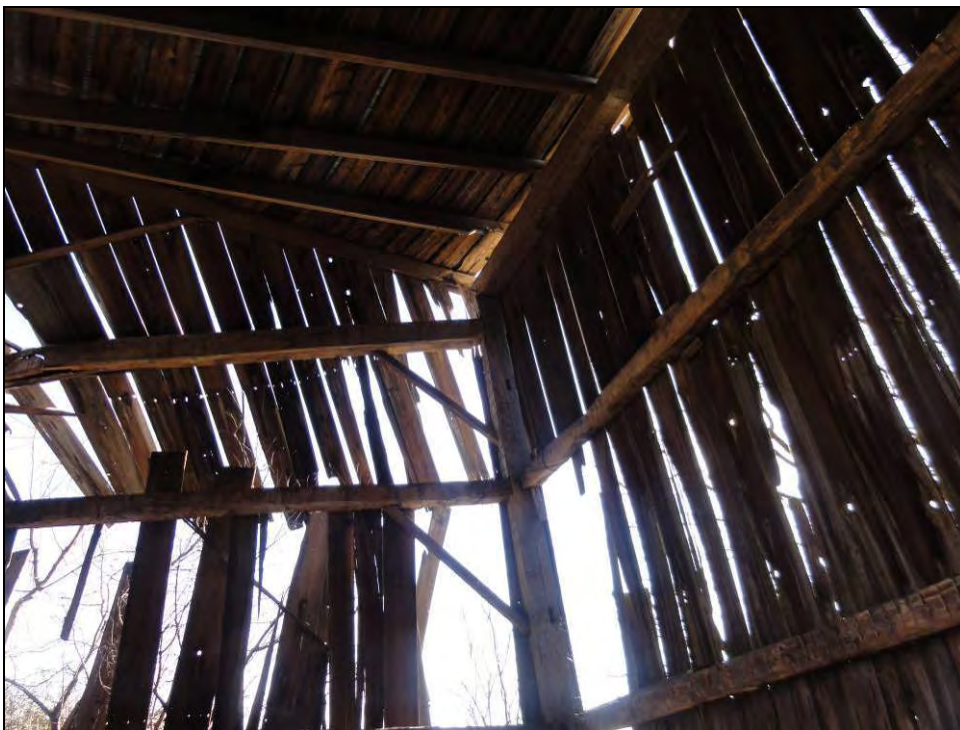
Plate 60: View of southwest corner of collapsed portion of barn.
