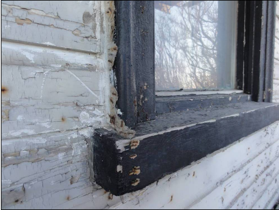
Plate 21: Detail of wooden sill.
