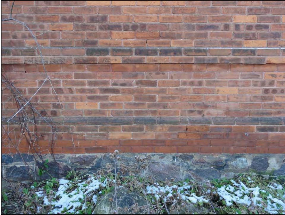
Plate 7: Detail of stone foundations, bands of projecting brick, and brick drip course above the foundations.
