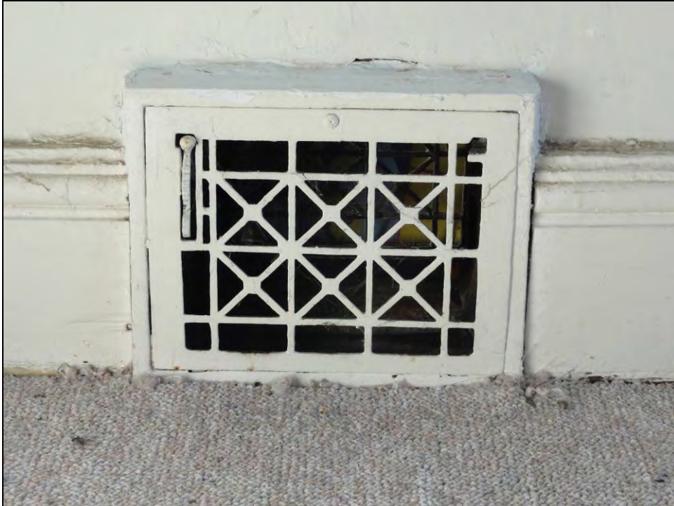
Plate 49: Note the heating grill in base of the wall and high, molded baseboards, located in Bedroom No.3.
