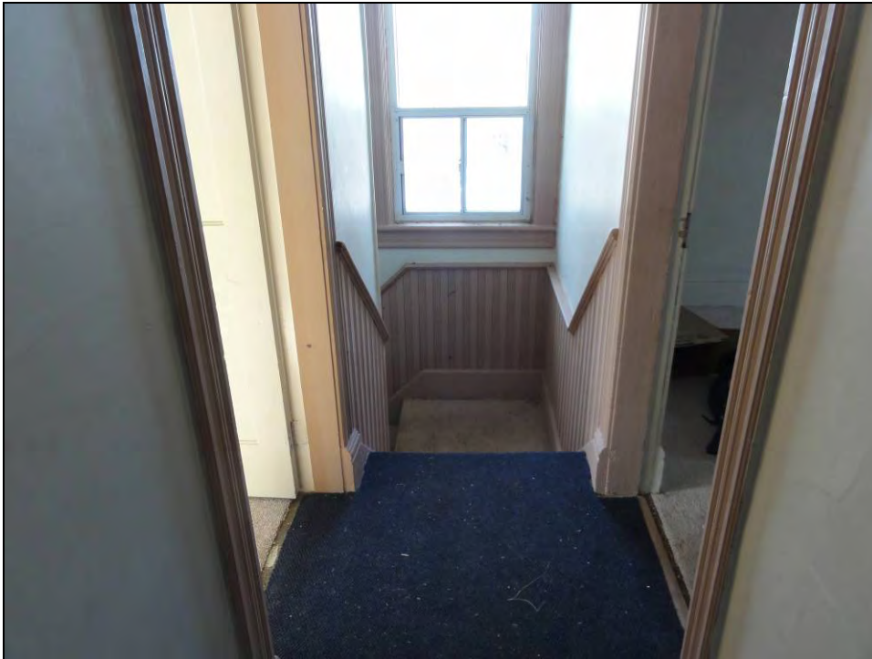
Plate 31: View of L-shaped stairwell from main floor to second floor, looking west.
