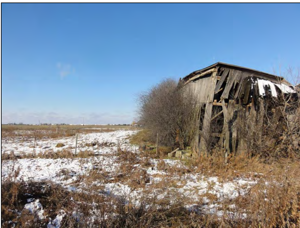
Plate 54: South elevation of barn (partially collapsed).
