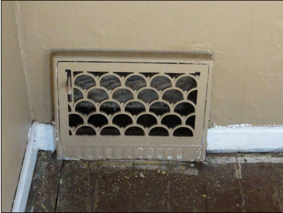
Plate 37: Decorative heating grill in the parlour. Note the simple, modern baseboards.
