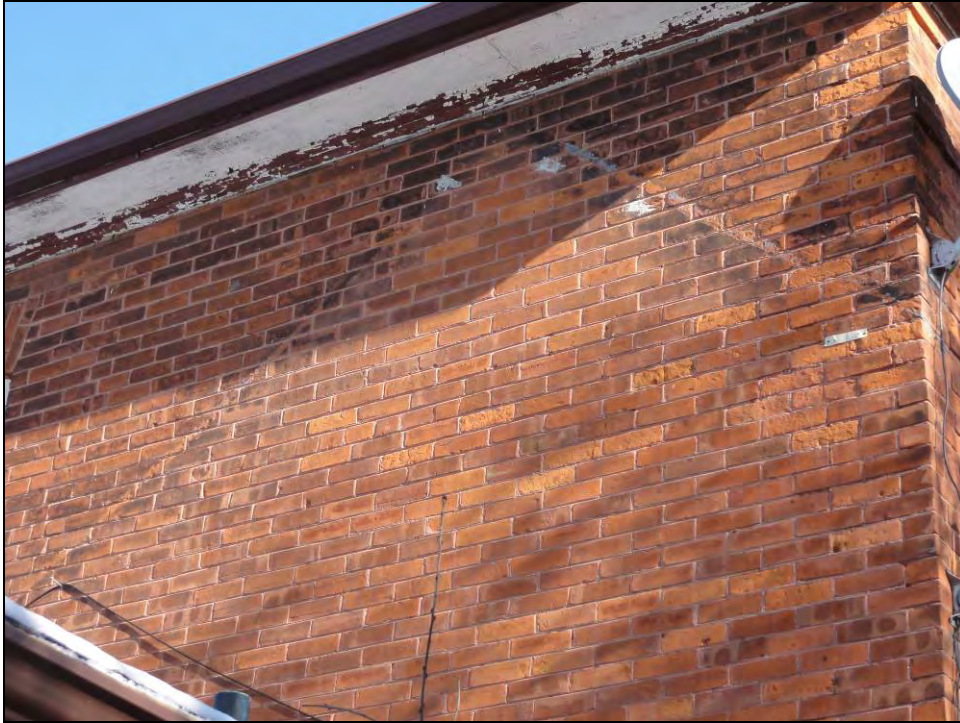
Plate 17: View of gable-roofed profile of original rear accretion on west elevation of the house.
