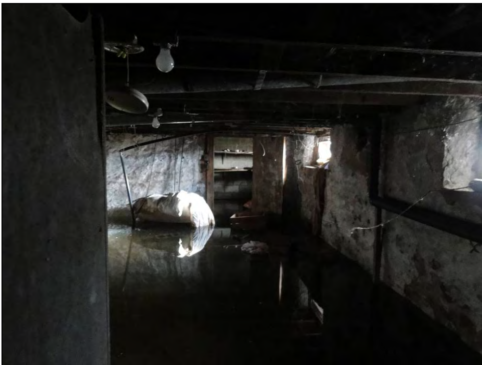
Plate 18: View of basement from the stairs, looking east. Note the entrance at the far wall into a cold cellar under the front porch.
