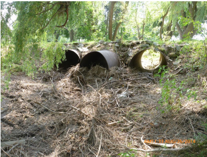
Photograph 3. ↑ Debris accumulation of outlet of private crossing upstream of the Gore Road in Reach 2.
