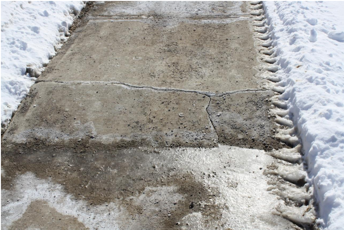
Figure A31 — Uneven Sidewalk Surface (Tripping Hazard) – Section between Ebenezer Road and Fogal Road
