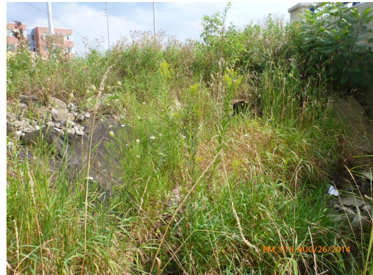
↑ Failed placed stone, erosion blanket, and inactive CSP outfall on US LB
