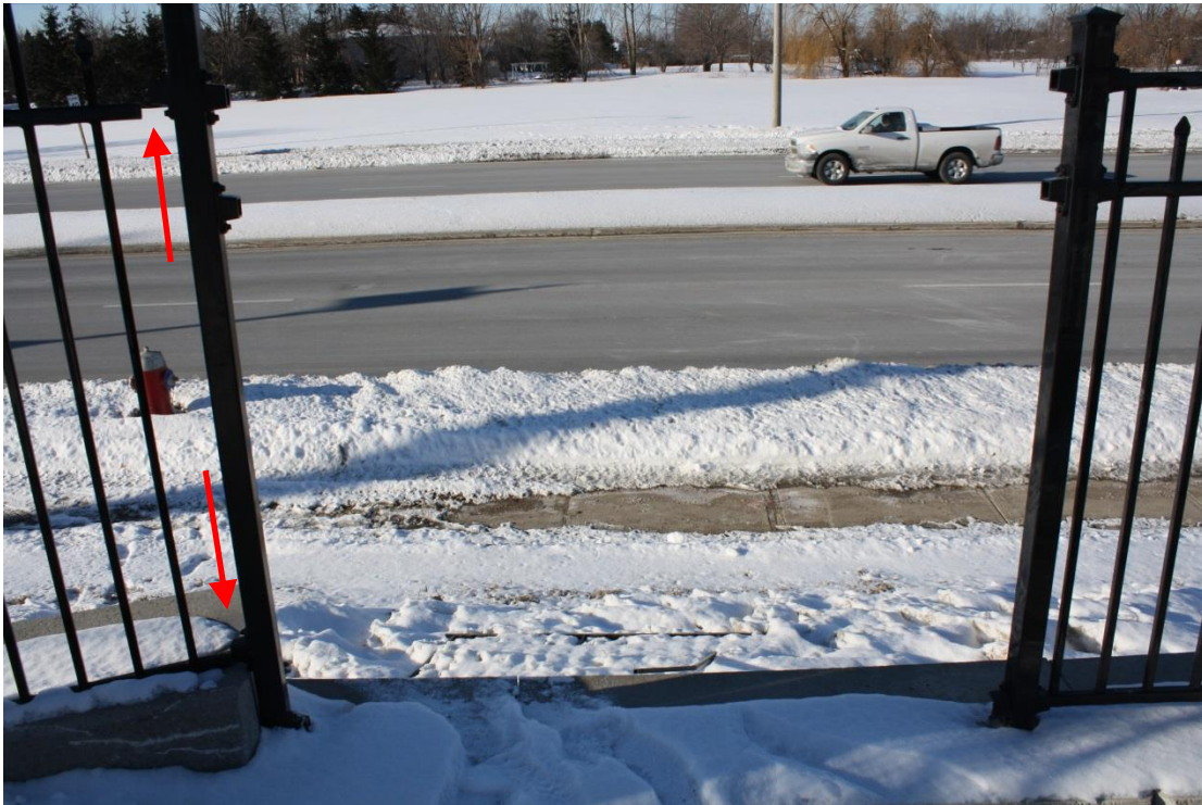
Figure A12 – Broken Fence and Missing Fence Section on Pedestrian Ramp from Newington Crescent to The Gore Road
