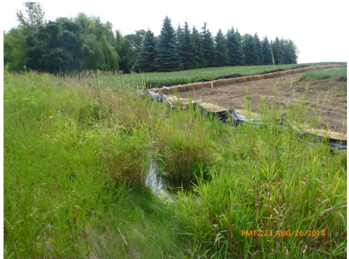
Photograph 4. ↑ Looking downstream in the recently realigned portion of the channel between the Gore Road and Castlemore Road in Reach 2. Note the construction on the right bank.
