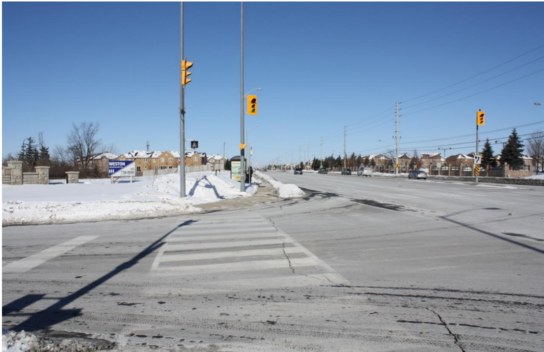
Figure A29 — No Pedestrian Count-Down Signal and Worn CROSSWALK Markings - Intersection of The Gore Road and Don Minaker Drive / Tyler Avenue
