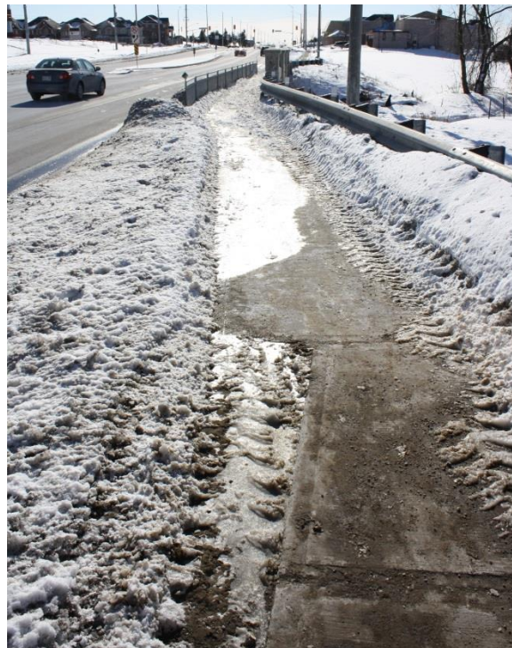
Figure A17 – Uneven Sidewalk Edge – Section between Castle Oaks Crossing and Gardenbrooke Trail / Pannahill Drive
