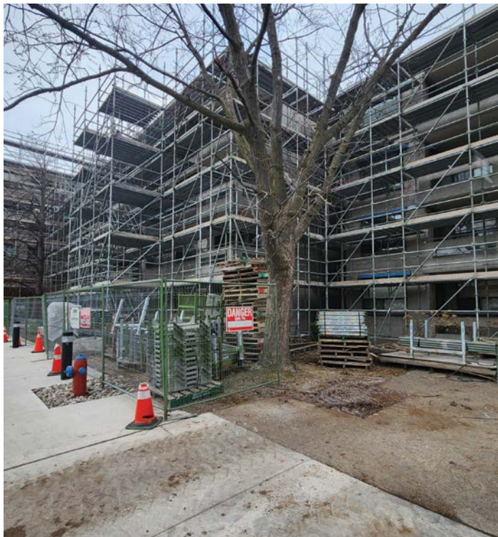
Hillside Place is a seniors' residential building that is part of a community energy project funded by the CCBF that will see the current natural gas heating system replaced with an energy-friendly heat pump system, providing both heat and air conditioning to the building.
