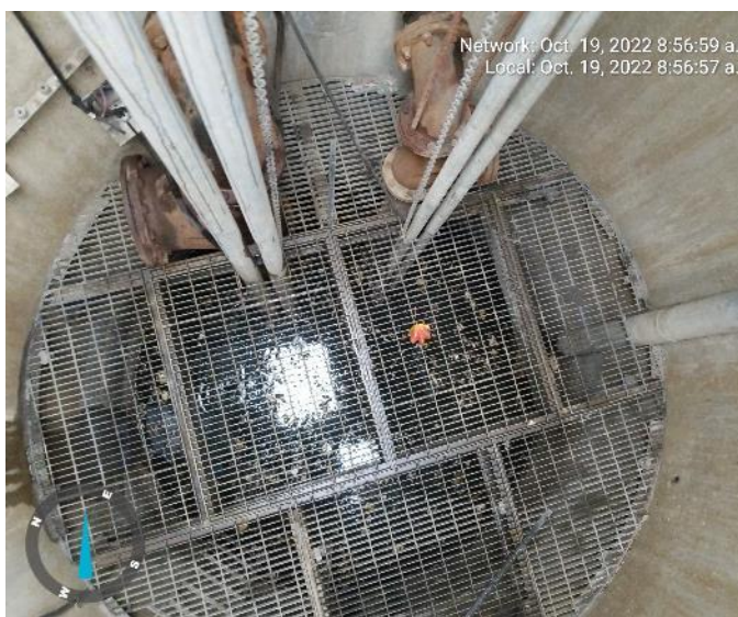
Photograph 6: Interior view of Finch SPS wet well from top hatch, facing down.
