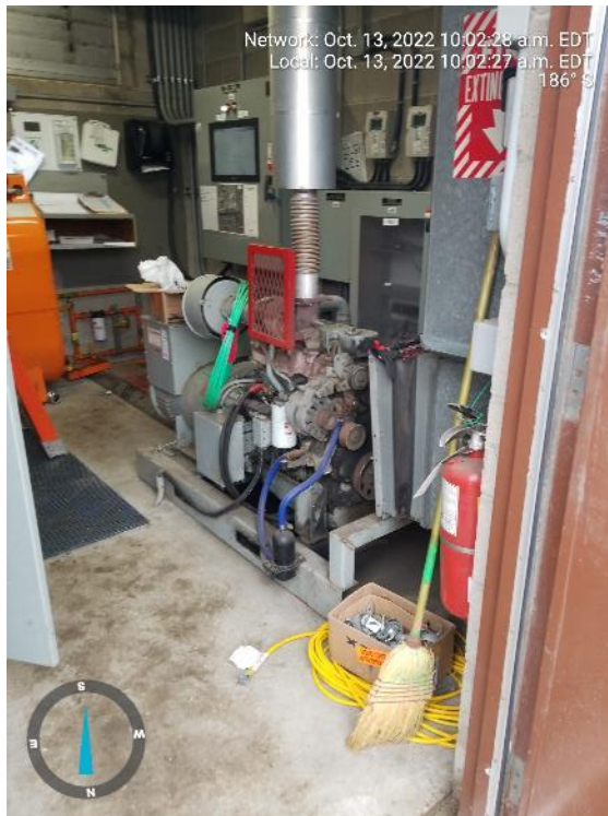
Photograph 4: Interior view of Finch SPS control building from front door facing south.
