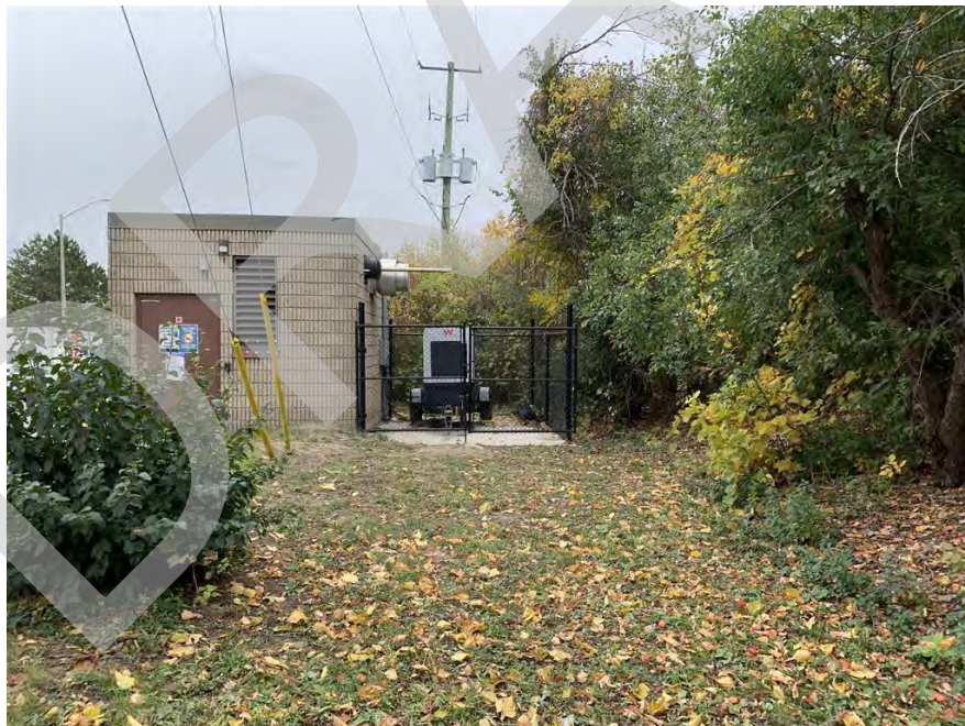
Image 4: View of current pumping station along west side of Finch Avenue West, within Proposed Design Alternative A, facing south. 20 October 2022
