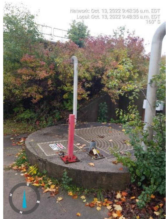
Photograph 5: Exterior view of Finch SPS wet well and CN Rail (back) from west of Finch Avenue West, facing south.
