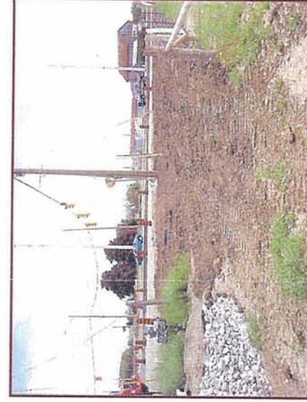
Figure 11-3: Disturbed Northwest Corner of the Intersection of Dixie Road and Mayfield Road (looking southwest)
