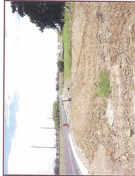
Figure 11-4: New Construction in Southwest Corner of the Intersection of Dixie Road and Mayfield Road (looking southwest)
