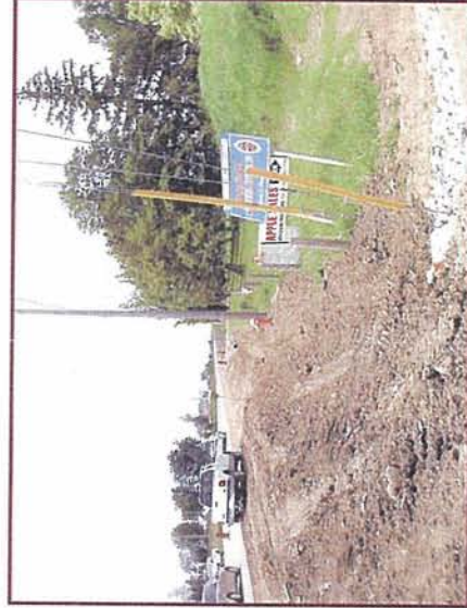
Figure 11-2: Disturbed Area at Northeast Corner of Intersection of Dixie Road and Mayfield Road (looking northeast)
