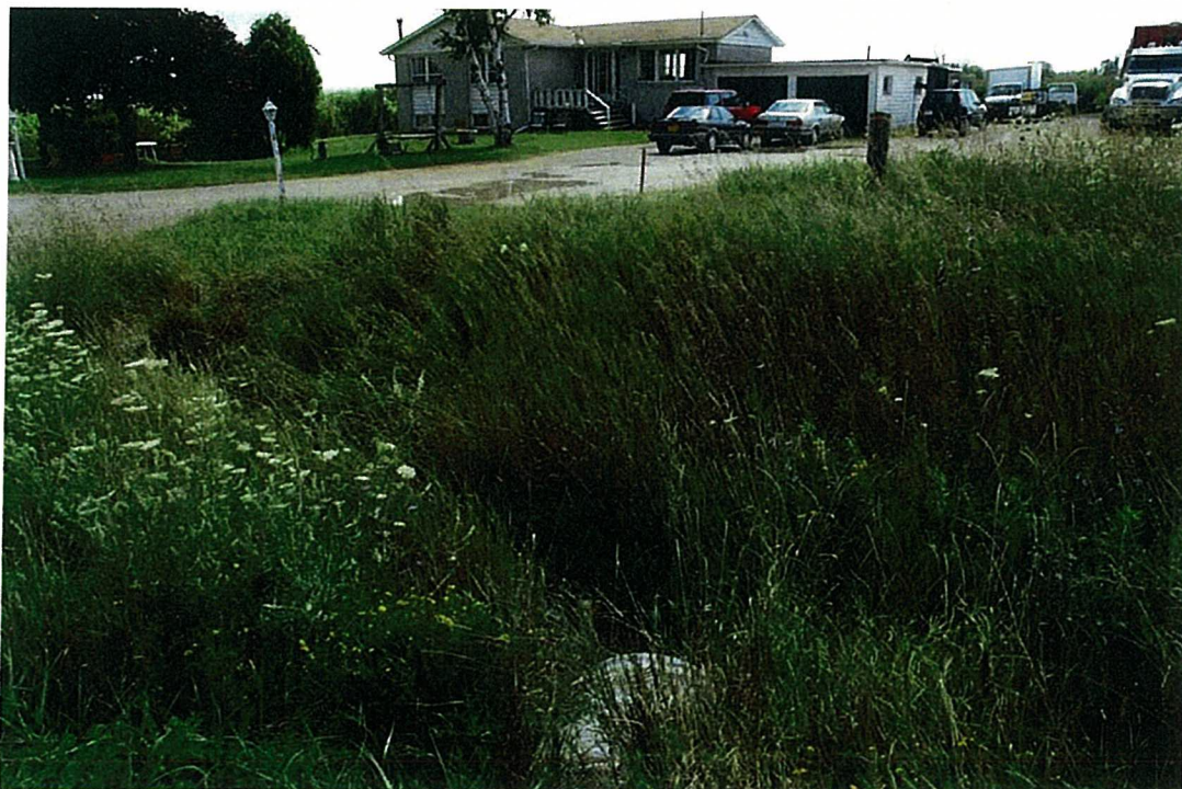
A 0.6 m diameter CSP crosses under Dixie Road south of Mayfield Road conveying a headwater tributary of Etobicoke Creek to the southeast
