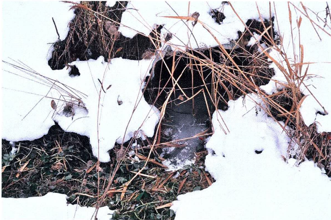
The culvert inlet at the northeast quadrant of Mayfield/Dixie is almost obscured by vegetation
