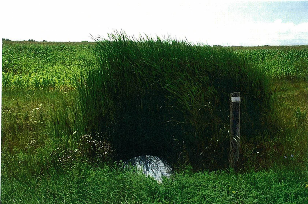
Another Etobicoke Creek tributary crosses Dixie Road north of Countryside Drive via a 1.8 m diameter CSP
