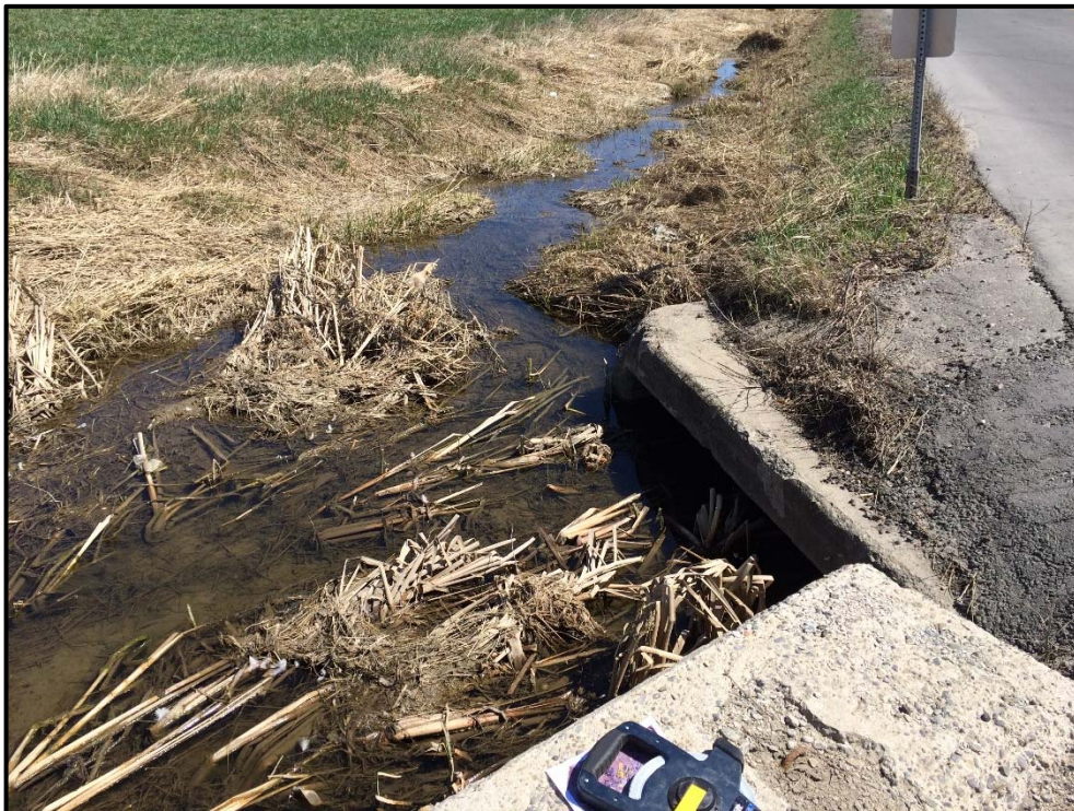
Photo 6: Downstream end of Crossing RB3. Agricultural drainage ditch passes under roadway through box culvert.
