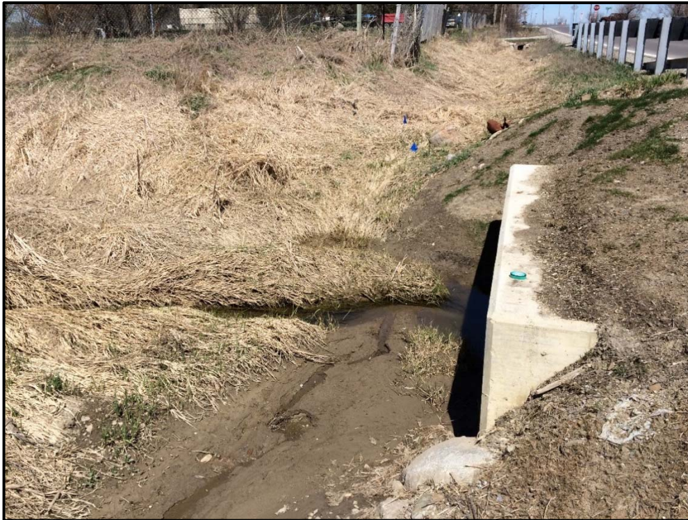
Photo 9: Upstream end of Crossing RB2. Note ditch drainage outletting from the west of the watercourse.
