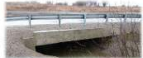
Clarkway Drive over Clarkway Tributary
