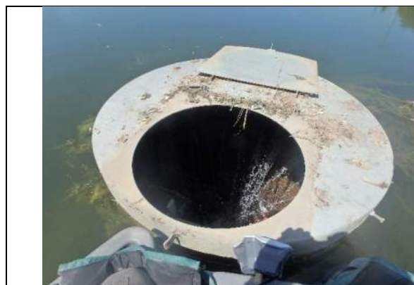
Photo 1: The top of the riser pipe with the flap open.
