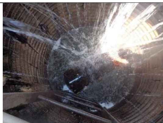
Photo 2: View inside the riser with the slotted outlet pipe at the bottom.
