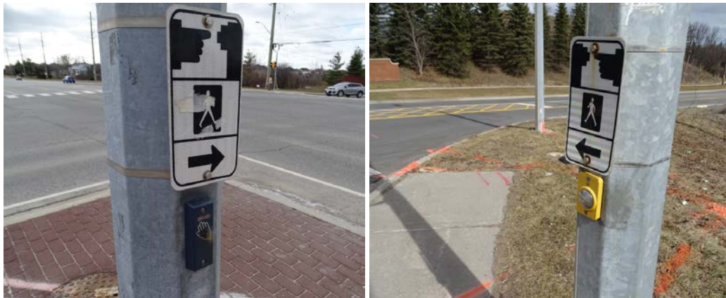
Figure 19 – Pedestrian Pushbutton Not Fully Accessible
