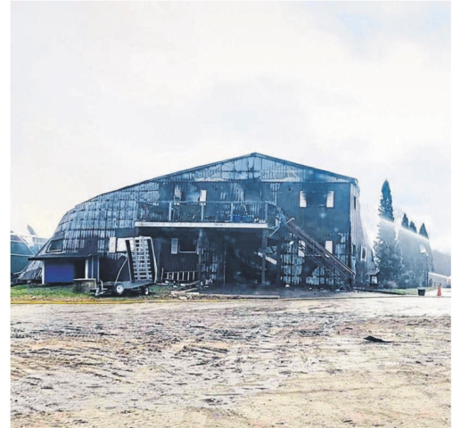
Caledon OPP photo Caledon OPP and Caledon Fire and Emergency Services were called to a barn fire on Saturday, Nov. 27.
