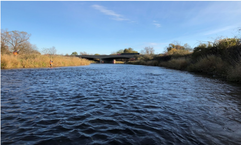
Photograph 10: Reach CR-1; view downstream approaching bridge at Highway 401; right bank has steepened.
