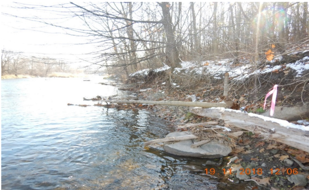
Photograph 14: Reach CR-2; vertical right bank with exposed tree roots and leaning trees as well as washed up woody debris.
