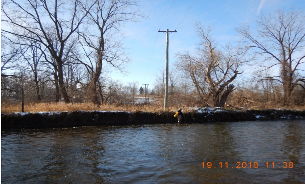
Photograph 19: Reach CR-2; vertical right bank in response to channel widening; right bank has been eroded back to the hydro line.
