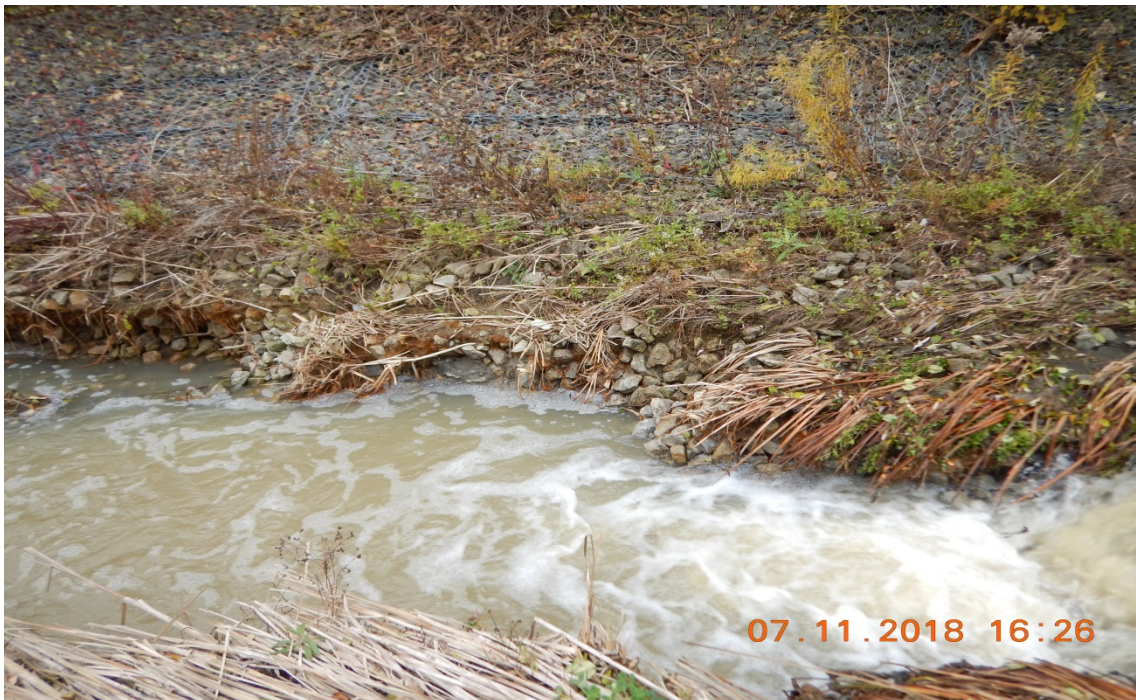
Photograph 8: Reach MC-1; eroded banks downstream of knickpoint due to high flow velocity.
