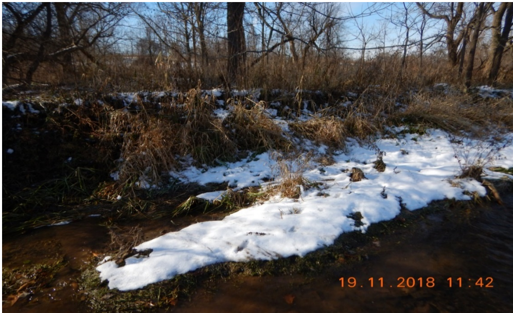
Photograph 18: Reach CR-2; slumping along right bank.
