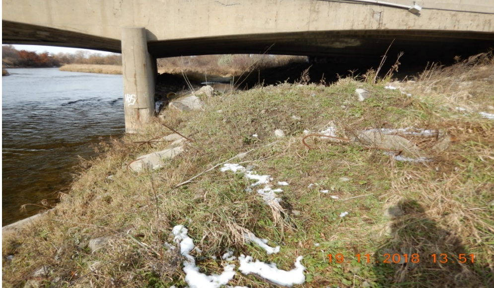
Photograph 13: Reach CR-2 (Credit River downstream of Highway 401); large concrete boulders and exposed rusted rebar along right bank.
