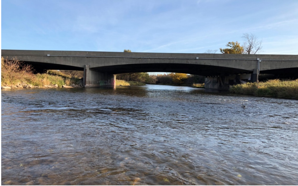
Photograph 11: Reach CR-1; bridge crossing at Highway 401 representing reach break between CR-1 and CR-2; note concrete slabs that have washed up along the left bank.
