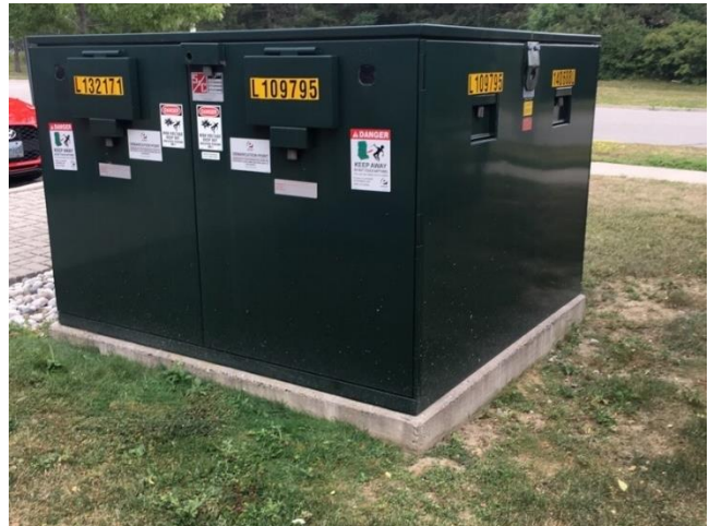
Photo 34: Evidence of buried utilities in Area 6.2; view northwest
