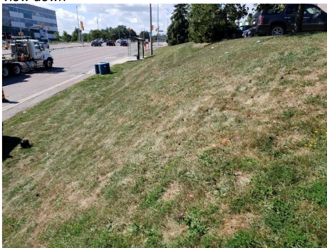
Photo 27: Severe slope and disturbance within Area 5.3 west of Derry Road; view south
