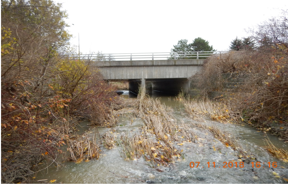
Photograph 11: Reach MC-1; view downstream at bridge crossing with Century Avenue; stacked gabion baskets line banks on either side of the bridge.
