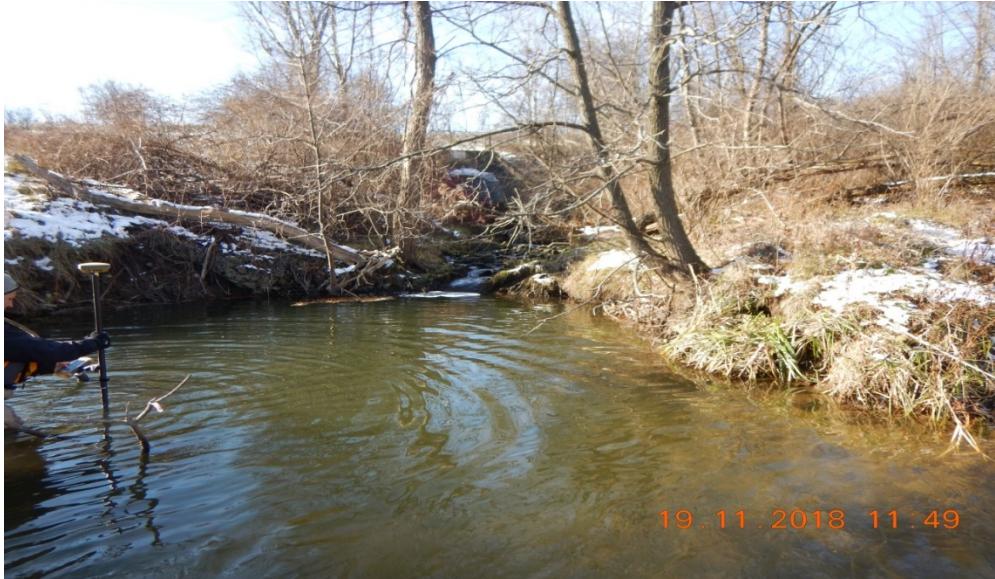
Photograph 15: Reach CR-2; large scour pool ~0.8 m deep downstream of a stormwater outfall with a water dissipation pad; gabion baskets along right bank have started to fail and banks have become undercut 10 to 20 cm.
