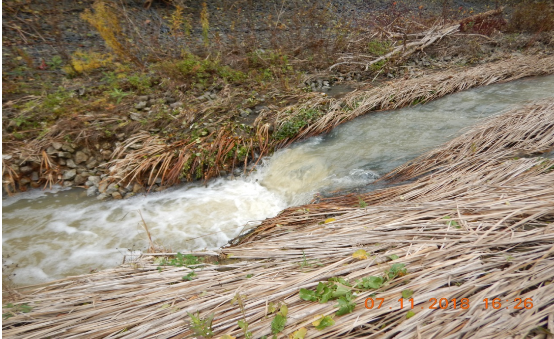
Photograph 7: Reach MC-1; scour pool downstream of a knickpoint with a bankfull depth of ~1.1 m; gabion baskets lining channel banks.
