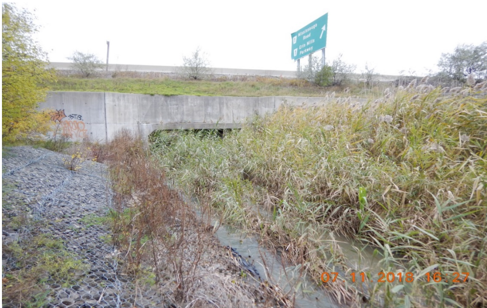
Photograph 6: Reach MC-1; looking upstream at bridge crossing with Highway 401 (on downstream side of highway); dense growth of in-stream grass; channel banks lined with gabion baskets.
