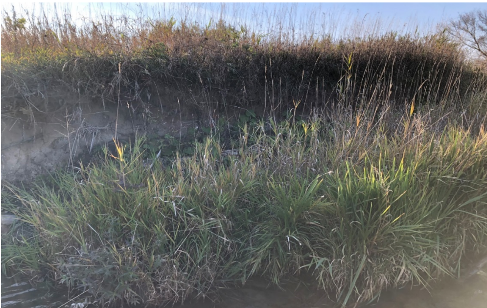
Photograph 8: Reach CR-1; bank slumping along the right side of channel resulting in a vertical bank.
