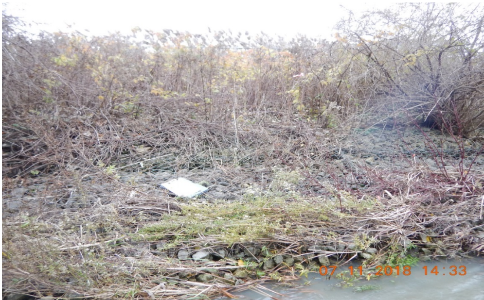
Photograph 2: Reach MC-1; gabion baskets upstream beginning to fail as evidenced by angular boulders along channel bank.
