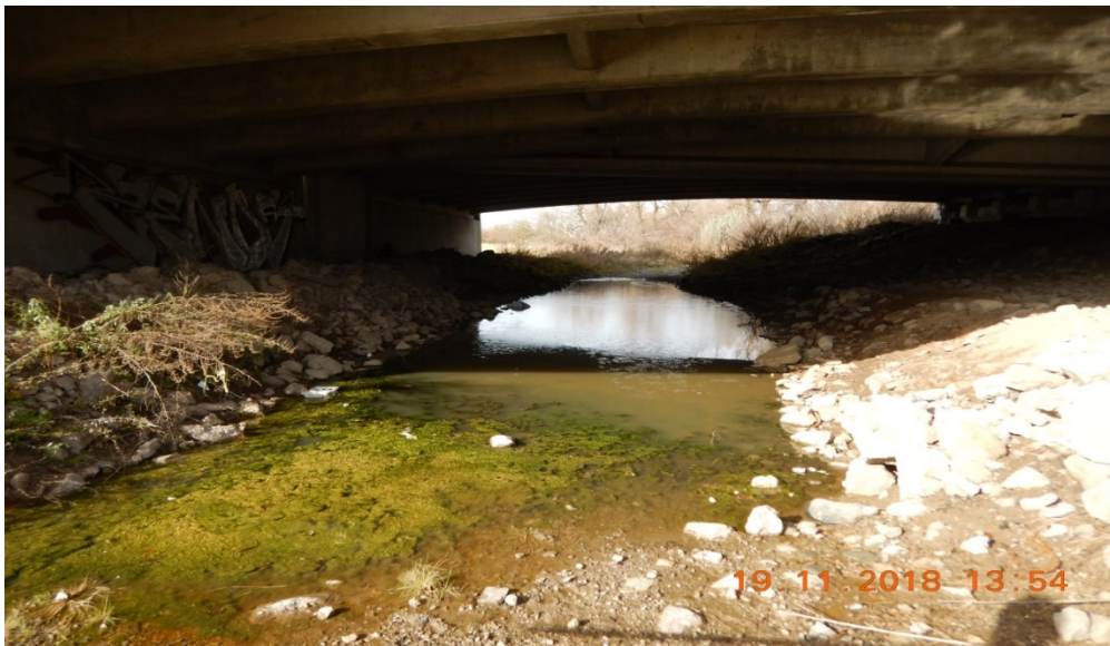
Photograph 12: Credit River under the bridge crossing at Highway 401; algal growth in stagnant water; steep piles of angular boulders embedded in sand bordering the channel.
