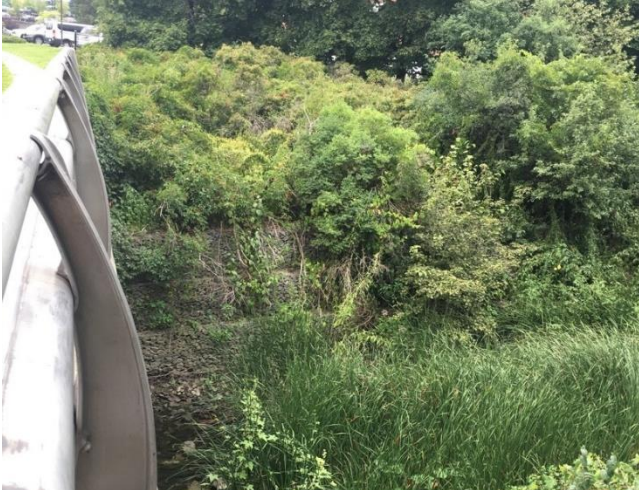
Photo 37: Example of the severe slope found in Area 6.2; view southwest
