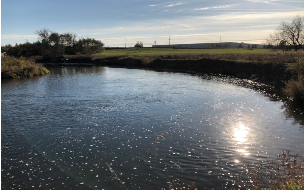
Photograph 5: Reach CR-1; large scour pool ~1.2 m deep (wetted depth); right banks are vertical.
